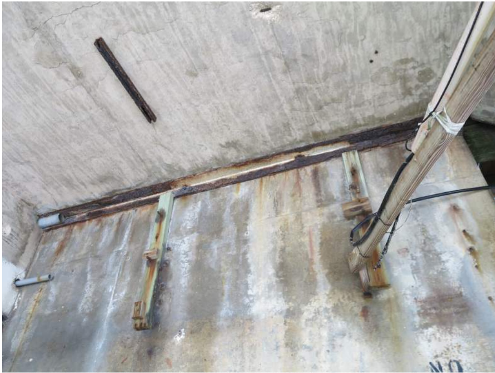
Photo 7 Existing Steel Angle Ledger, Looking Up and North Note Severe Corrosion of Angle on Right Side
