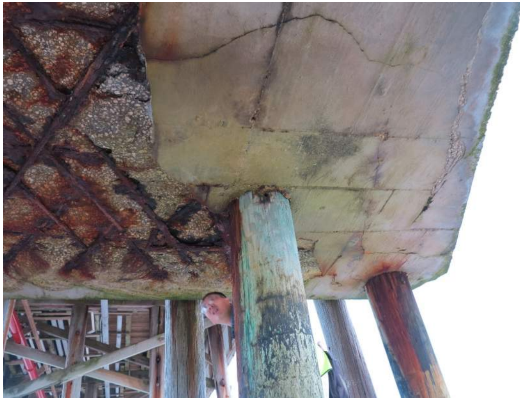
Photo 8 Former Chairlift Concrete Pier Support Between Bents 14 and 15, Looking Up and West Note Spalled and Delaminated Areas with Exposed Steel Reinforcing Bars
