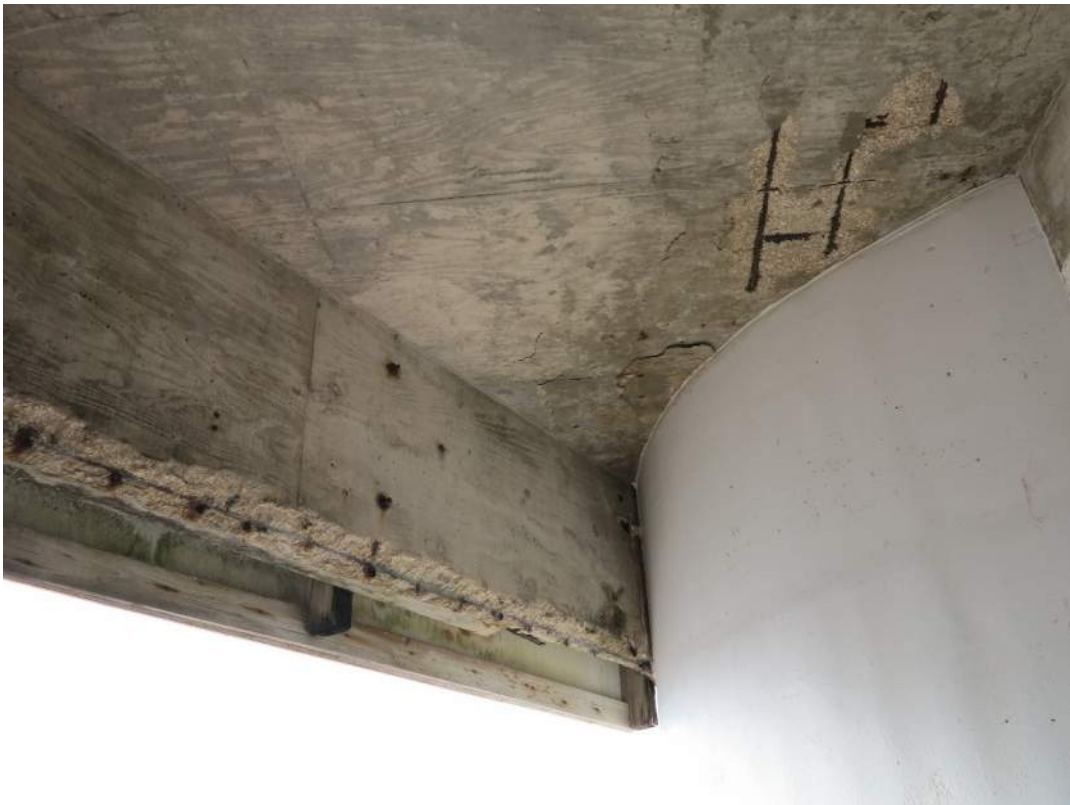
Photo 2 Existing 8"x48" Concrete Beam (Wing), Looking South Note Missing Steel Reinforcing Bar
