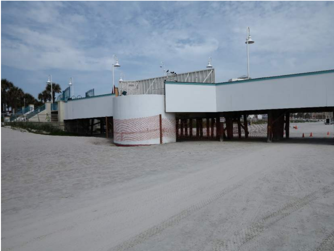
Photo 1 Former Space Needle Cradle/Bowl Concrete Support, Looking Northwest No Deficiencies Were Noted at the Cylindrical Concrete Support
