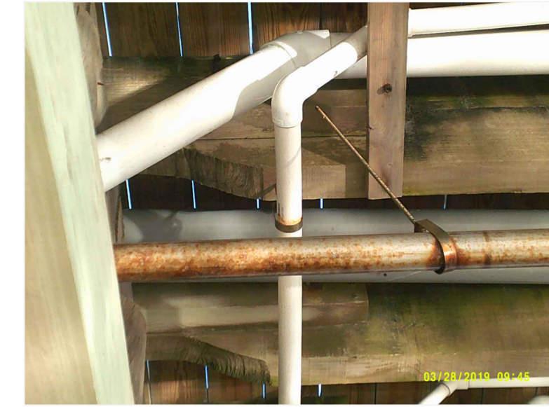
BENT 6: LOOSE GAS LINE HANGER
