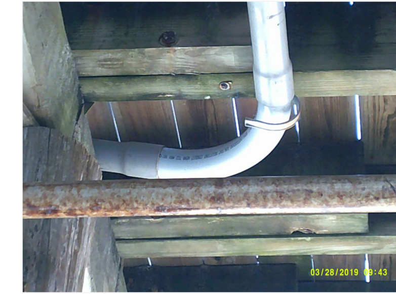
BENT 5: LOOSE ELEC. CONDUIT HANGERS
