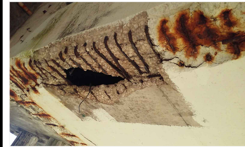
BENT 3-4: CONCRETE SPALL
