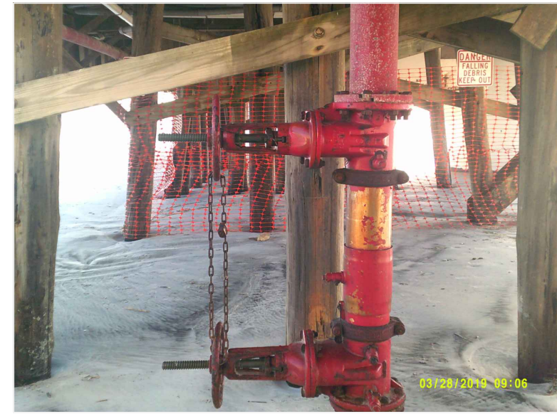
BENT 1: 6" FIRE LINE DOUBLE CHECK VALVE ASSEMBLY
