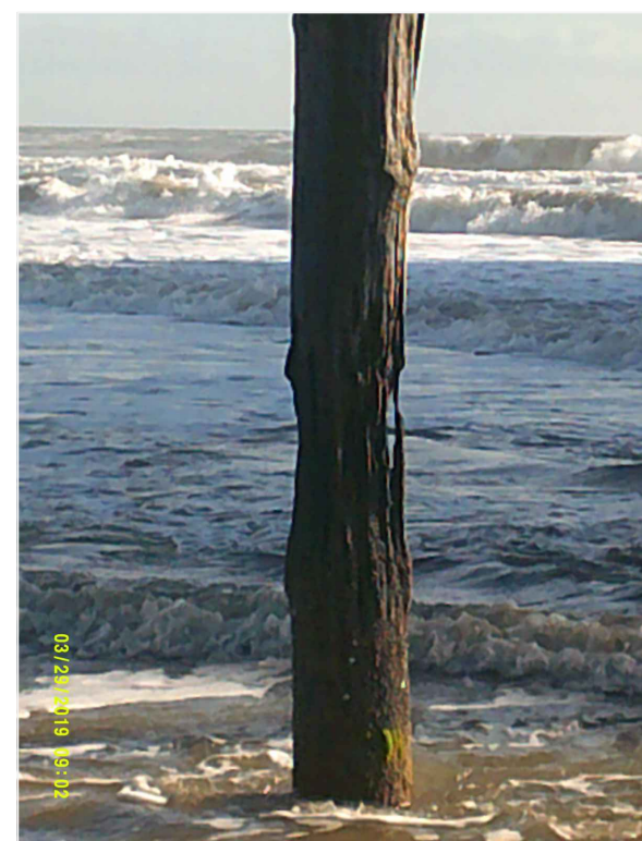
BENT 12: ROTTED PILE
