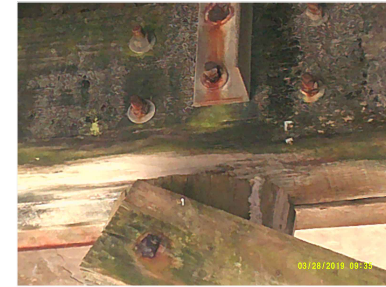
BENT 4: 4" GAP AT PILE TO PILE CAP
