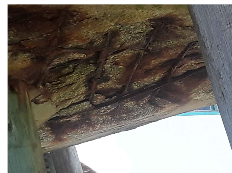
BENT 14: CONCRETE SPALL
