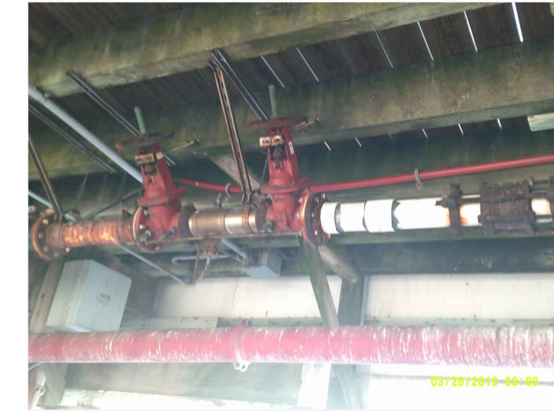
BENT 4: PURCHASE OF BACK FLOW PREVENTER
