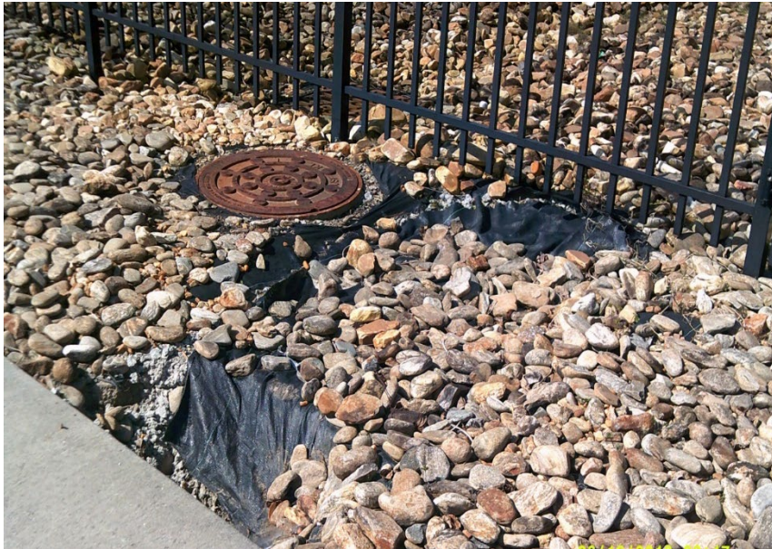
Figure 10: 1 Governmental Avenue MH G285
