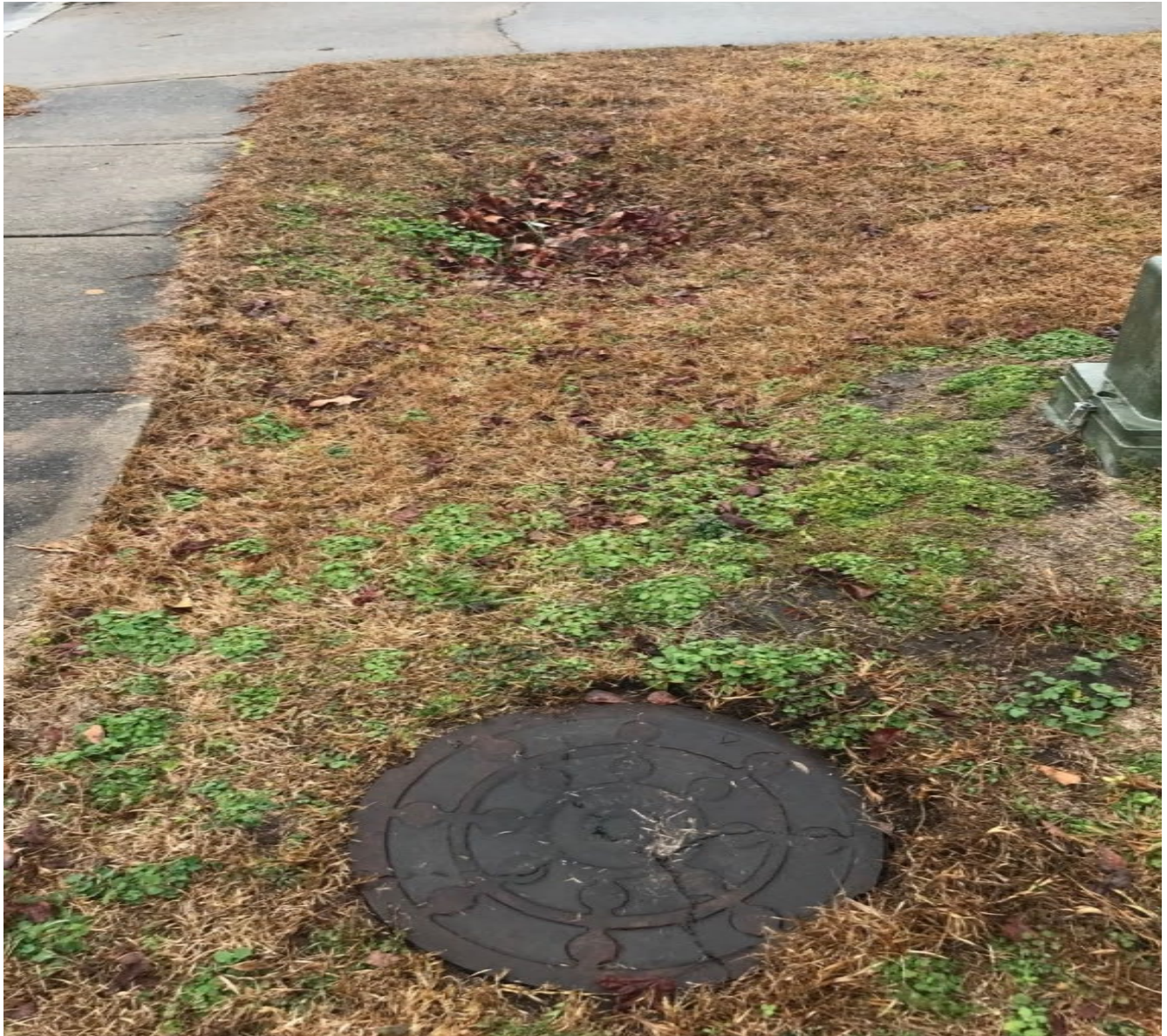
Figure 5: 131 Twin Wood Drive MH HS7
