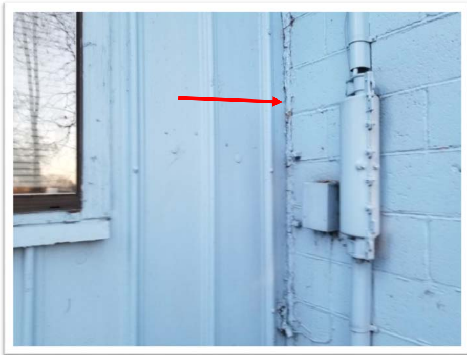
Photograph #20 Building Exterior at Interface of CMU Block Wall and Sheet Metal – Caulk at Building Interface is 5% Chrysotile.
