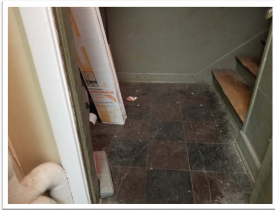
Photograph #15 Entry to 2 nd Deck Stairs – 12”X 12” Black and Brown VFT/Mastic (5% Chrysotile/5% Chrysotile).
