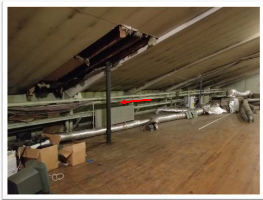
Photograph #22 2 nd Deck - TSI Pipe Wrap is 25% to 25% Chrysotile and 15% to 18% Amosite. TSI and Pipe Wrap Throughout the Building is Asbestos Containing.
