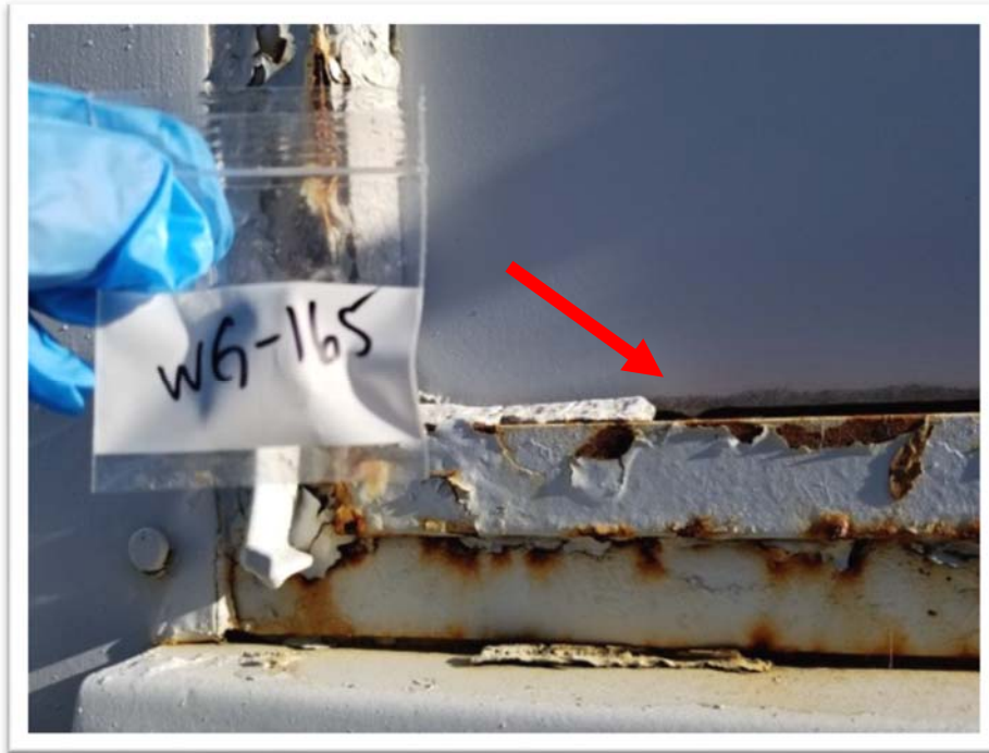
Photograph #17 Exterior Window Between Machine Shop and Main Propulsion – Close Up View of 3% Chrysotile Window Glazing
