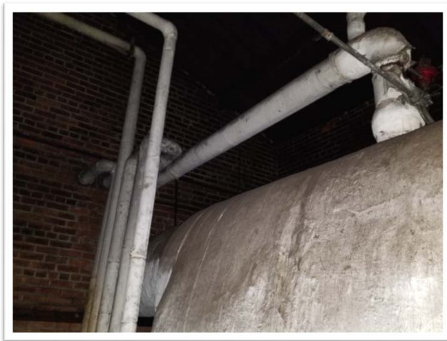
Photograph #18 Boiler Room, Boiler Jacket – 20% Chrysotile
