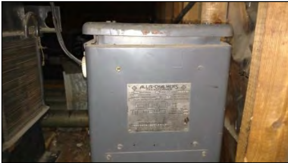
View of an old transformer in the attic.
