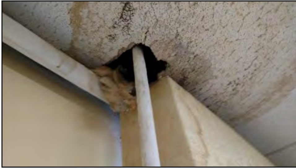
View of water damage in an office.
