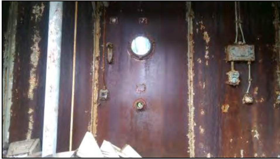
View of the interior of the structure on the southern property boundary.
