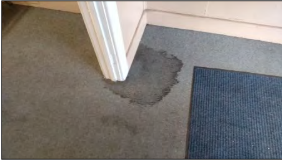
View of water infiltration at the entrance of the building.
