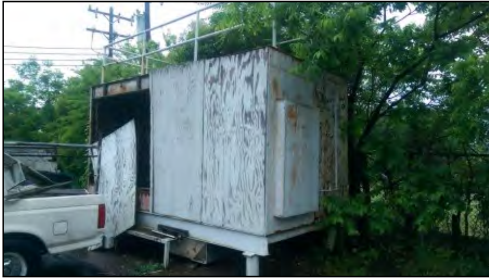
View of the exterior of the structure on the southern property boundary.
