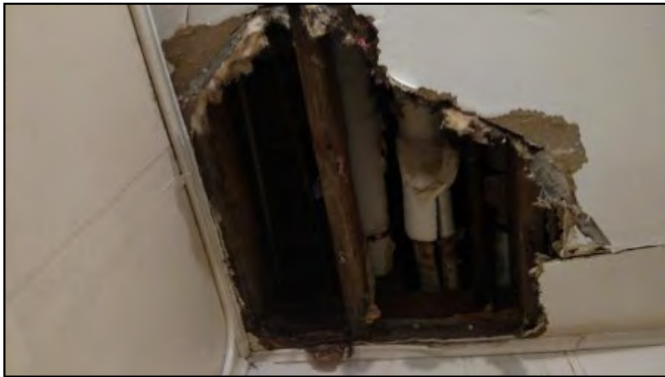
View of another area of water damage on the ceiling of an office.
