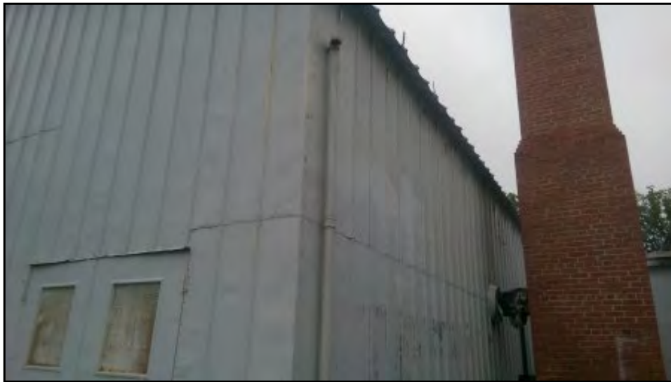
View of a suspect vent pipe on the southern side of the building.
