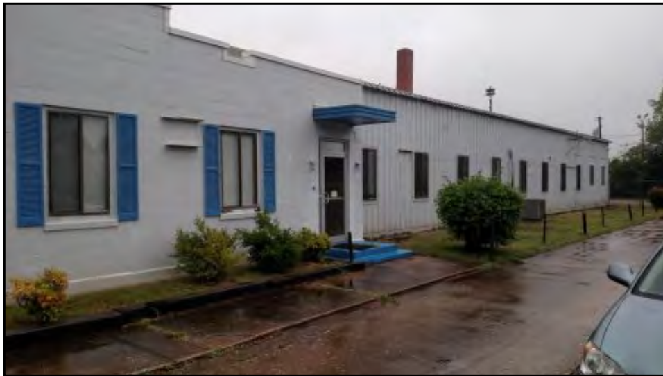
View of the west side of the building from the northeastern side of the building.
