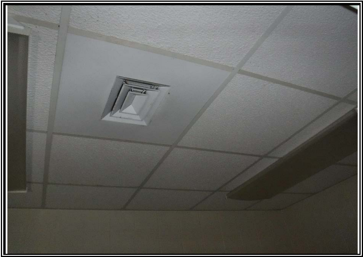
3. Asbestos containing materials –textured lay-in ceiling tile
