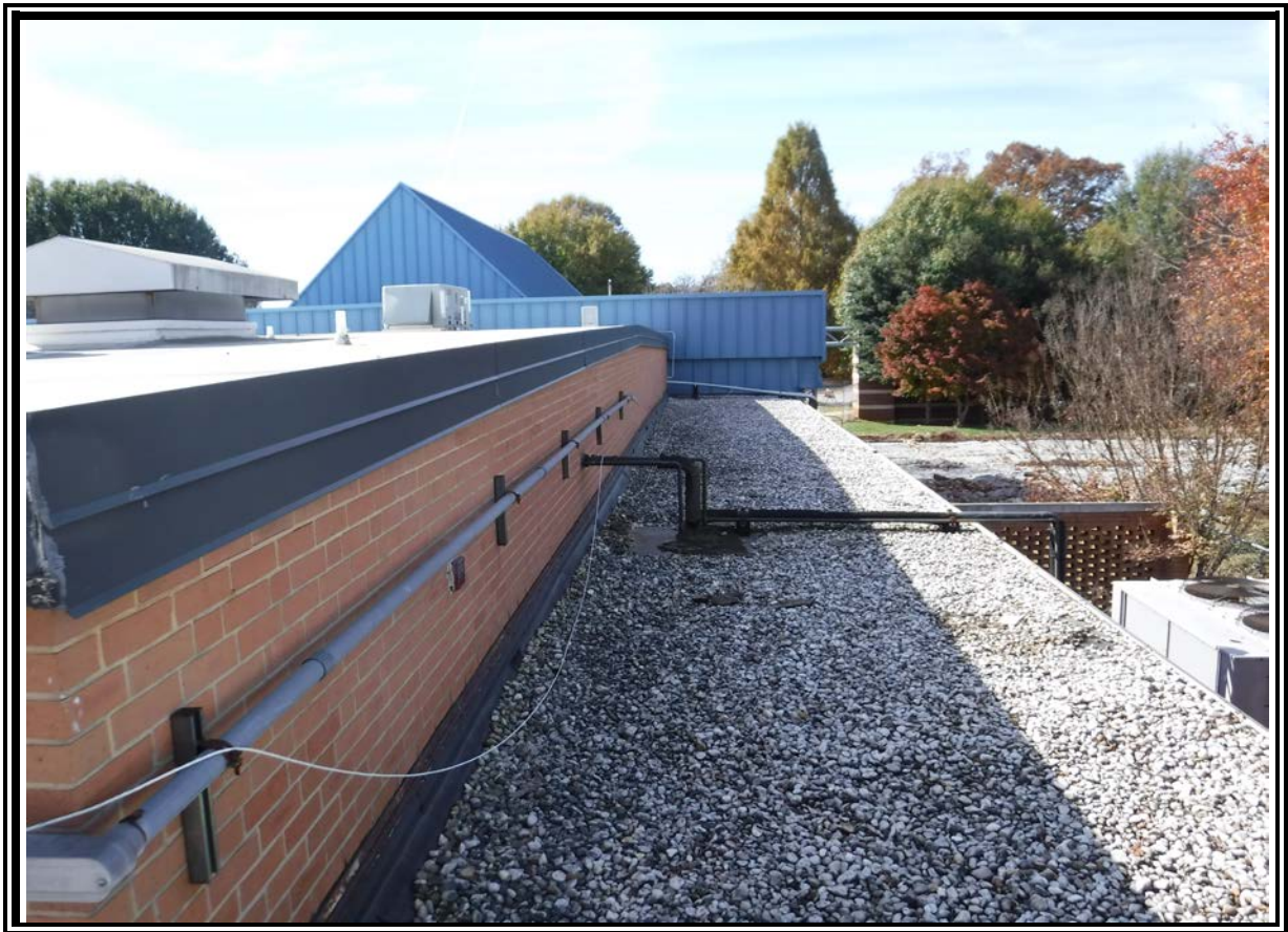
6. Asbestos containing material – built-up roofing materials on covered walkway
