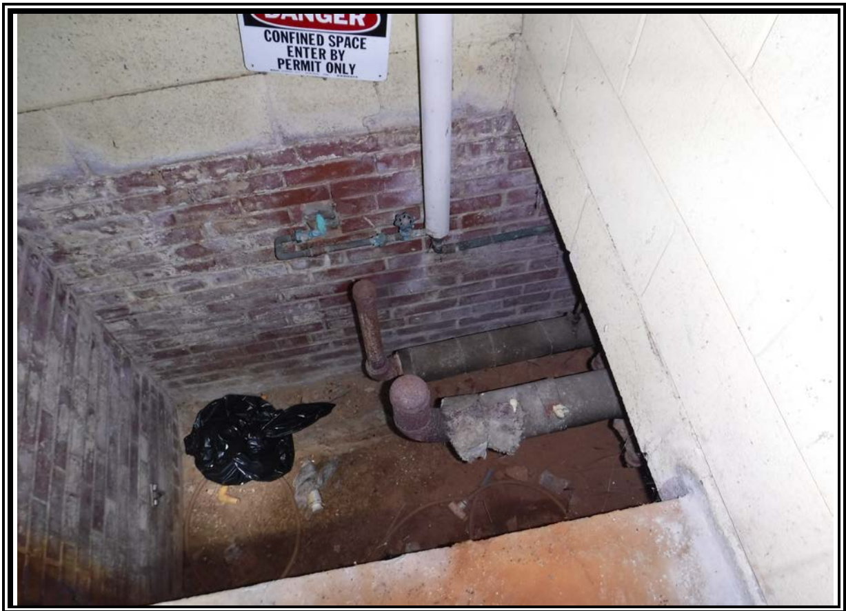
4. Asbestos containing material – black pipe wrap on piping
