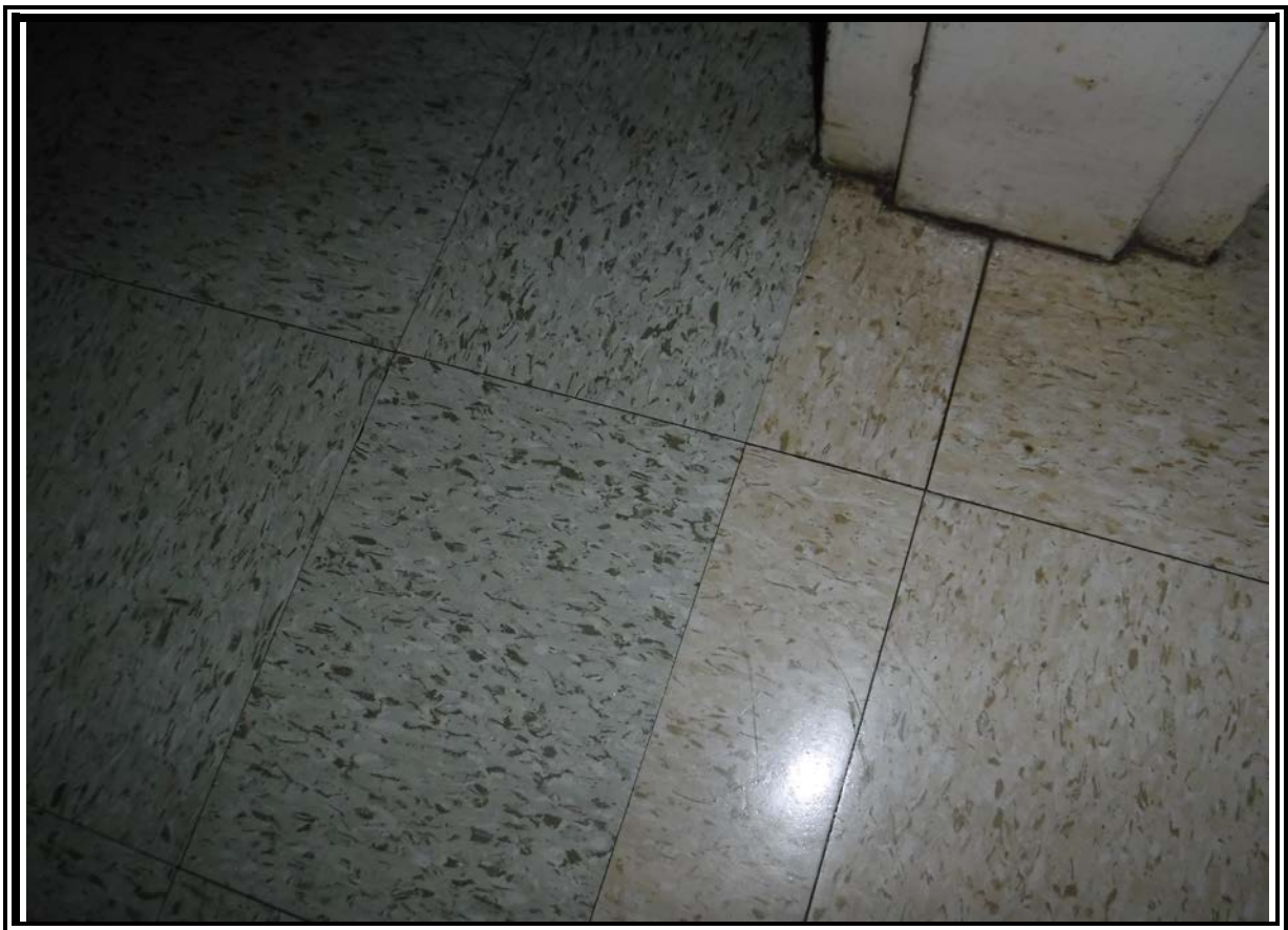
2. Asbestos containing material – floor tile (both types) and mastic
