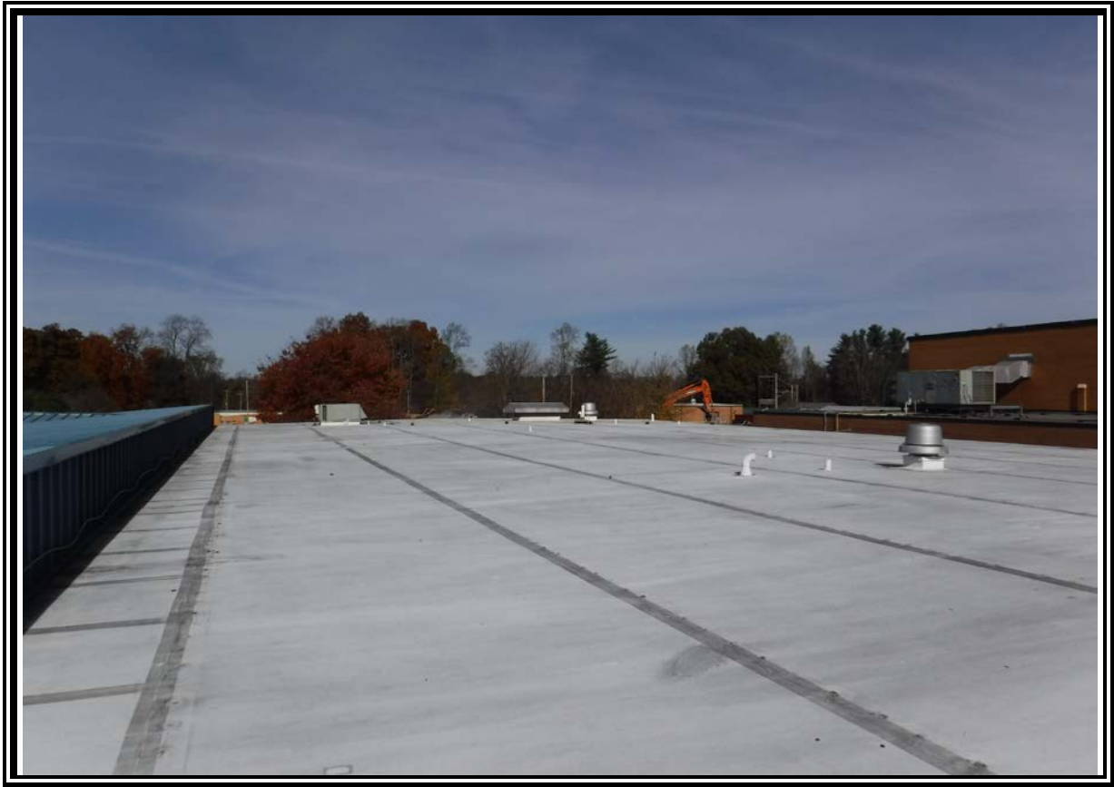
5. Asbestos containing materials –built-up roofing materials on “B” Building
