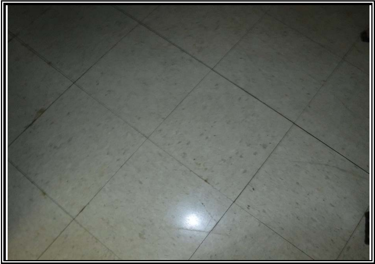
1. Asbestos containing materials – floor tile and mastic
