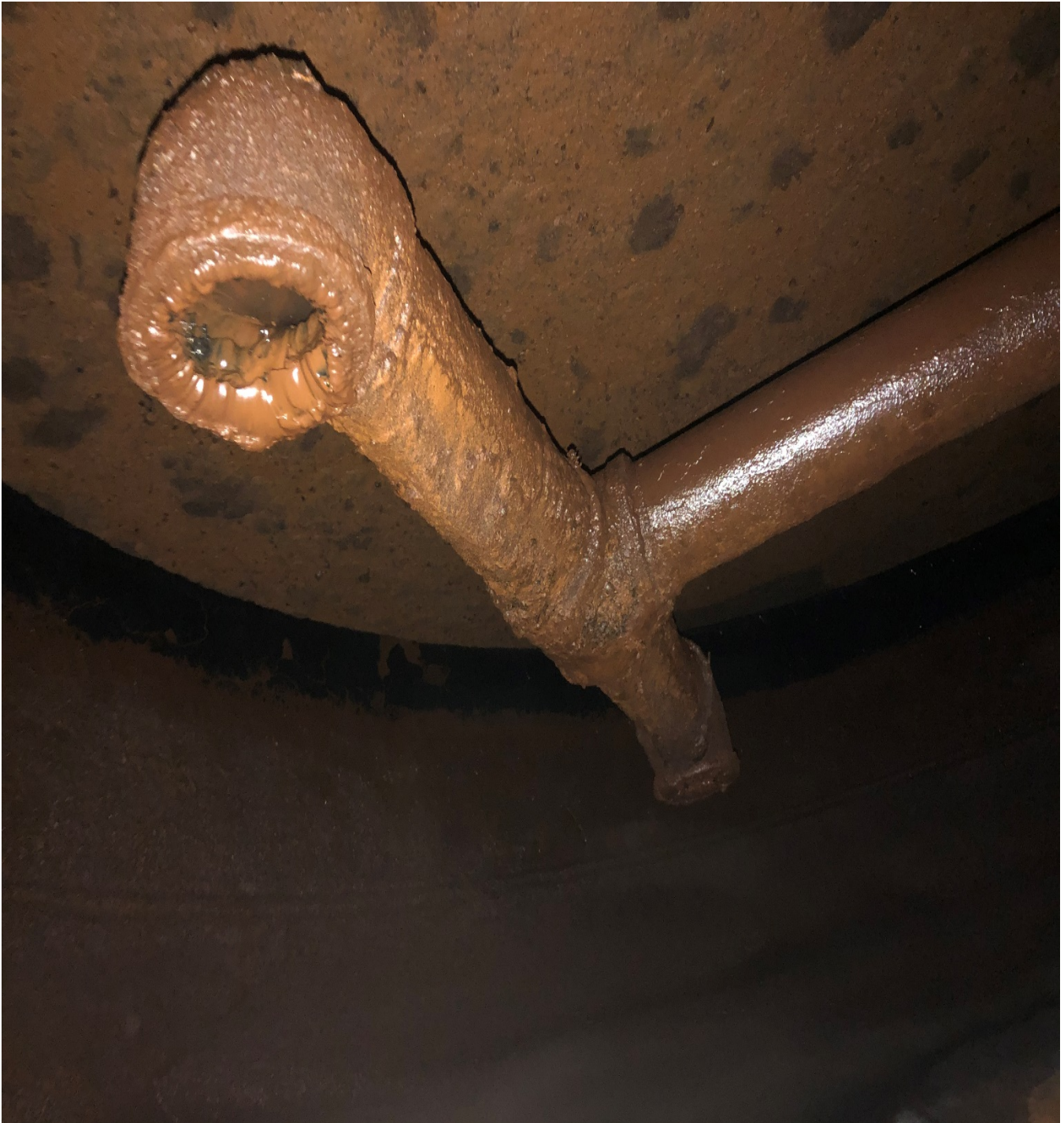
Figure 10 Filter Inlet Distributor Arms
