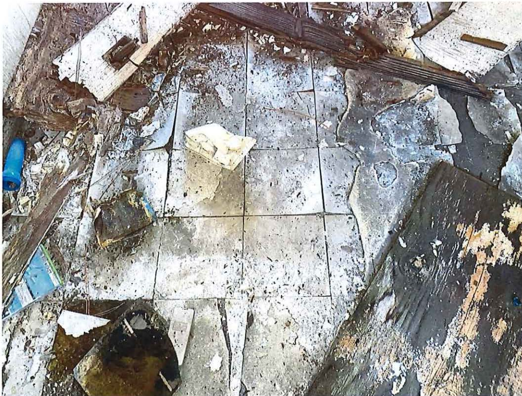
9"X 9" Floor Tile (Beige) w/Black Mastic Throughout House
