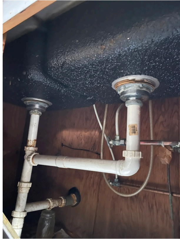
View of asbestos-containing Black Sink Coating (HA 408-7)
