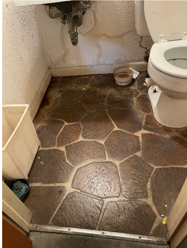
View of asbestos-containing Large Stone Pattern Sheet Flooring and its associated Yellow Mastic (HA 409-5)
