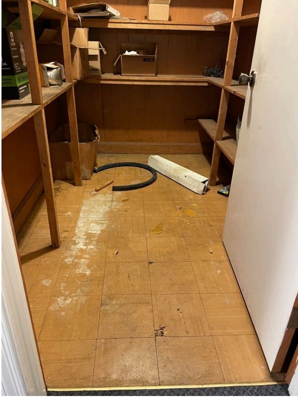
View of asbestos-containing 9" x 9" Brown/Tan Floor Tile and its associated Black Mastic (HA 408-13)
