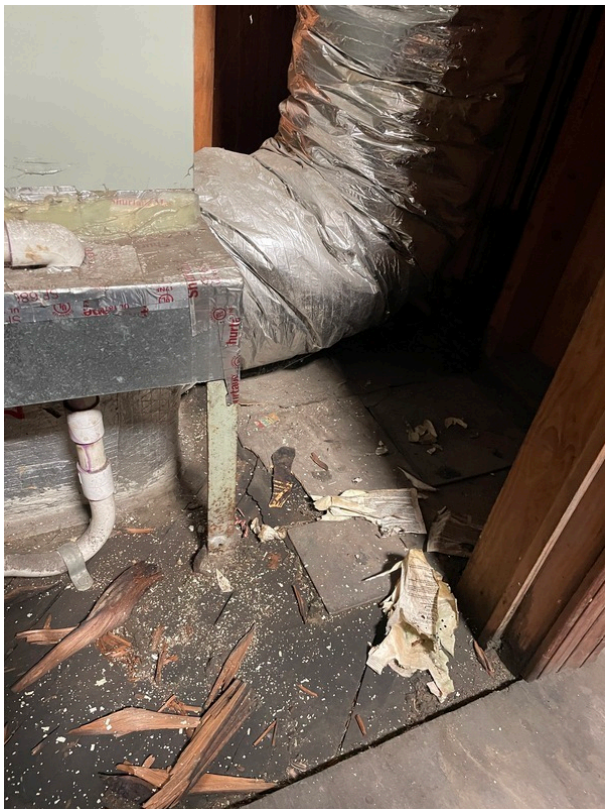
View of asbestos-containing 9" x 9" Brown/Tan Floor Tile and its associated Black Mastic (HA 408-8)
