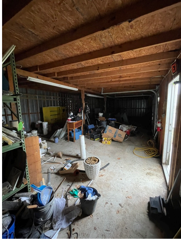
General view of the interior of the 410 Jones Street South commercial structure
