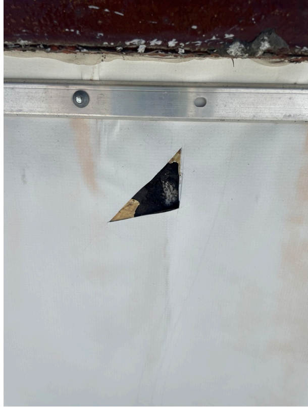
View of asbestos-containing Black Tar located behind rubber membrane on the parapet wall of the roof (HA 419-18)
