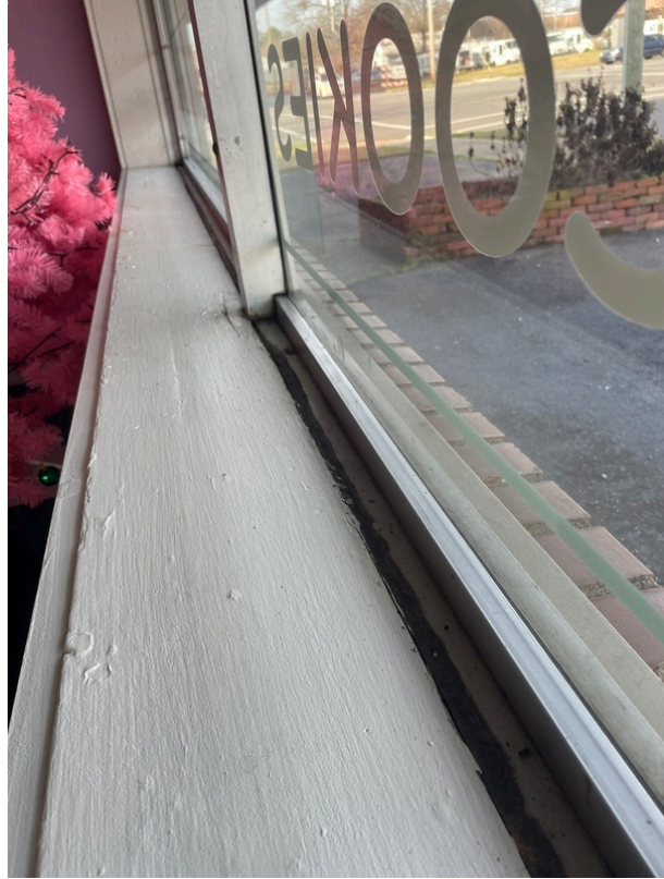
View of asbestos-containing Off-White Interior Window Frame Caulk (HA 419-3)
