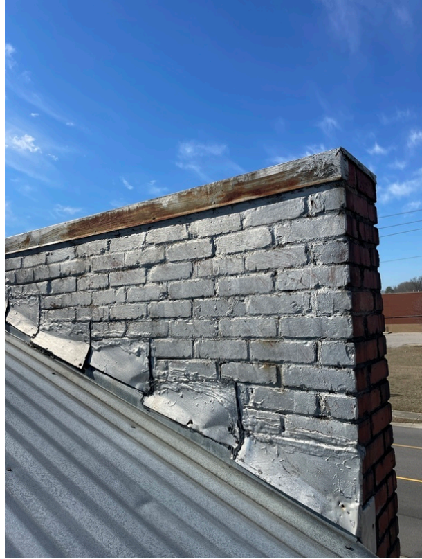
View of asbestos-containing Silver Coating and its associated Black Tar (HA 411-3)
