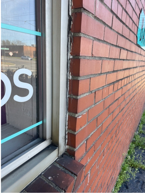
General view of asbestos-containing Gray Exterior Window Frame Caulk beneath White Caulk (HA 419-11)
