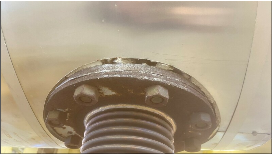
6 - View of the tank insulation
