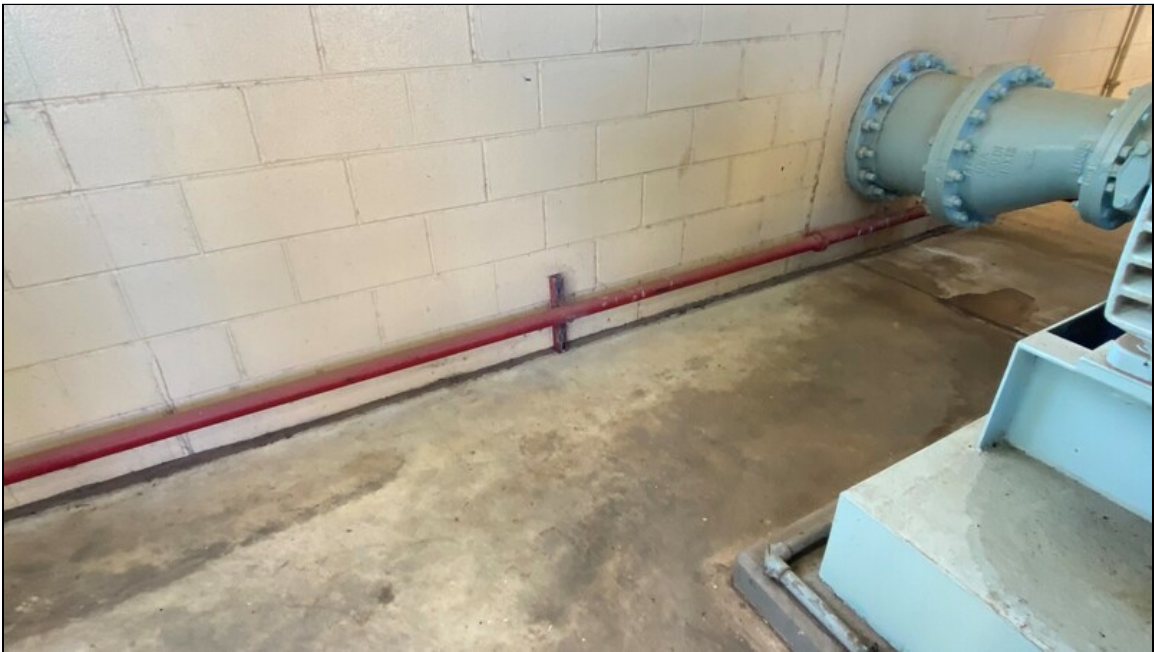
4 - View of red paint on pipes and blue paint on base of equipment
