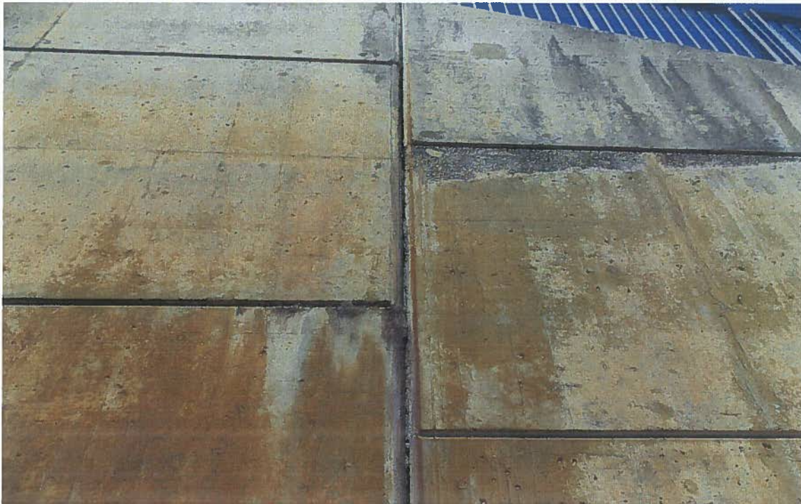
Downstream - South Mid-Panel Wall. Note Seepage Staining and Joint Deterioration.
