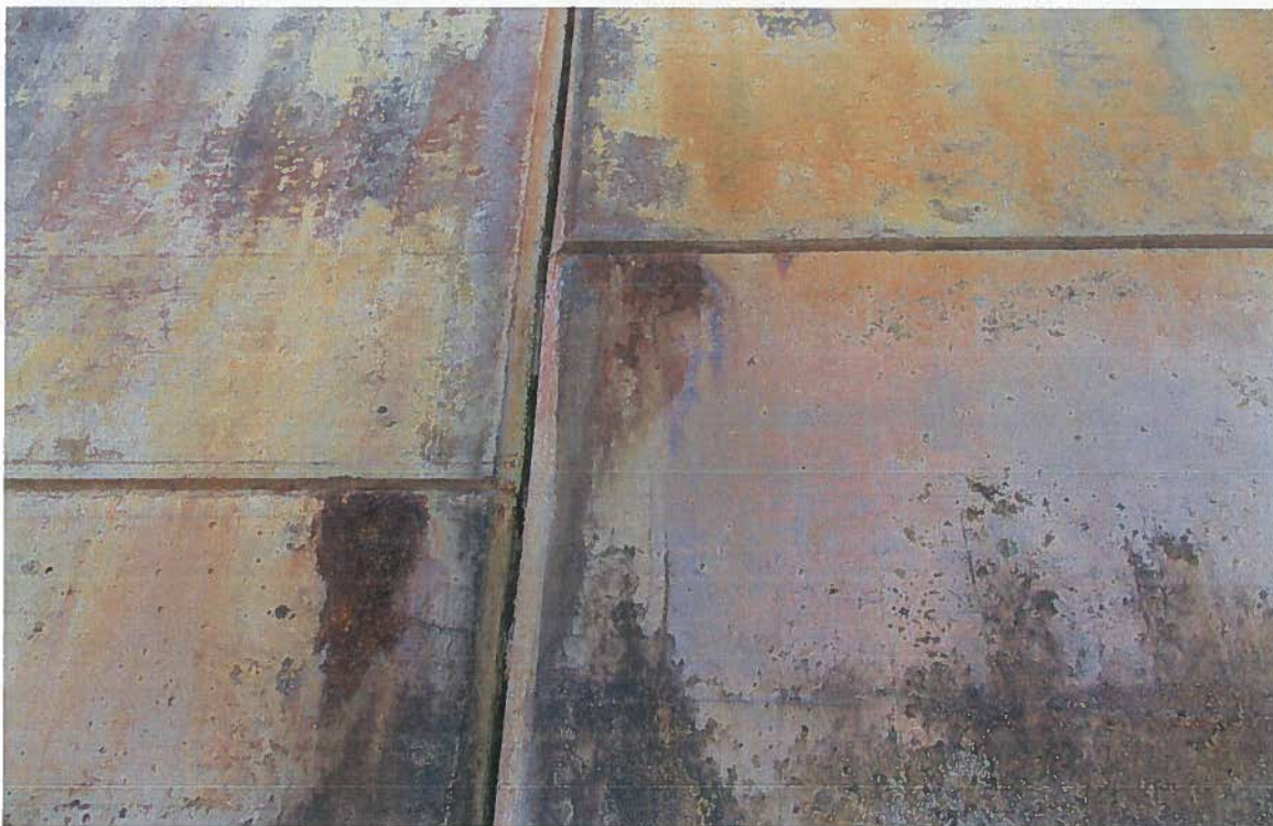
Downstream - North Mid-Panel Wall. Note Joint Filler Deterioration.
