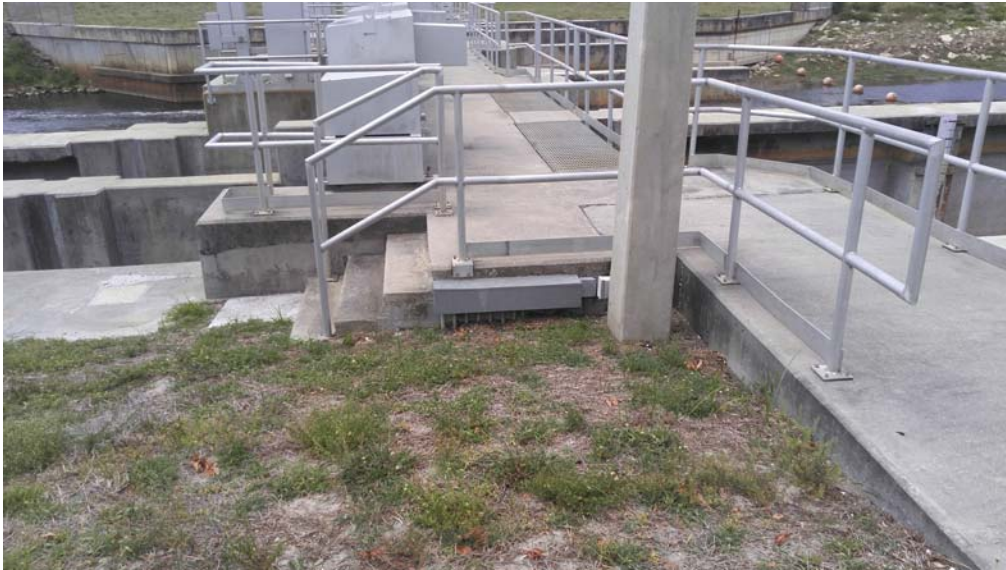
Catwalk junction box for flow gates
