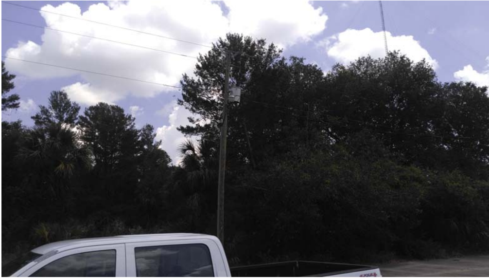
Electrical power service pole
