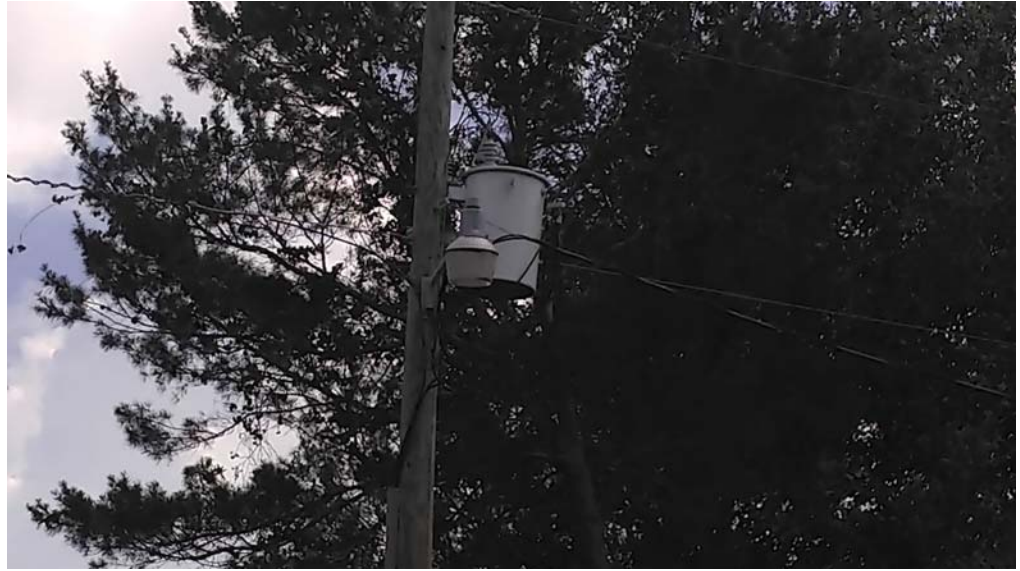
Electrical power service
