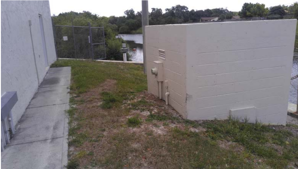
Pump house power supply and water line feeder to discharge valve
