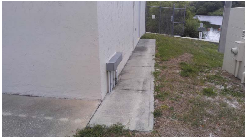
Close up of flow gates junction box along southside of building
