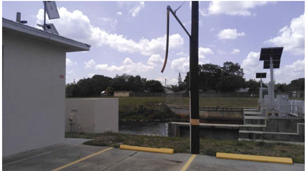
Pump discharge point
