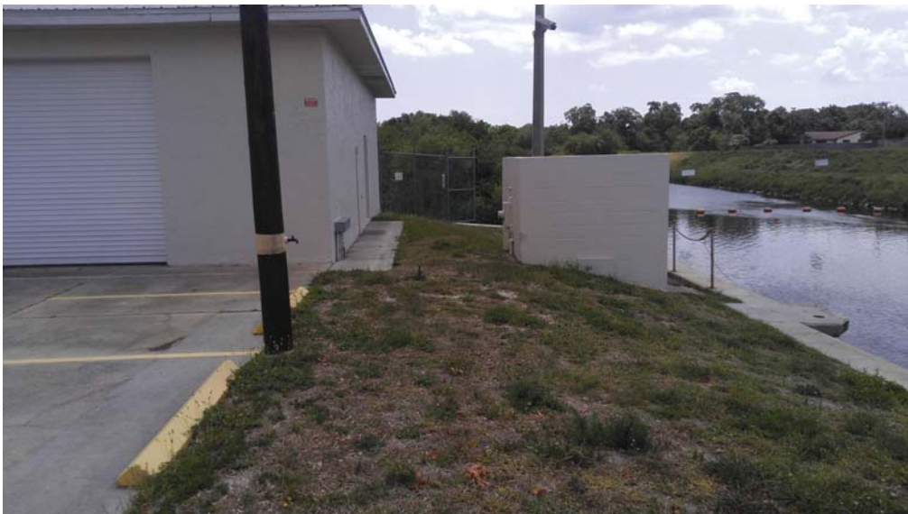
Pump hose and SW corner of building showing junction box for flow gates
