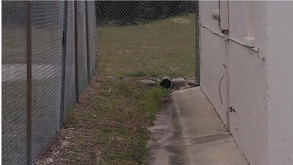
Stormdrain pipe to retention pond along northside of building
