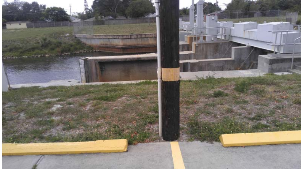
Pump water riser and valve
