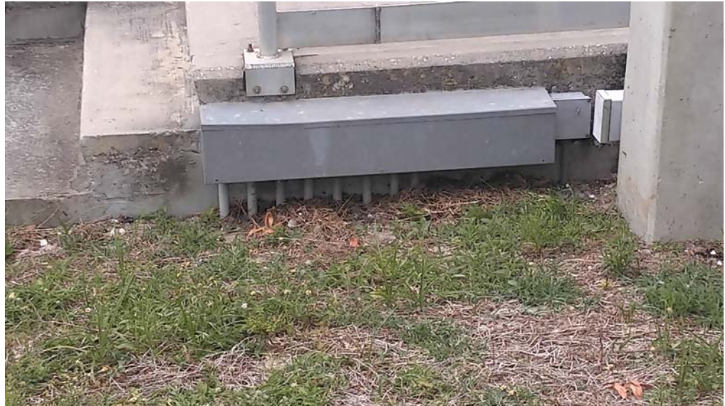
Close up of junction box for flow gates
