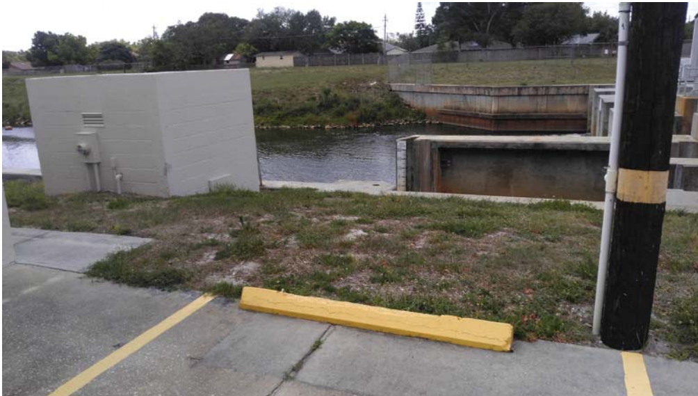
Pump house and riser
