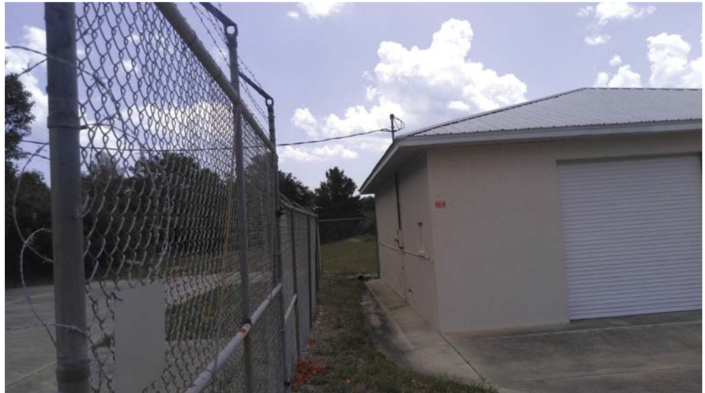
Weather head for power service on northside of building
