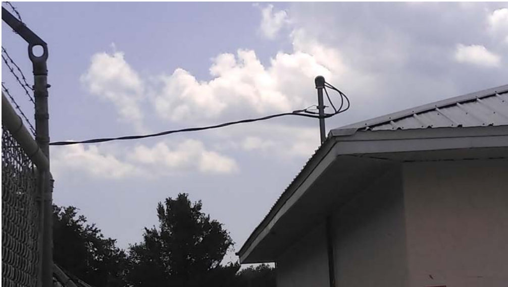
Weather head for power service to building
