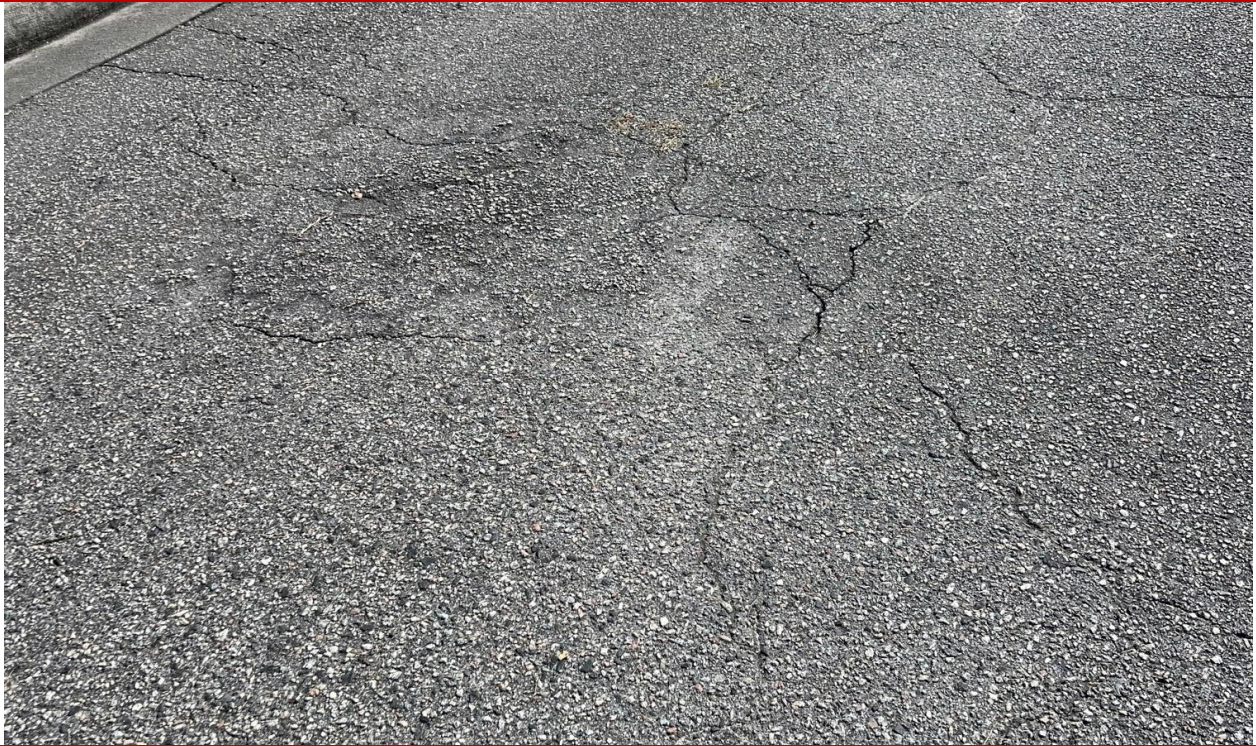
Low severity longitudinal and transverse cracking, a small depression was also observed near the entrance gate
