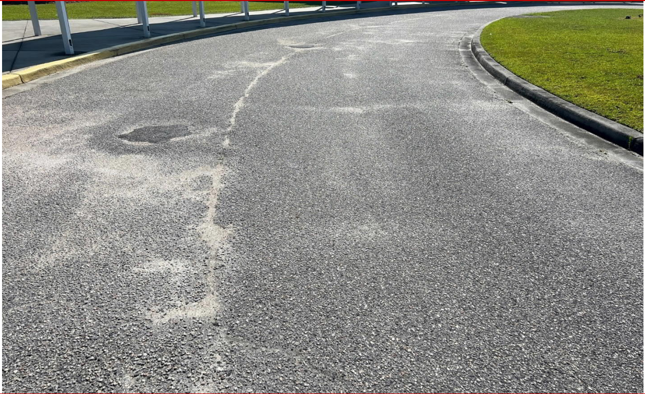
Low severity longitudinal cracks, depressions, and patching near the end of the existing loop
