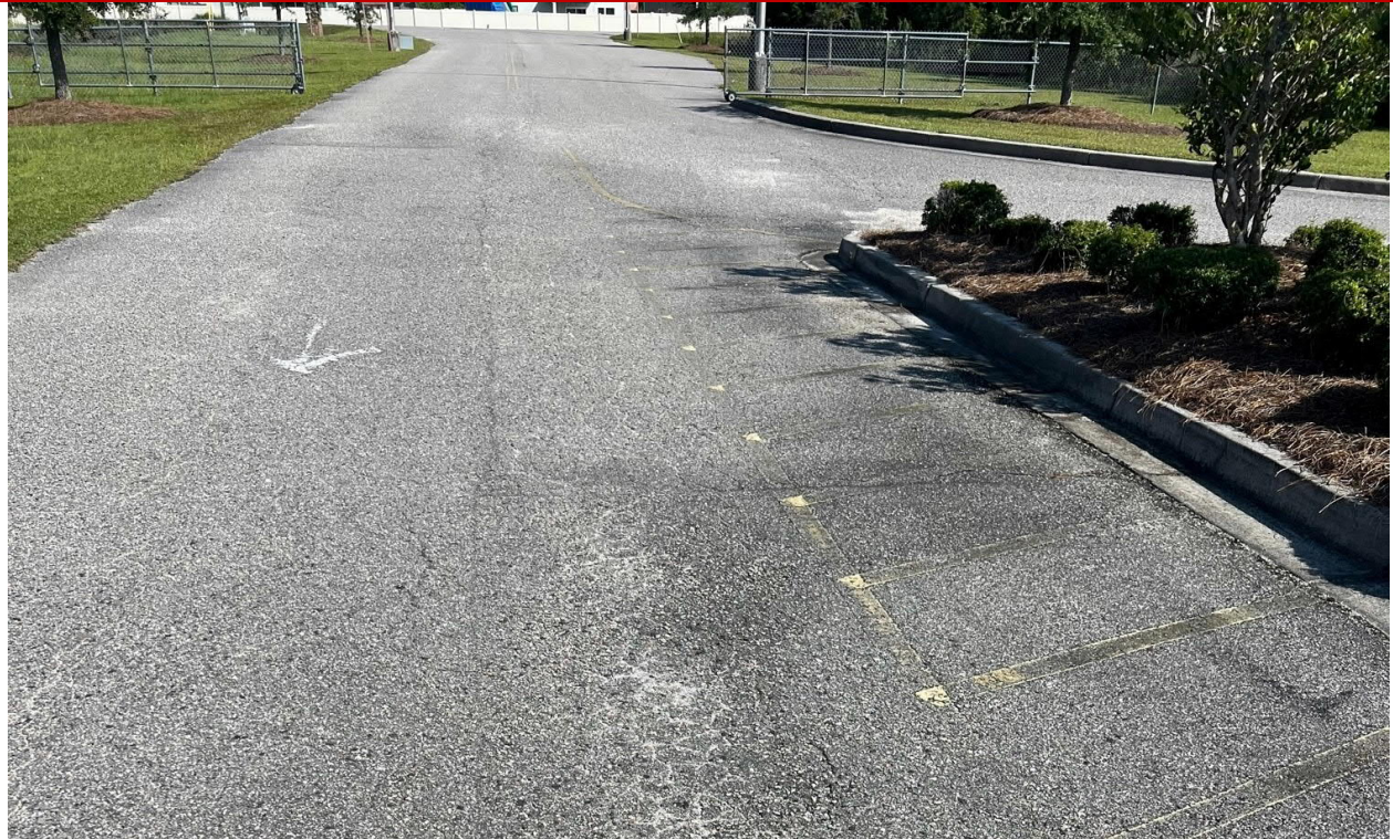
Low severity fatigue cracking and polishing near the entrance gate
