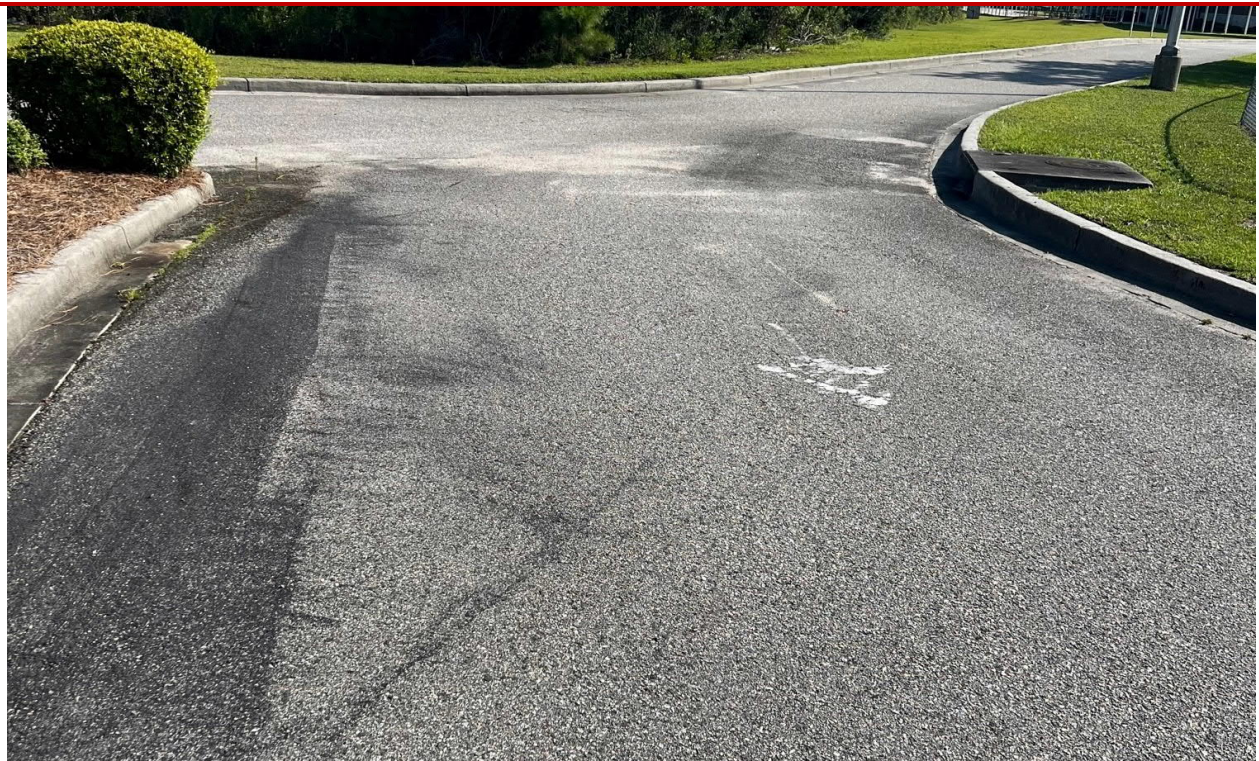
Low severity cracking polishing near the entrance gate
