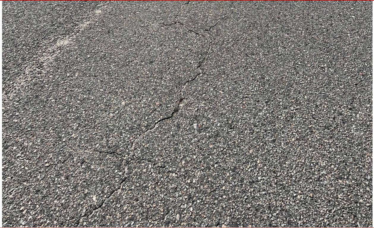
Low severity longitudinal cracking before the turn to the parking area
