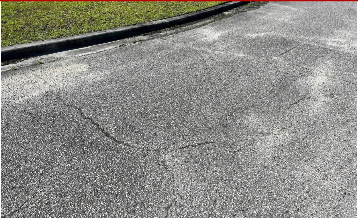
Low severity transverse and longitudinal cracking near the end of the existing loop
