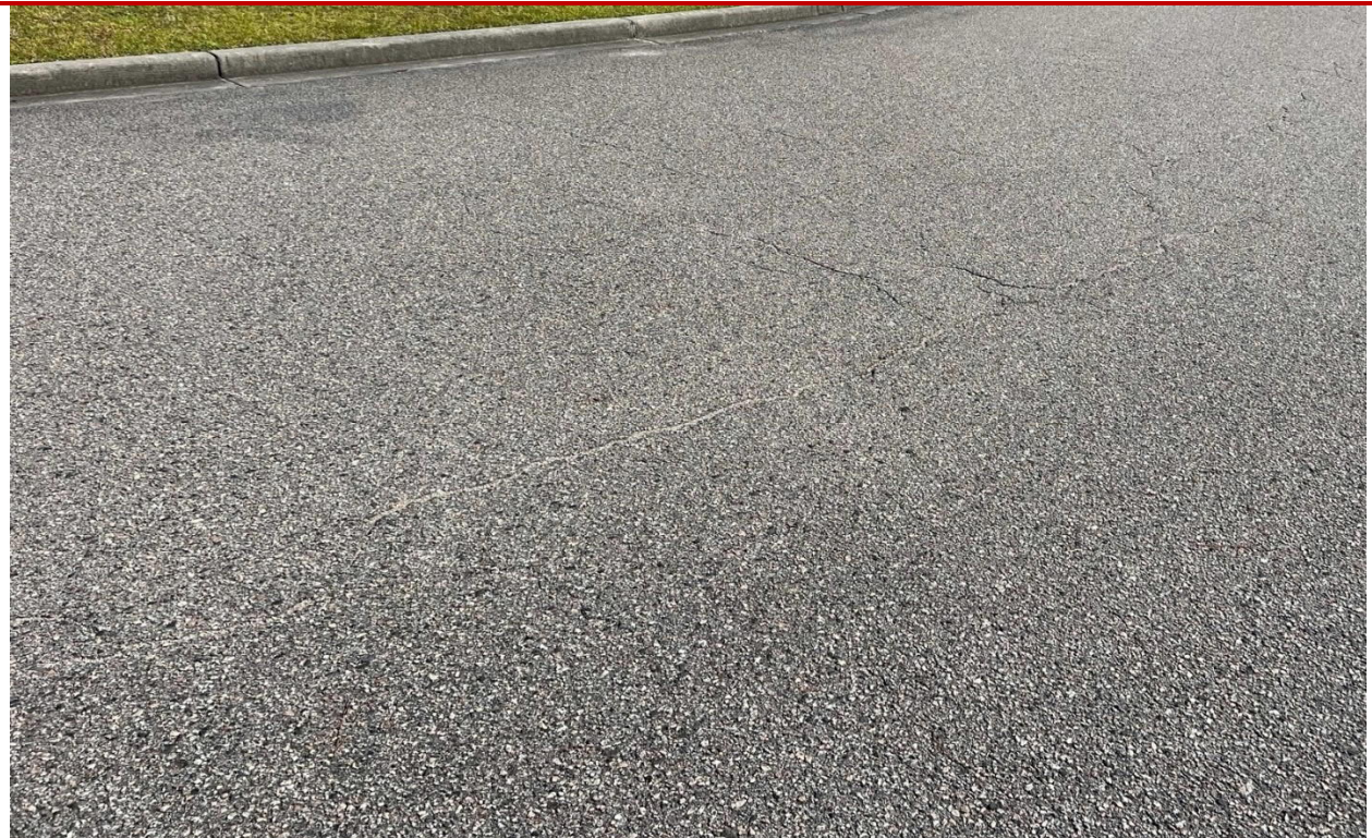
Low severity transverse and longitudinal cracking near HAB-05
