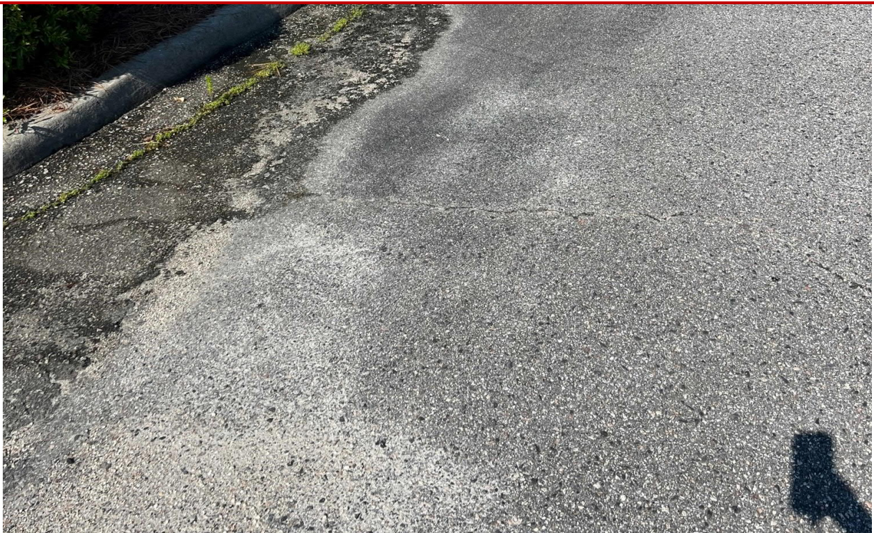
Low severity transverse cracking, polished aggregate and the evidence of ponded water near the entrance gate
