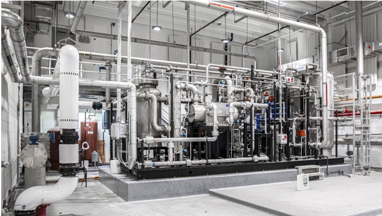
Figure 10. Typical Membrane Treatment Installation
