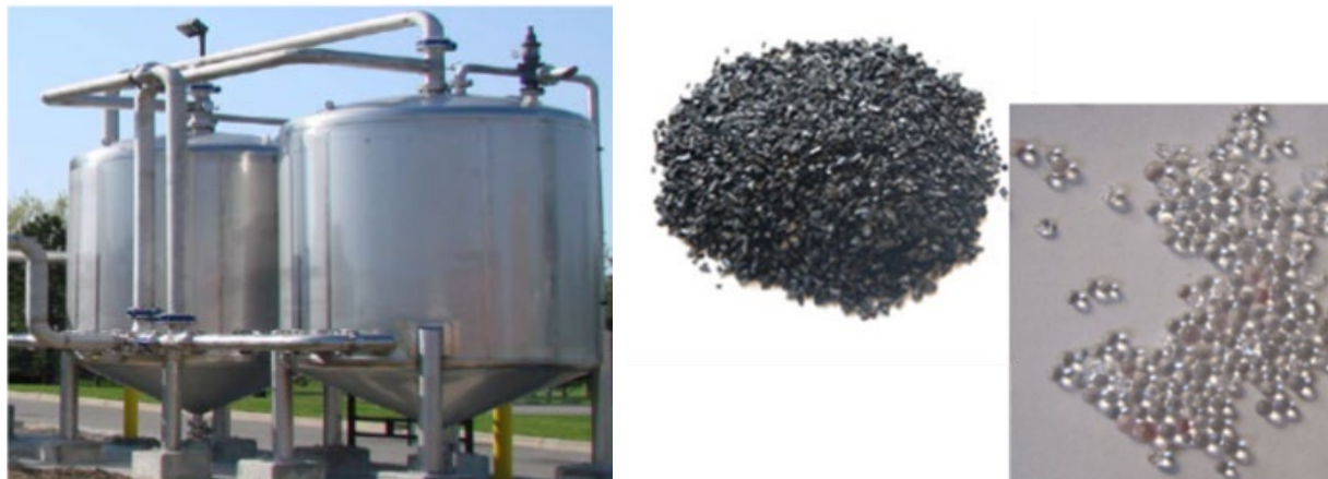
Figure 3. Siloxane Removal Equipment and Media
