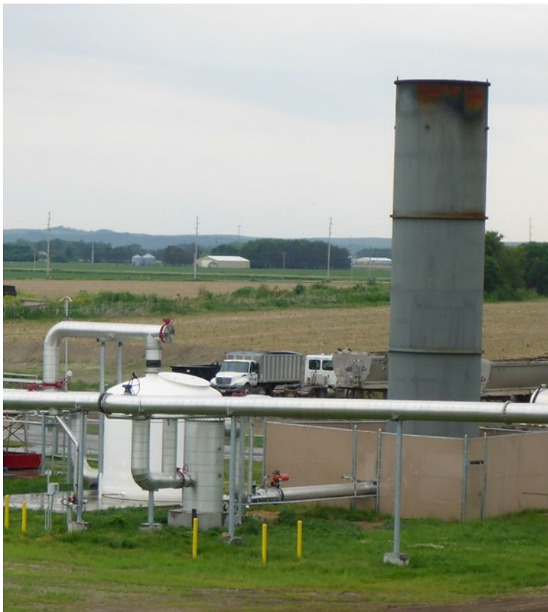
Figure 4. Enclosed Waste Gas Flare
