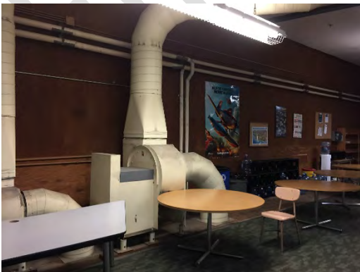
Existing fan (and filter?) on Hangar B mezzanine, over Composites Lab.
