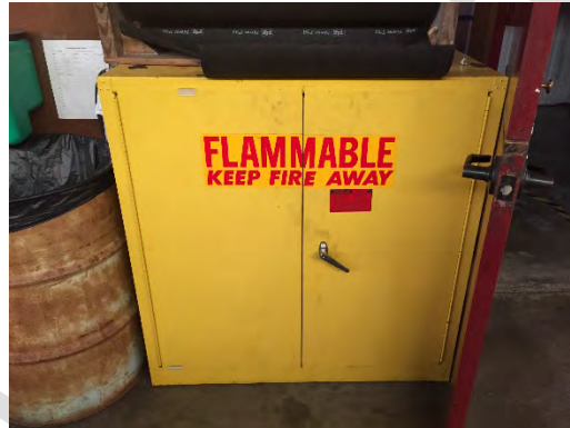
Flammables cabinet, Hangar A
