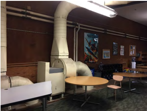
HVAC at Hangar B mezzanine, over Composites Lab
