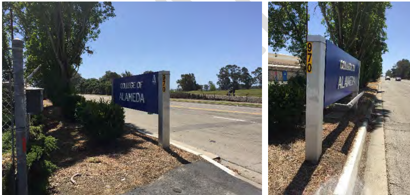
College of Alameda sign at campus entry, no electrical connection for sign light
