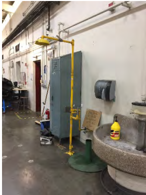
Sink + eyewash, Hangar A
