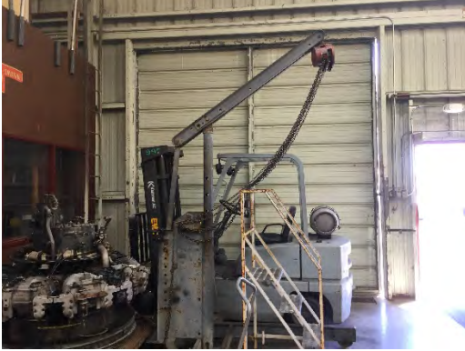
Portable hoist, Hangar A Engine Area
