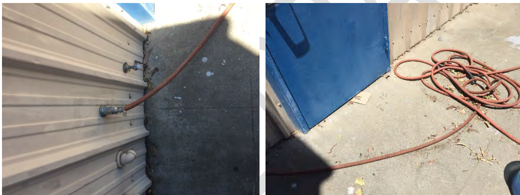
Compressed air spigot at exterior, near Valve Grinding Room
