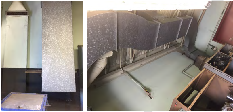
Ventilation and ductwork at corrosion room
