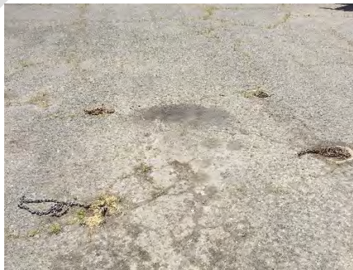
Engine test tie-downs in outside yard
