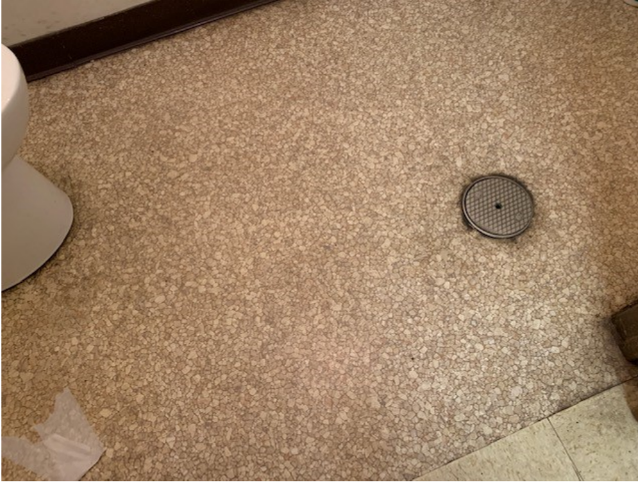
Photograph 3: View depicting asbestos-containing sheet flooring in Headhouse.
