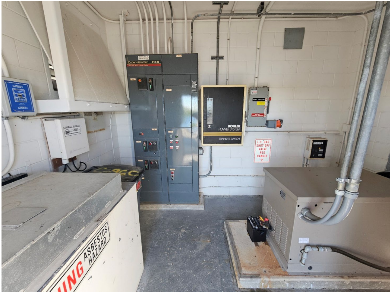
FIGURE 1: S-96C WATER CONTROL STRUCTURE TRANSFER SWITCH LOCATION
