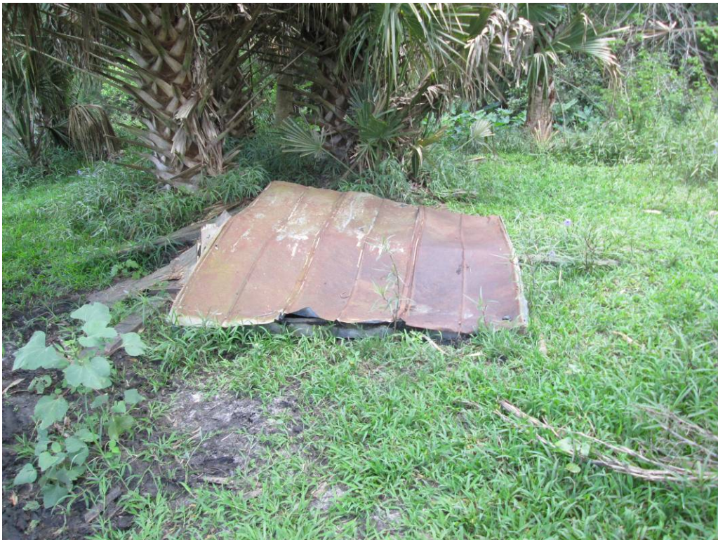
8. View of the remnants of a wooden structure observed on the northwestern portion of the site.
