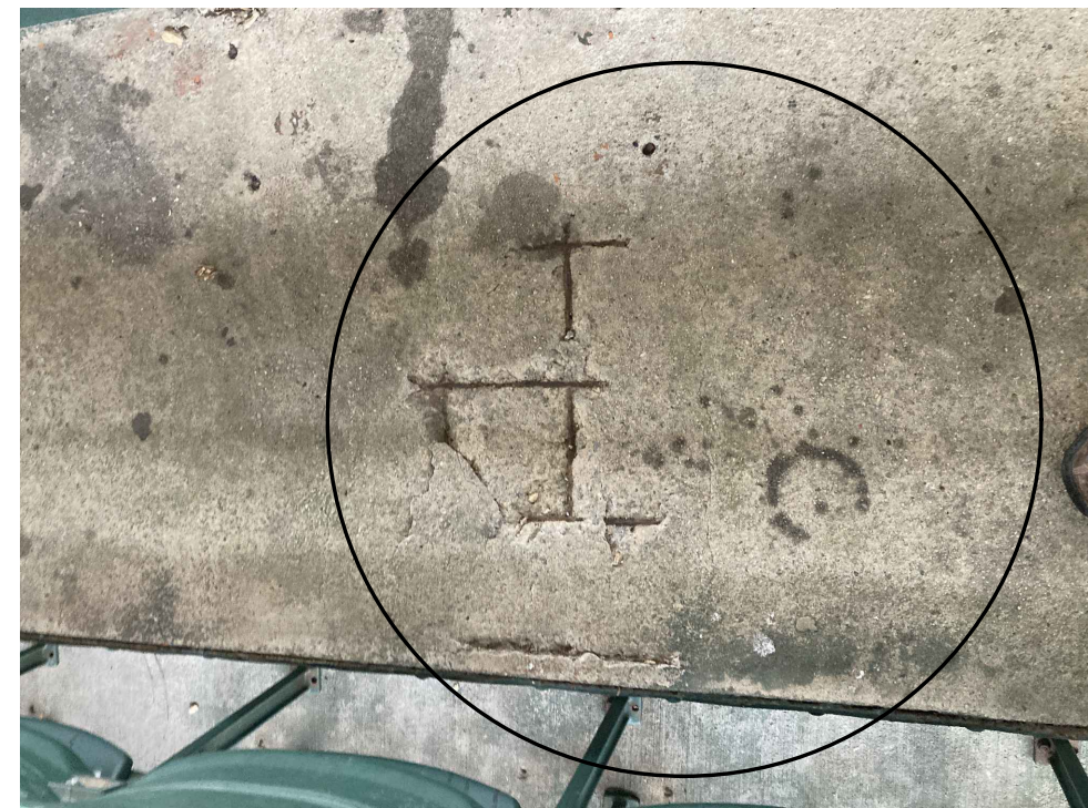
EXAMPLE OF SPALLING CONCRETE
