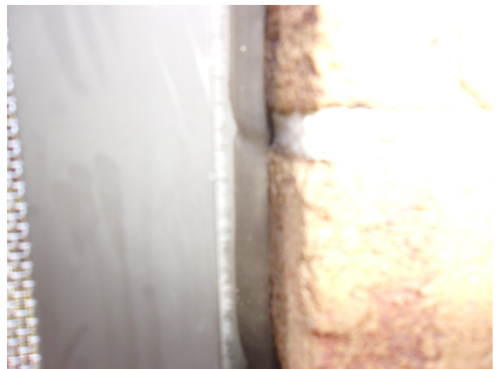
Photo 12 – Typical view of interior and exterior black window caulk throughout buildings 7 to 35.
