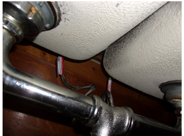
Photo 10 – Typical view of a kitchen sink with white undercoating throughout buildings 7 to 35.
