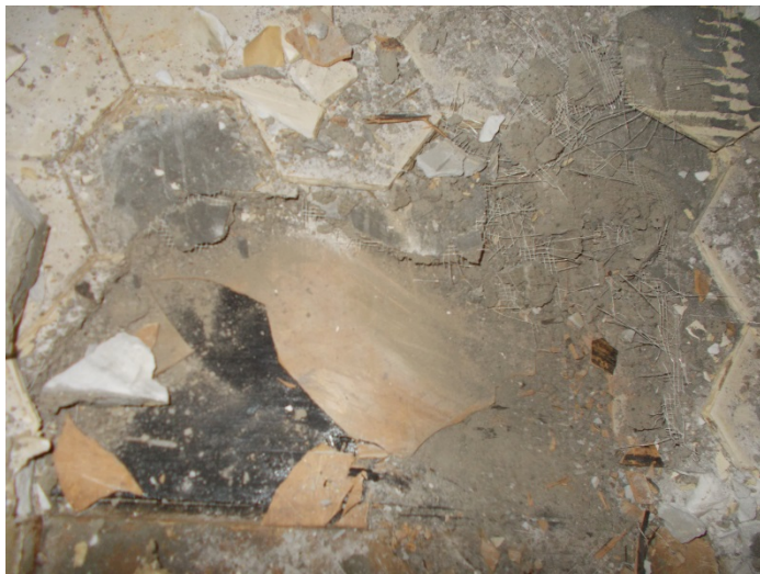
Photo 41 – Typical view floor tile and mastic under ceramic tiles in bathrooms throughout Buildings 7 to 35.
