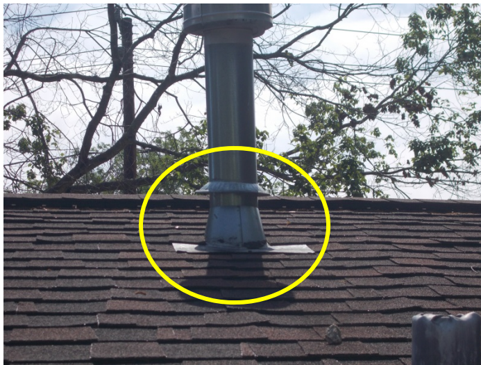
Photo 39 – Typical view of roof mastic/tar on roof penetrations throughout a portion of the buildings.
