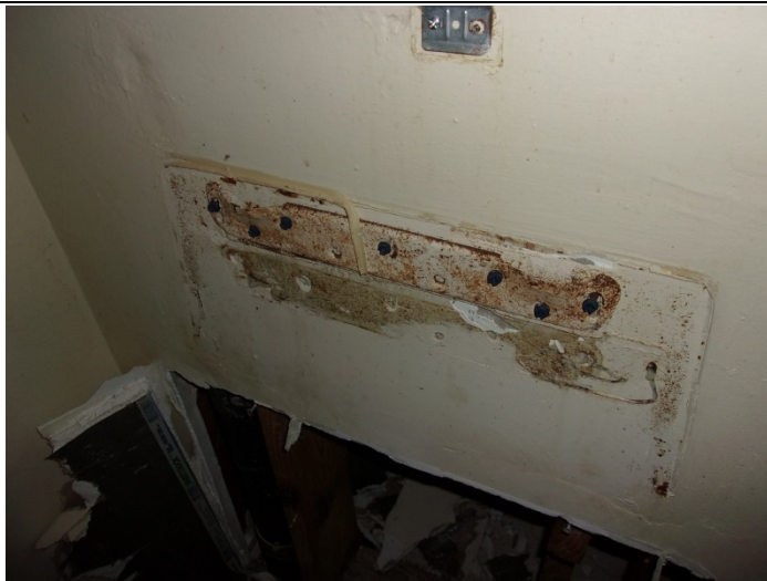
Photo 37 – Typical view of bathroom caulk on sinks throughout Buildings 7 to 35.
