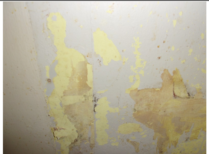
Photo 8 – Typical view of stove back splash mastic in a portion of Buildings 7 to 35.
