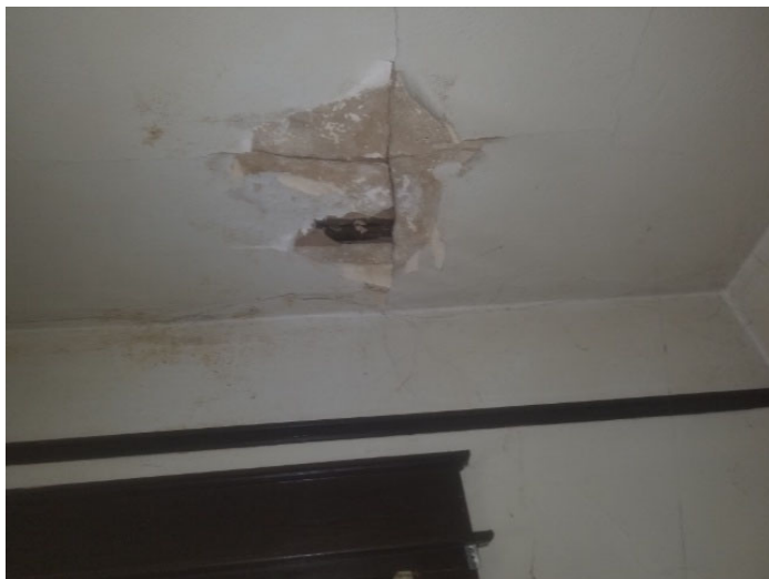
Photo 5 – Plaster throughout ceilings
