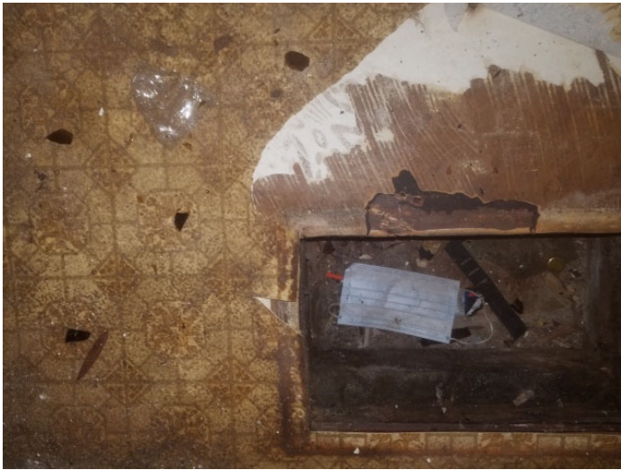
Photo 7 – Tan and brown roll vinyl flooring with second layer of tan and red flooring in front right room
