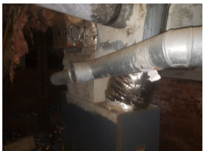
Photo 16 – HVAC tape in the basement area
