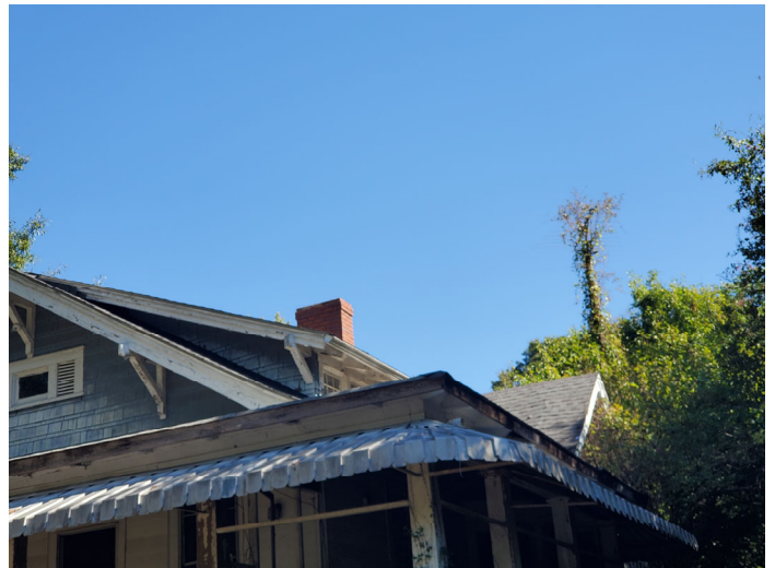
Photo 18 - Right chimney with tar assumed ACM.
