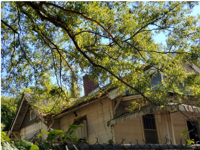
Photo 17 – Left chimney with tar assumed ACM.
