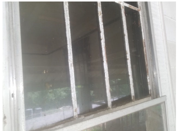
Photo 6 – Glazing found on wood windows
