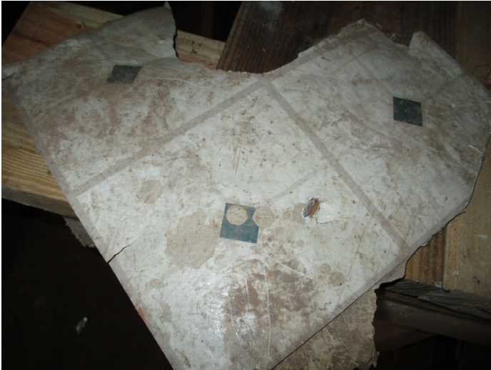
Photo 13 – Two layers of flooring. Square and diamond patten top layer, tan second layer located in crawlspace.
