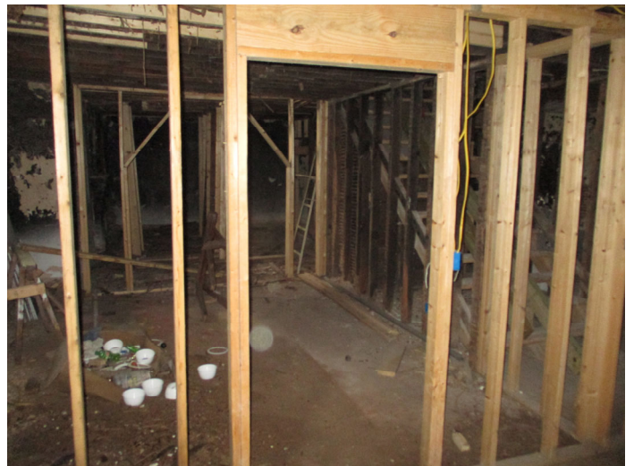
Photo 16 – Unfinished basement area with building material debris.
