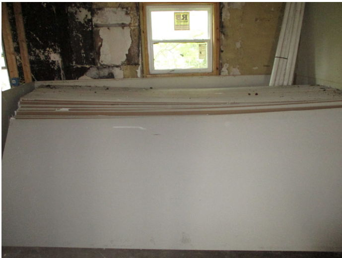
Photo 9 – Stacks of drywall located sporadically throughout.
