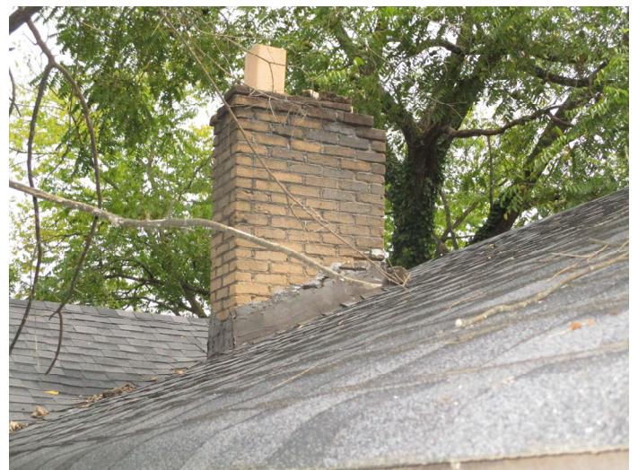
Photo 2 – Assumed asbestos containing chimney tar.
