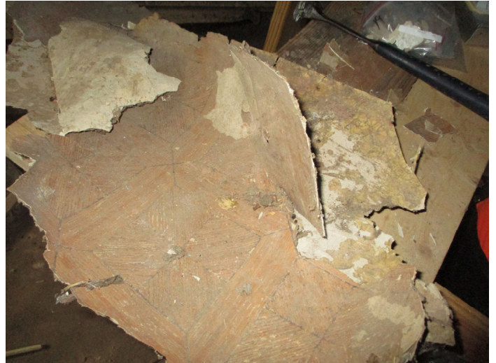
Photo 14 – Asbestos containing square wood pattern flooring over tan marble flooring located in crawlspace.
