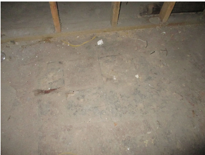
Photo 15 – Asbestos containing 9"x9" floor tile & mastic located in the back left corner in the basement.
