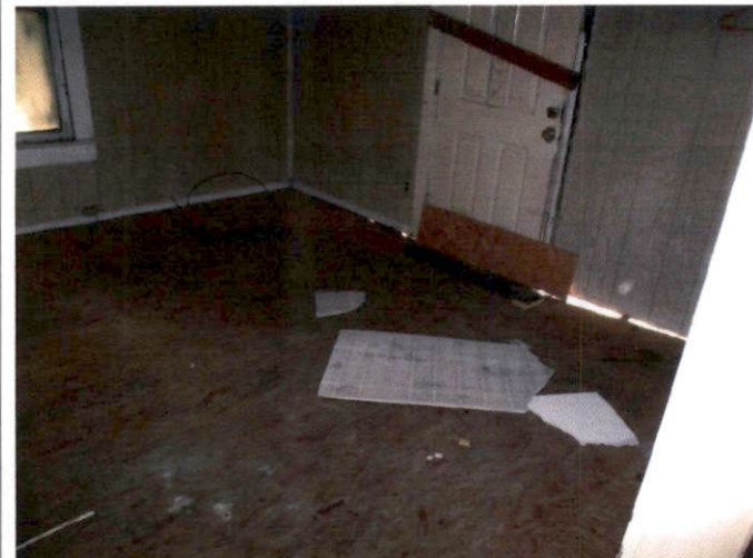
Photo 11 – Floors located in the rear of the house are sagging due to damaged floor joists.
