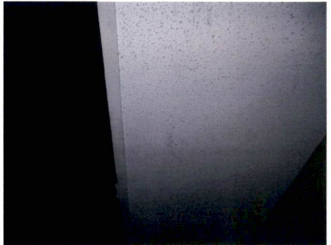
Photo 10 – Pinhole 2x4 ceiling tile located in back left room ceiling.
