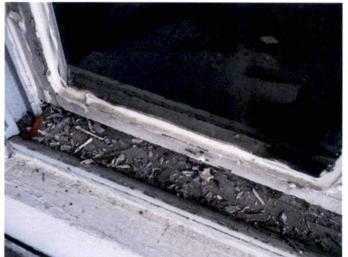
Photo 4 – Glazing debris located in window troughs
