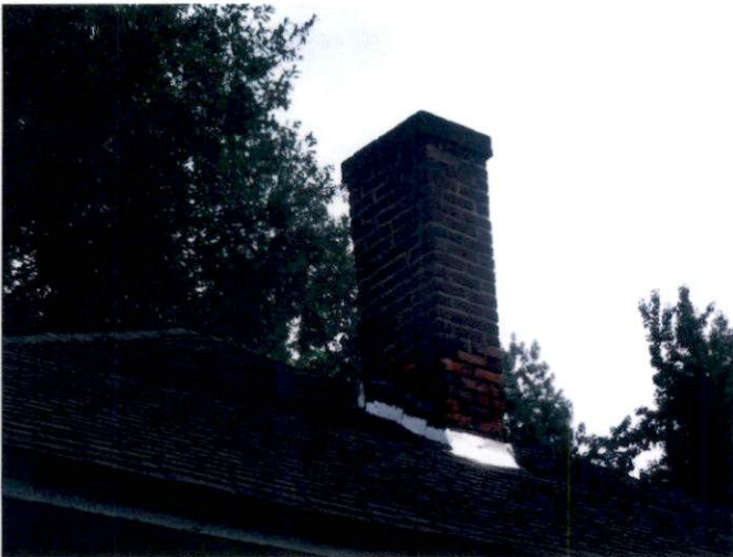
Photo 3 – Assumed asbestos containing tar on chimney.
