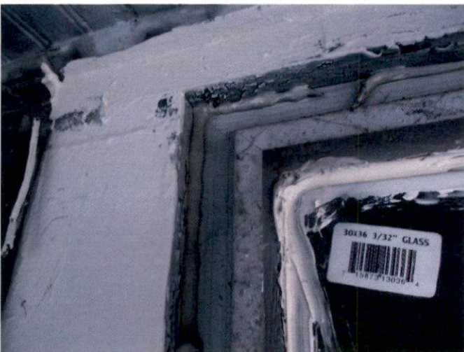
Photo 5 – Gray caulk located around aluminum casing of windows.
