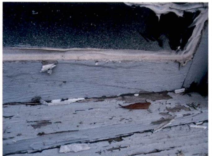
Photo 6 – White caulk located on wooden windows.
