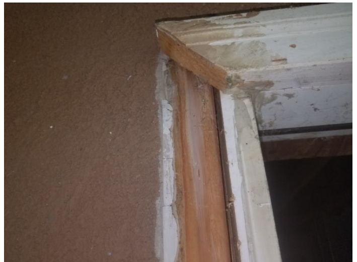
Photo 4 – Caulk located on exterior of door trim.
