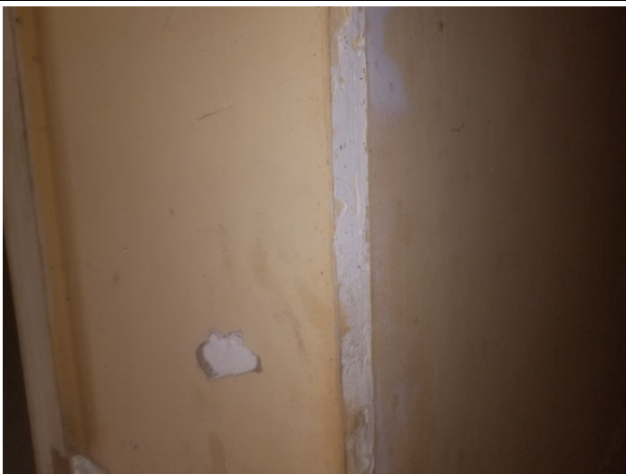
Photo 5 – Drywall sporadically throughout unit walls and ceilings.
