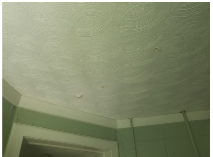
Photo 6 – Swirl ceiling texture in Unit 2, kitchen and hall.
