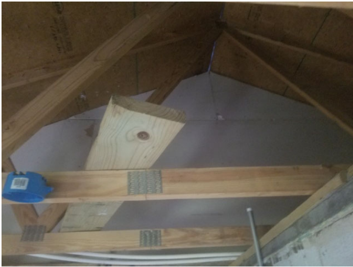
Photo 7 – Unfinished drywall in attic.
