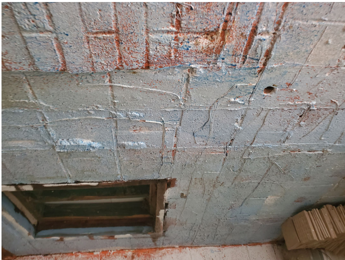
Photo 11 – Hard caulk located in unit 4 laundry room
