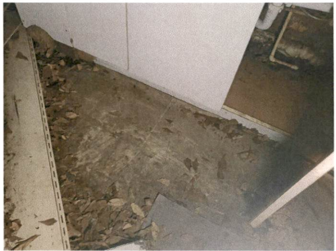
Photo 14 – Tan square pattern roll vinyl patch in front of kitchen sink.
