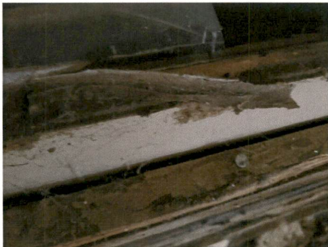
Photo 5 – Interior window caulk found on the living room wood window.
