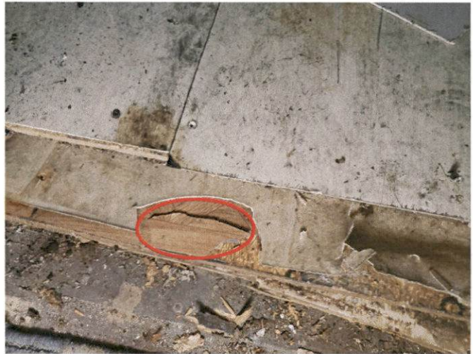
Photo 10 – 12x12 self-stick wood square pattern under cream colored roll vinyl flooring in the bathroom.
