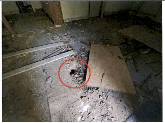
Photo 20 – Hole located inside of entry way into the living room.
