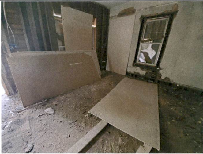
Photo 7 – Unfinished drywall throughout the building.
