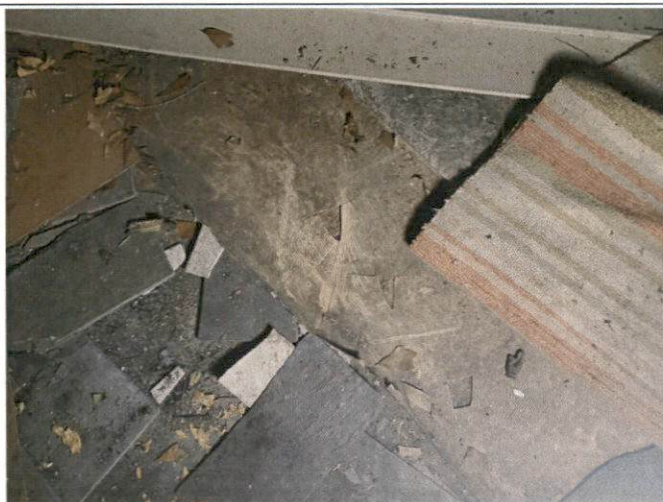
Photo 17 – Tan squared diamond pattern roll vinyl flooring with adhesive located in kitchen.
