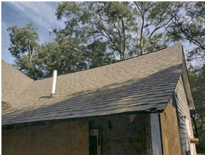
Photo 3 – Two layers of shingles with no felt paper.
