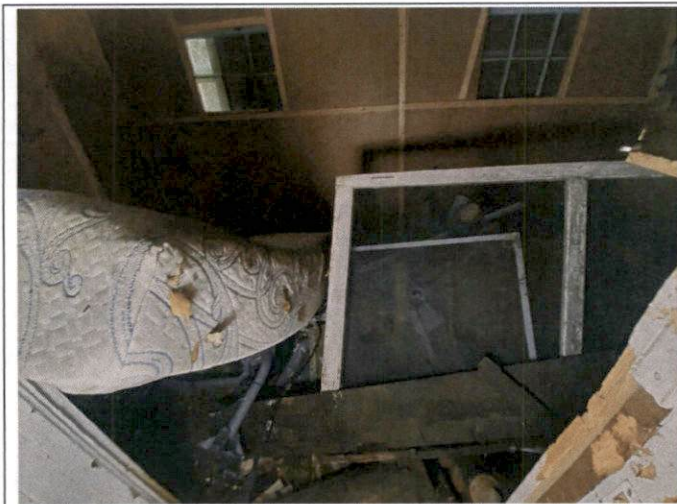
Photo 19 – Household debris located in back room off of the kitchen.
