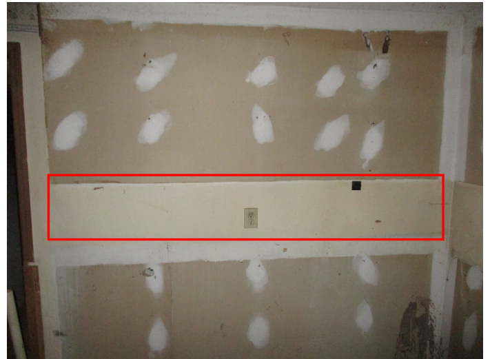
Photo 8 – Beige drywall mud located on ceilings and walls is asbestos containing material.
