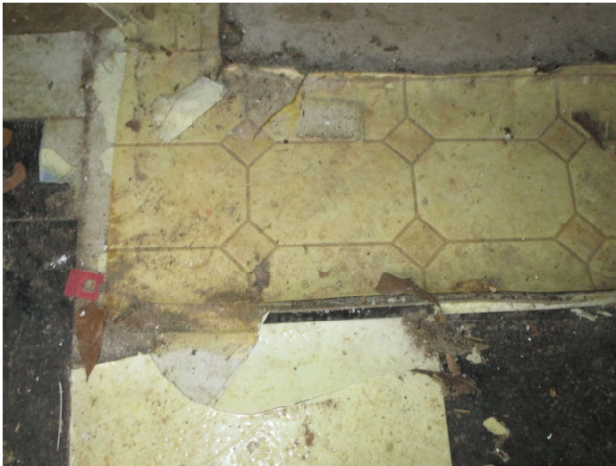
Photo 13 – Tan octagon and diamond roll vinyl floor & mastic located in the kitchen and hallway (2nd layer).
