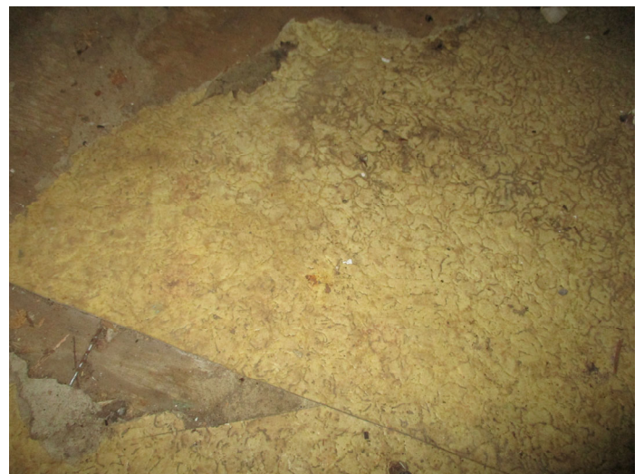
Photo 10 – Tan ripple pattern roll vinyl floor & mastic located in the front right and middle left room.
