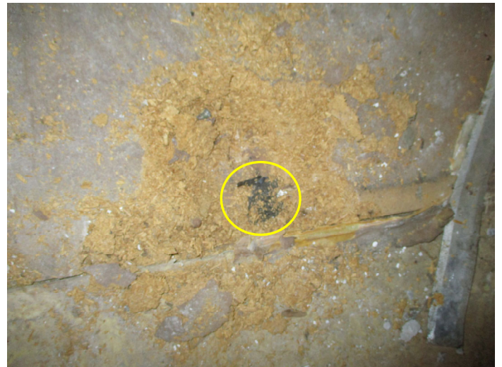
Photo 16 – Black felt paper under top layer of wood floor located in back left room.
