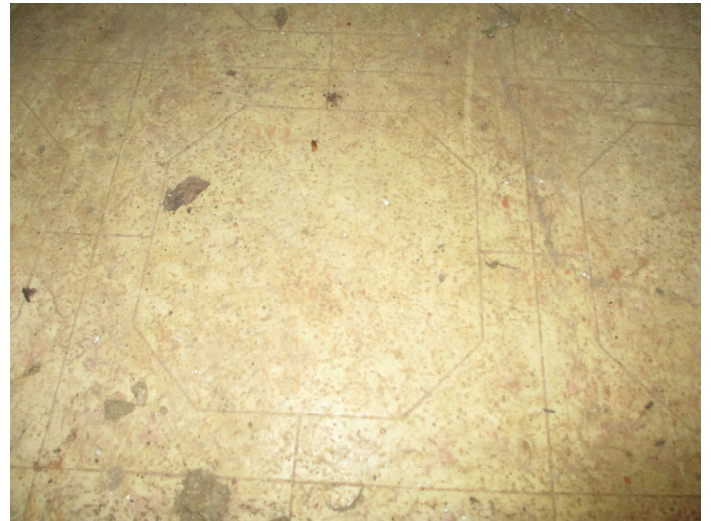
Photo 14 – Large tan square roll vinyl floor & mastic located in the hallway (top layer) and kitchen threshold.
