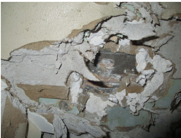
Photo 9 – Second layer of unfinished drywall scattered throughout.
