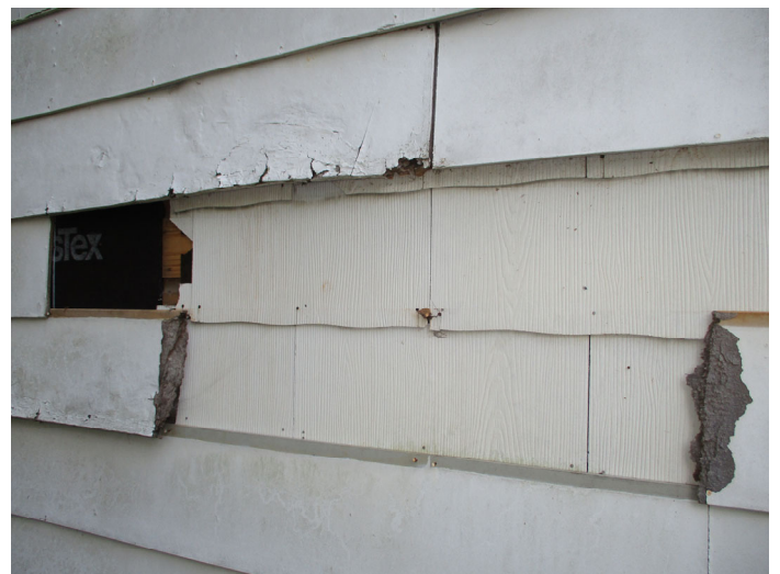
Photo 4 – White transite siding asbestos containing material.
