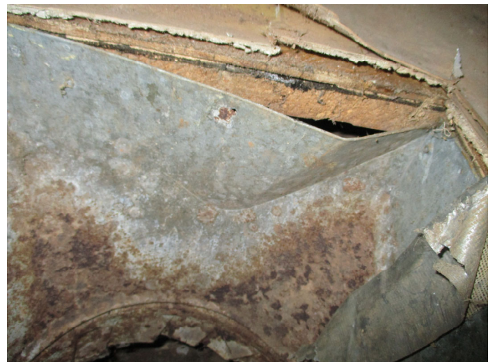
Photo 18 – Brown tile with mastic & black felt under thin layer of wood in hallway.
