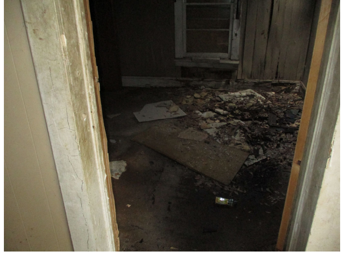
Photo 12 – Building debris throughout.
