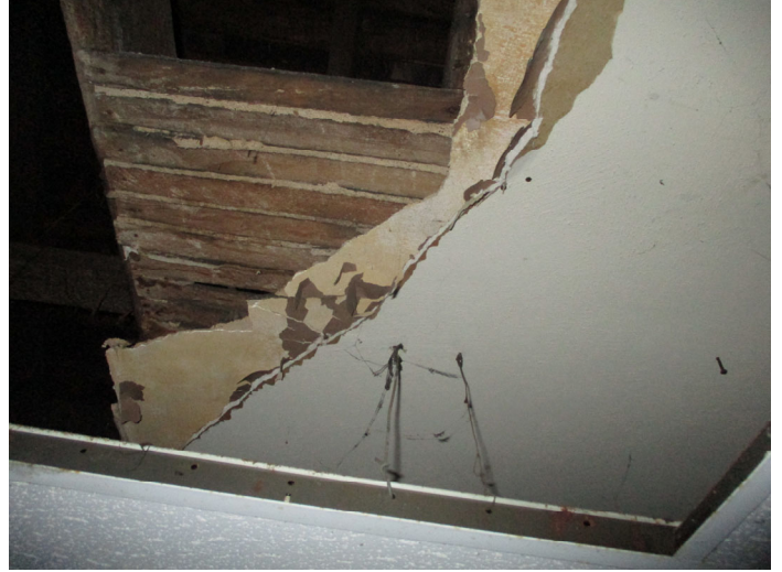
Photo 8 – Plaster on ceiling under 2'x4' ceiling tiles sporadically throughout.
