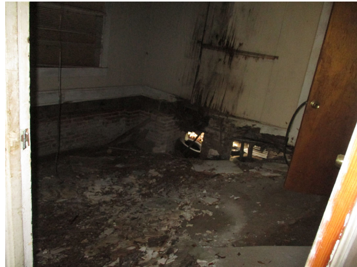
Photo 13 – Structural damage to left rear room. Room was not assessed.
