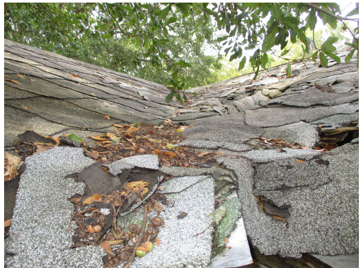
Photo 2 – Four layers of shingles with tar and no felt.
