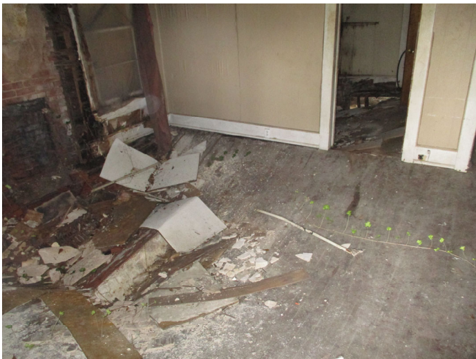
Photo 11 – Structural damage to left front room.
