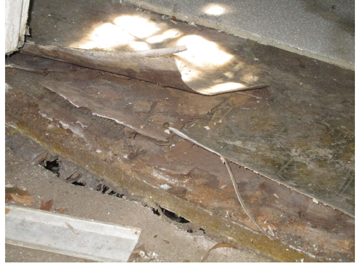
Photo 18 – Vinyl flooring in kitchen inaccessible due to unstable floor.
