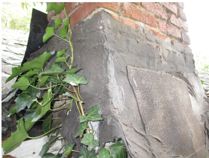
Photo 3 – Tar on chimney.
