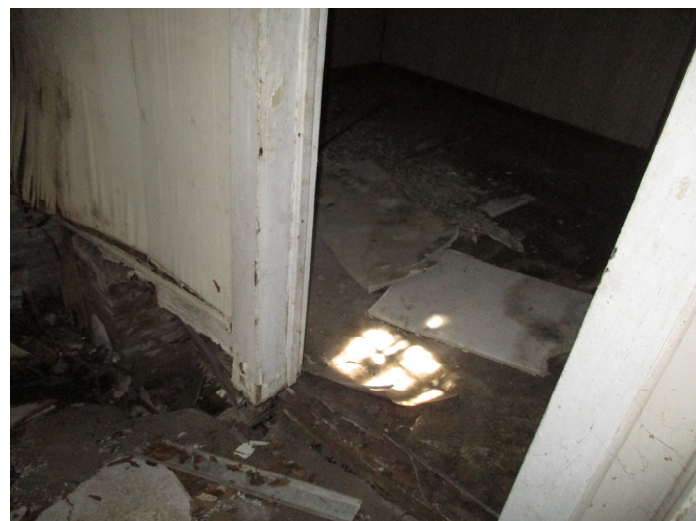
Photo 17 – Damage to floor entering into the kitchen.
