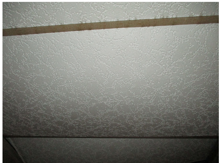
Photo 6 – 2'x4' fissure pattern ceiling tile.
