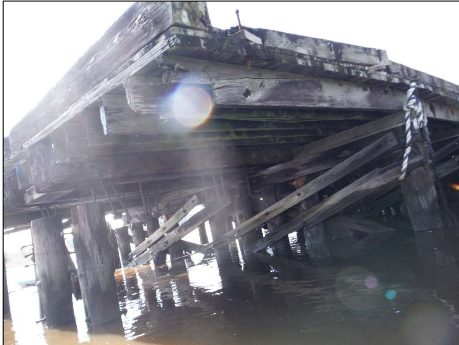
Photograph A 15 – Unsupported Deck at Southeast Corner
