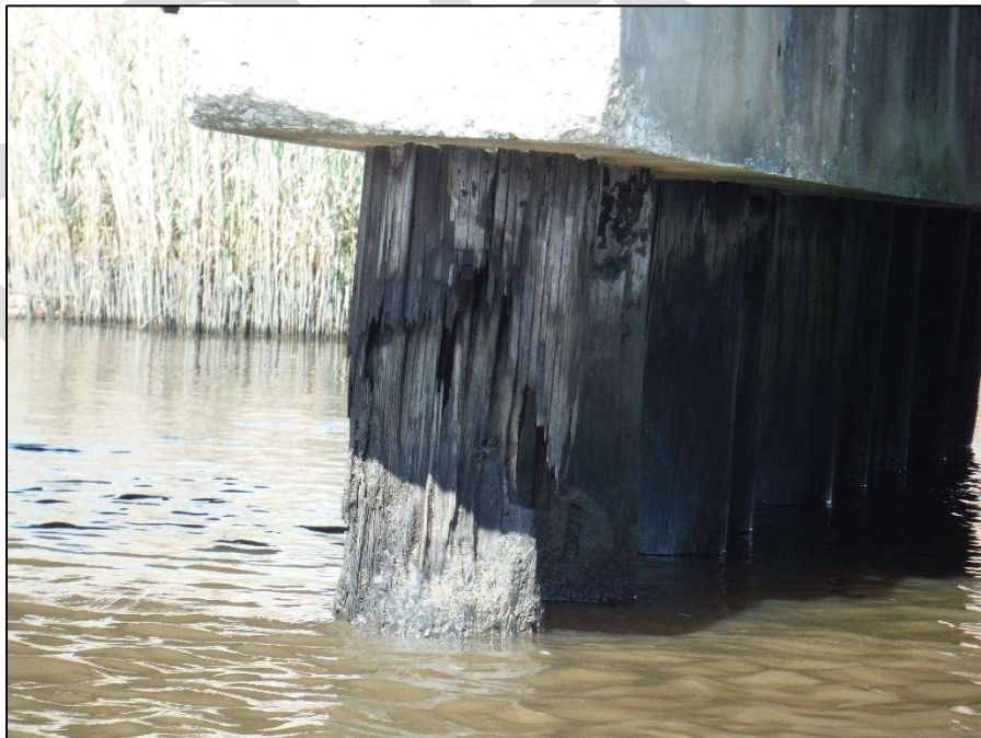
Photograph A 16 – Typical Damaged Pile Above Waterline
