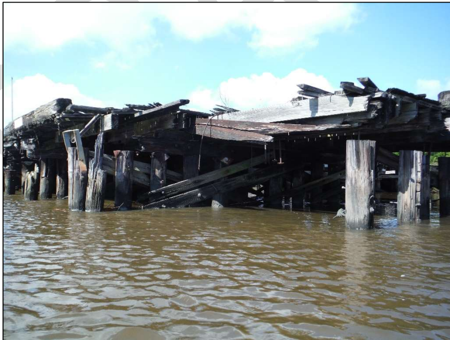
Photograph A 14 – Damaged Southeast Corner
