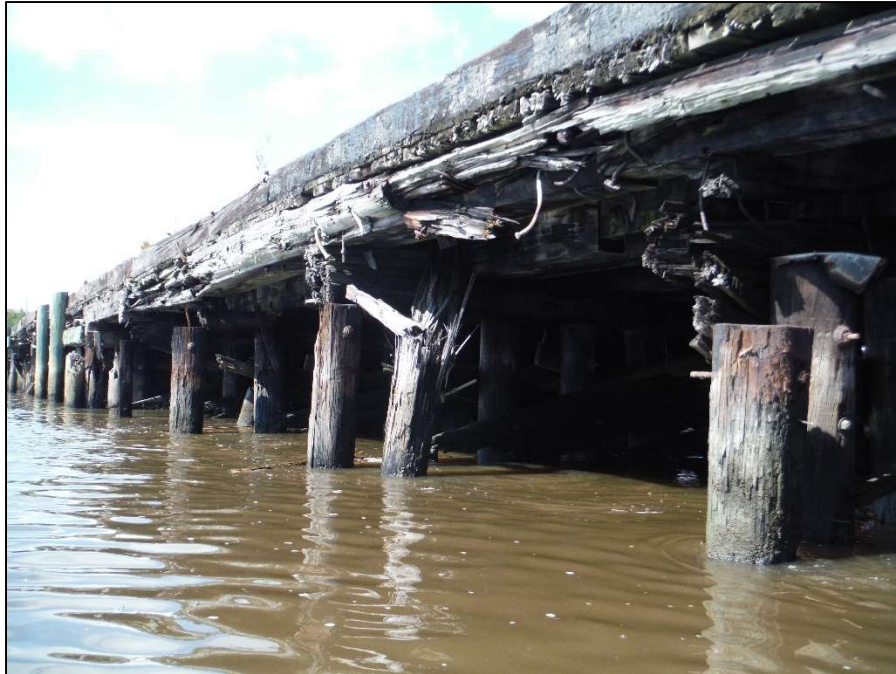
Photograph A 17 – Typical Damage Along Fender System
