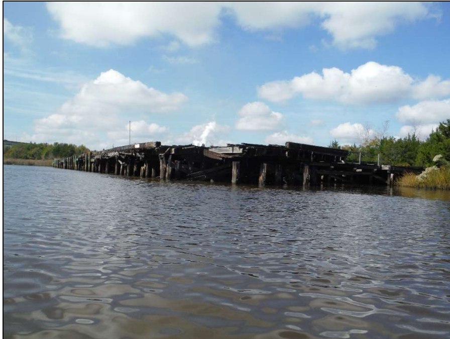
Photograph A 13 – Damaged Southeast Corner
