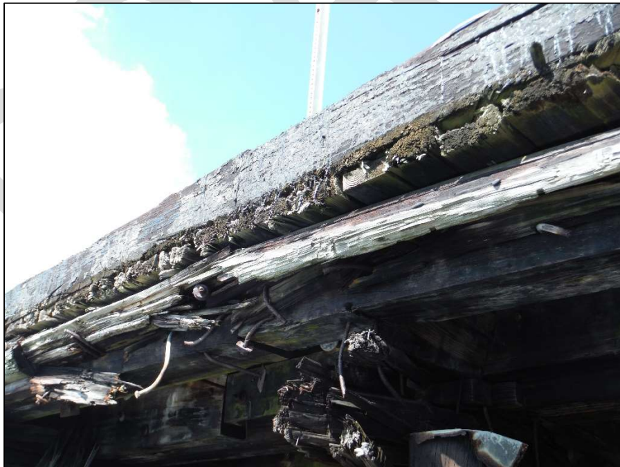
Photograph A 20 – Typical Damage Along Exterior Edge of Deck
