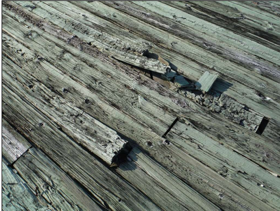
Photograph A 23 – Typical Bowed Deck Boards at Deck
