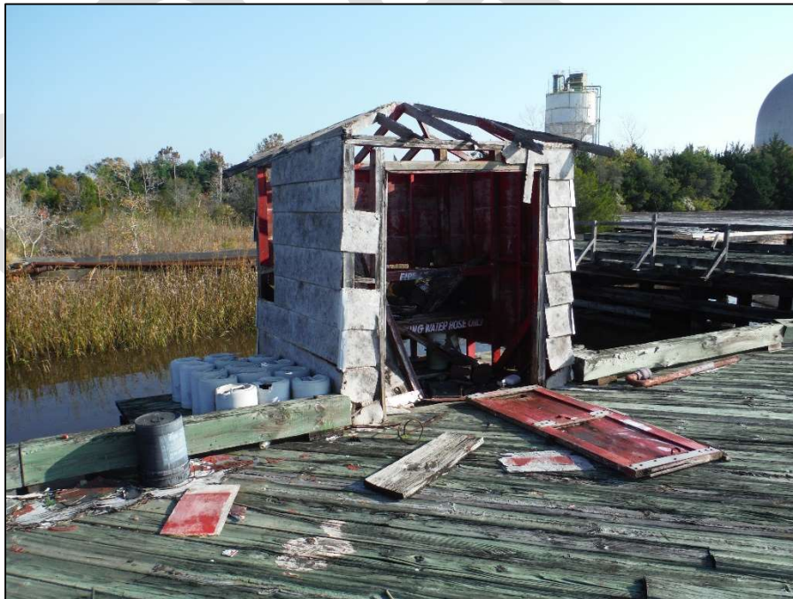
Photograph A 24 – Damaged Supply Shed at North Edge of Relieving Platform
