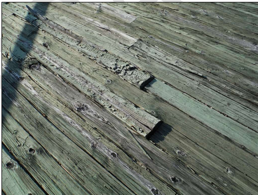
Photograph A 22 – Typical Weathering at Deck
