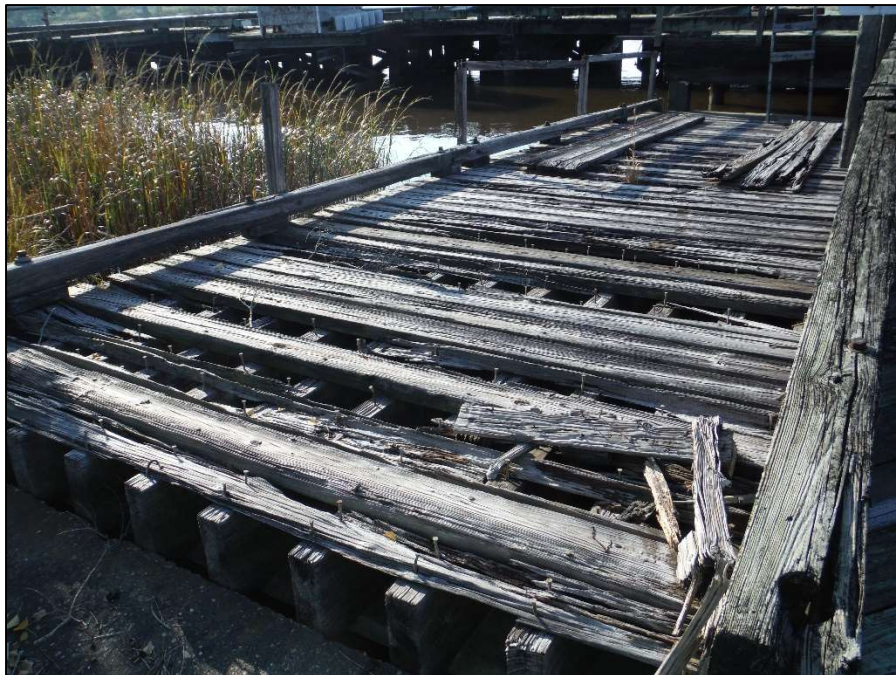
Photograph A 21 – Typical Missing Decking
