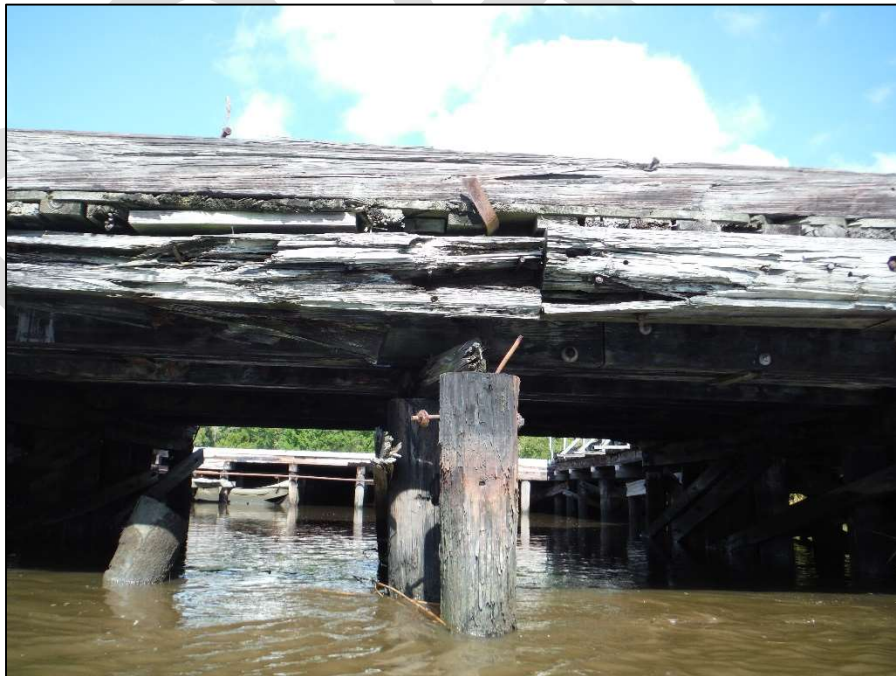
Photograph A 18 – Typical Damaged Fascia Beam at Fender System
