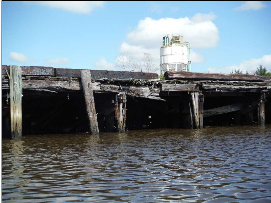
Photograph A 19 – Broken Fascia Beam at Fender System
