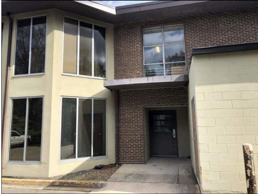
11 - View of Lead Based Paint on a Brown Metal Door. XRF Reading No. 1077.
