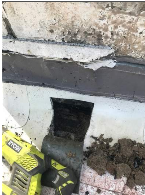
2 - View of Asbestos-Containing Multiple Layered Flashing Caulk on the Connecting Building Parapet Wall. Sample No. 61.
