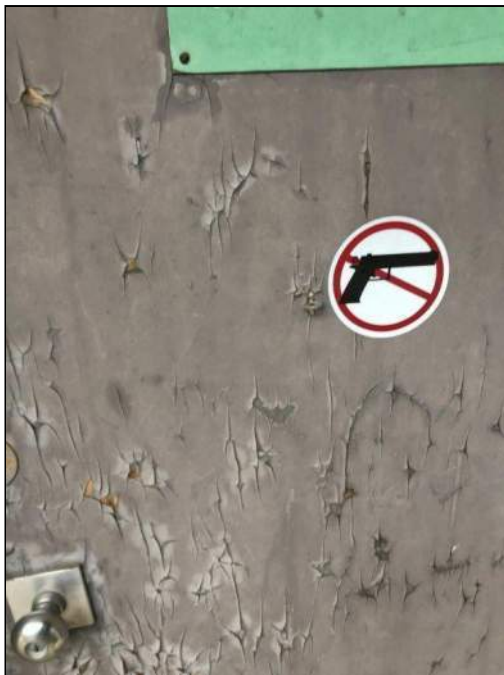
10 - View of Lead Based Paint on a Brown Metal Door. XRF Reading No. 1056.
