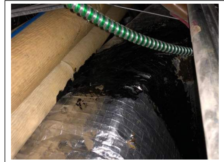
Photo #64 Material: Black Mastic On Foil Duct Sample Result: 5% Chrysotile
