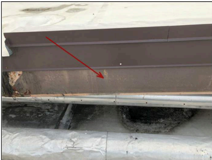
8 - View of Lead Based Paint on a Red Metal Beam on the Roof. XRF Reading No. 1031.
