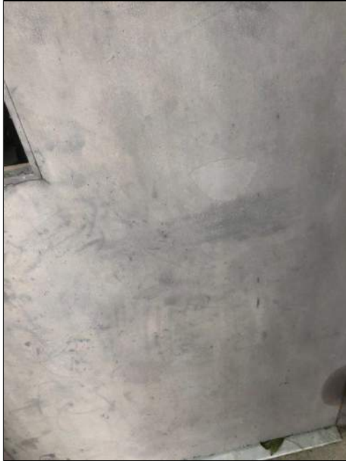
9 - View of Lead Based Paint on a Dark Gray Metal Door. XRF Reading Nos. 1050 and 1051.
