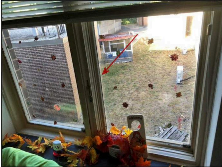
7 - View of Asbestos-Containing Interior Black Window Glazing on Connecting Building Windows. Sample No. 179.
