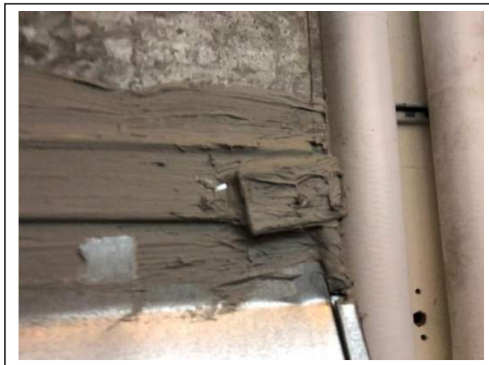
Photo #43 Material: Gray Metal Duct Seam Sealant Sample Result: No Asbestos Detected
