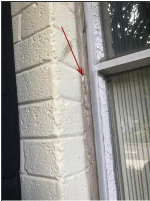
4 - View of Asbestos-Containing White Window Caulk on Exterior Windows. Sample No. 127-B.
