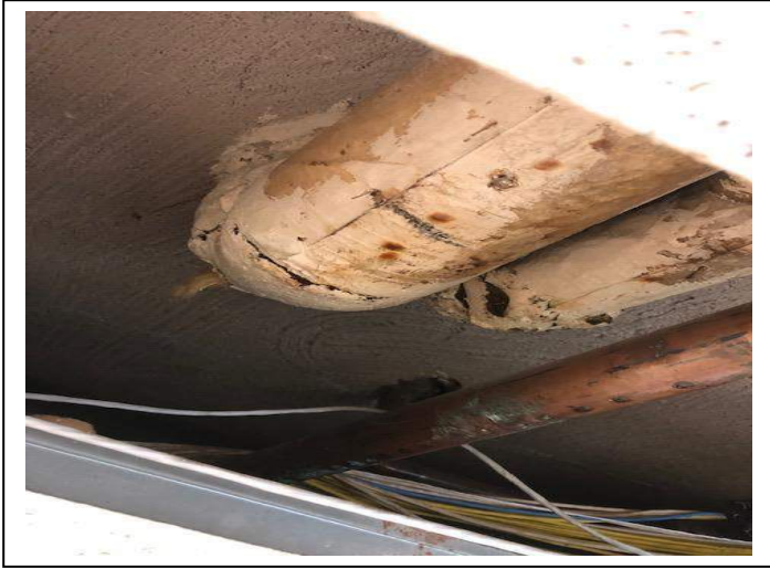
Photo # 25 Material: Muddied Fitting Sample Result: 5% Chrysotile
