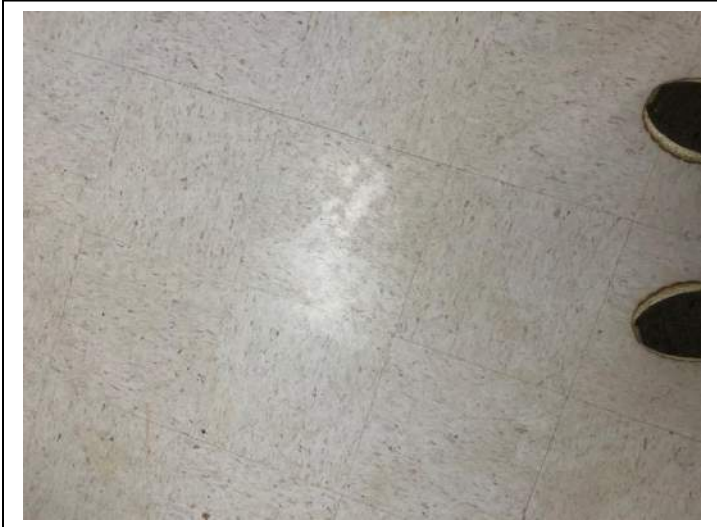
Photo #55 Material: 12"x12" White With Gray Specks Floor Tile Sample Result: No Asbestos Detected
