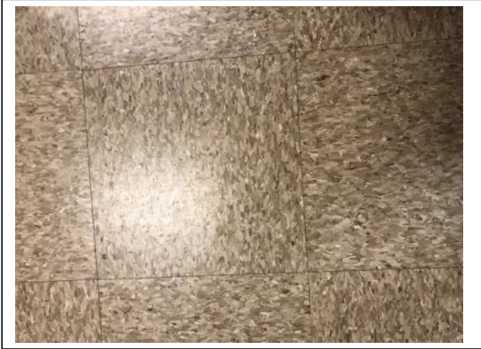
Photo #5 Material: 12"x12" Tan Mottled Floor Tile Sample Result: No Asbestos Detected
