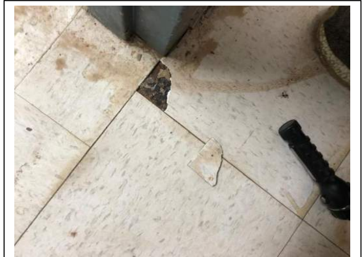
Photo #10 Material: 12"X12" White With Black Streaks Sample Result: No Asbestos Detected
