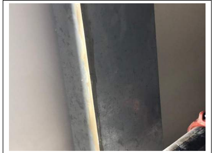
Photo #14 Material: Brown Metal Duct Seam Sealant On Metal Sample Result: No Asbestos Detected
