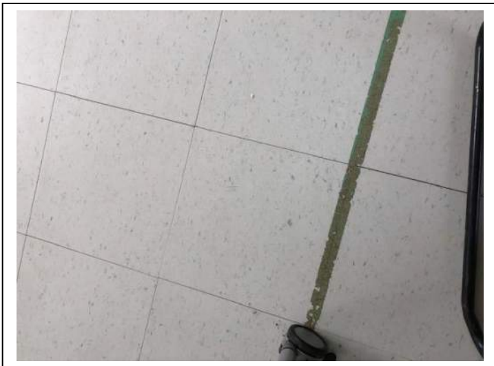
Photo #51 Material: 12"x12" White With Green Specks Floor Tile Sample Result: No Asbestos Detected
