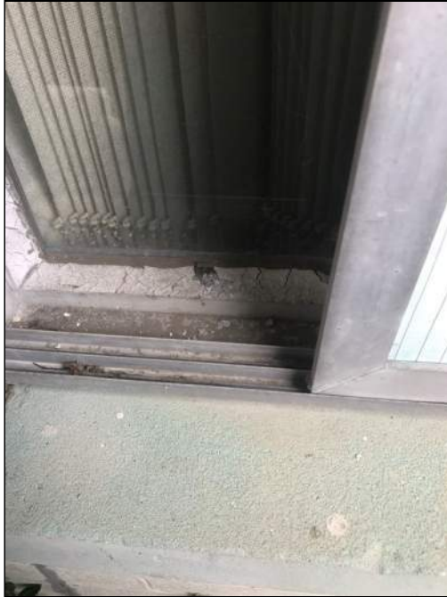
3 - View of Asbestos-Containing Gray Window Glaze on Exterior Windows. Sample No. 125.
