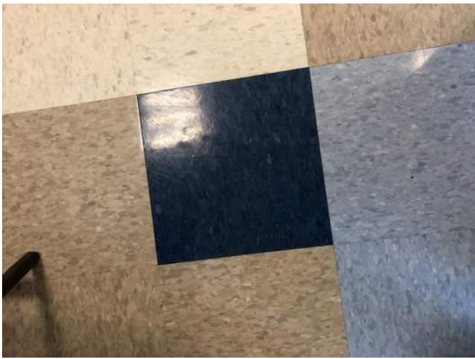
Photo #71 Material: 12"x12" Dark Blue Mottled Sample Result: No Asbestos Detected
