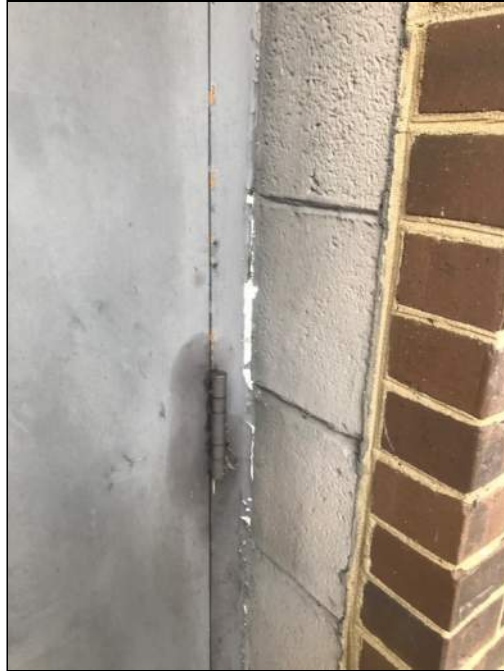
5 - View of Asbestos-Containing Tan Door Caulk on Exterior Doors. Sample No. 149.
