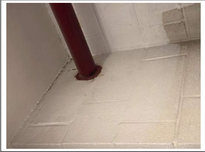
Photo #81 Material: Red Fire Stop Sample Result: No Asbestos Detected
