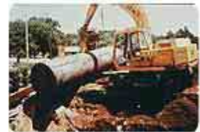
A former industrial site located near a residential area which caused a vapor intrusion issue.
