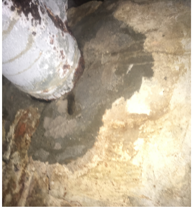
Pos. Stack Cement
