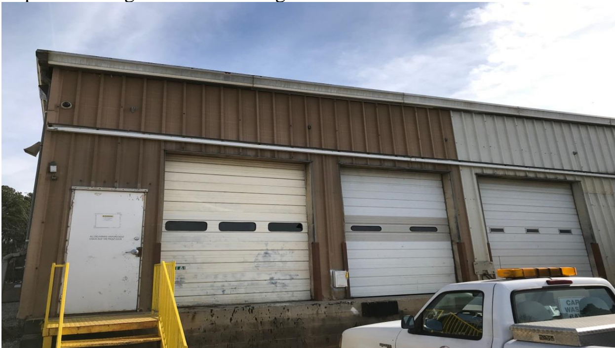
Clean and paint block wall below roll up doors rear of building
