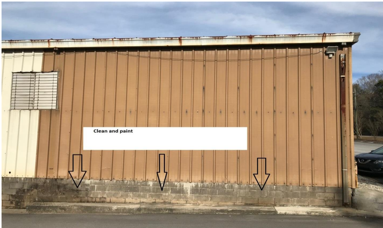
Fleet service side of building . Note rusted gutters and 2 tone metal panels . Clean and paint concrete base
