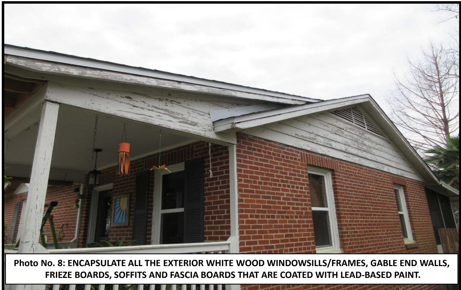
Photo No. 7: ENCAPSULATE ALL EXTERIOR WHITE WOOD WINDOWSILLS/FRAMES, GABLE END WALLS, FRIEZE BOARDS, SOFFITS AND FASCIA BOARDS THAT ARE COATED WITH LEAD-BASED PAINT.
