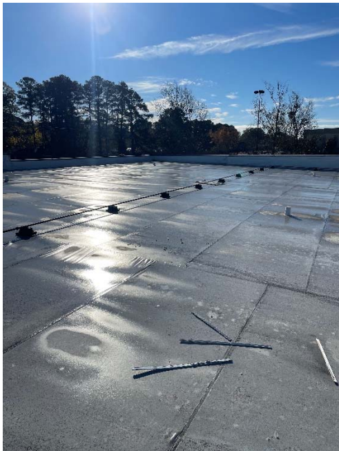
General view of the roof of the commercial structure on the Subject Property
