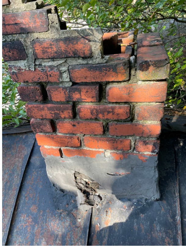
View of asbestos-containing Black Chimney Tar (HA 929-3)
