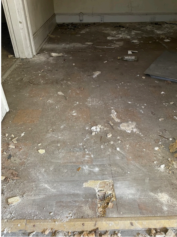
General view of asbestos-containing Tan Floor Tile (HA 209-6)
