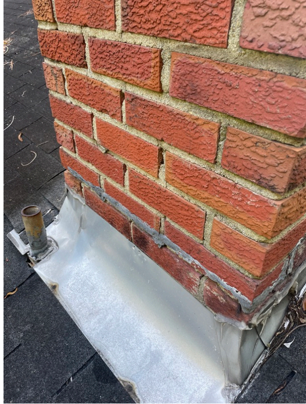
View of asbestos-containing Black Chimney Tar (HA 1419-7)
