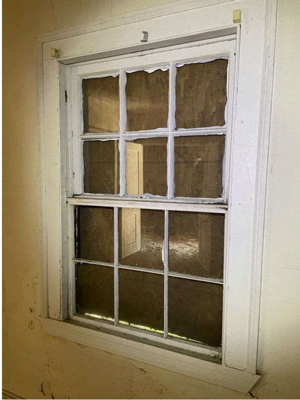
View of trace asbestos-containing White Exterior Window Glazing (HA 209-4)
