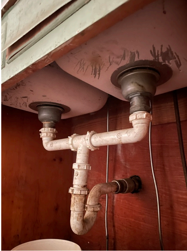
View of asbestos-containing White Sink Coating (HA 1419-5)
