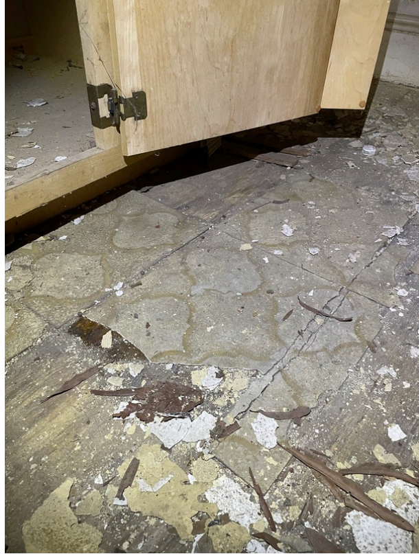
View of asbestos-containing 12" x 12" Tan Floor Tile (HA 209-5)
