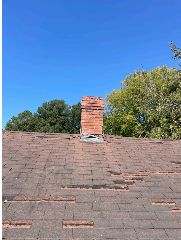
View of asbestos-containing Gray/Black Chimney Caulk (HA 209-9)
