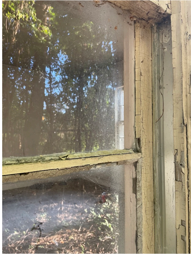
View of trace asbestos-containing White Exterior Window Glazing (HA 1419-1)
