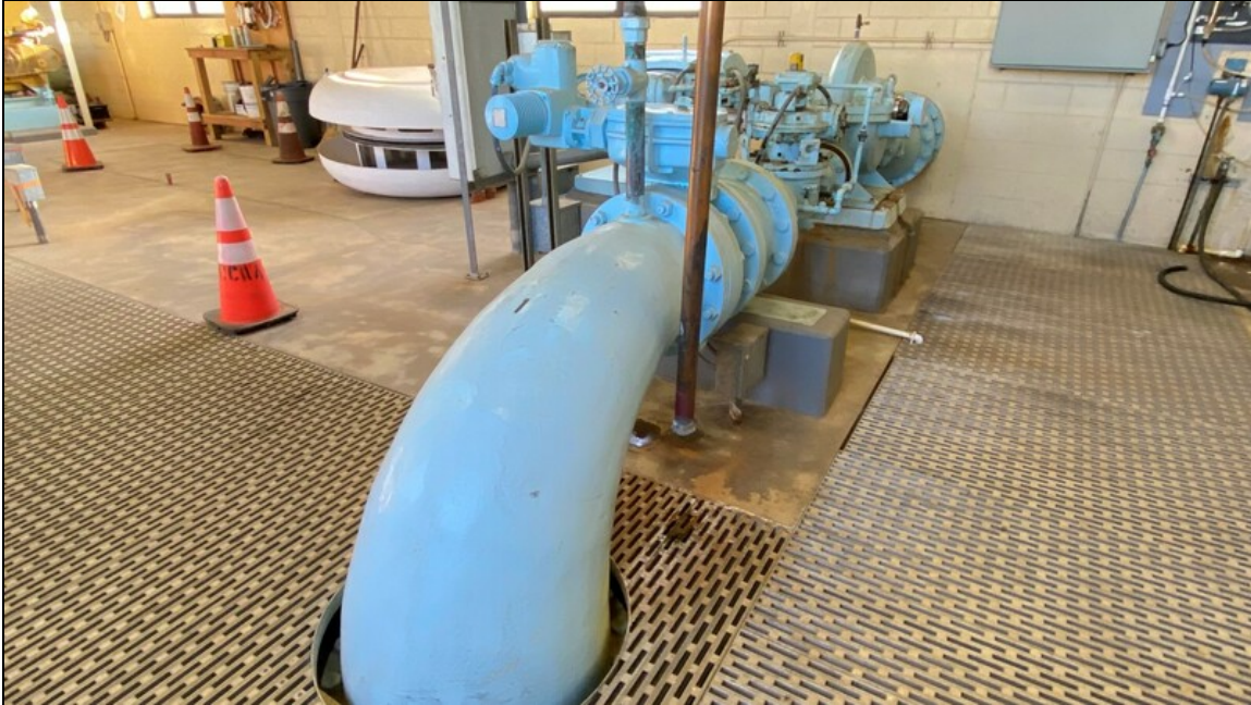
3 - View of blue paint on pipes
