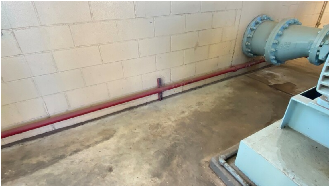
4 - View of red paint on pipes and blue paint on base of equipment
