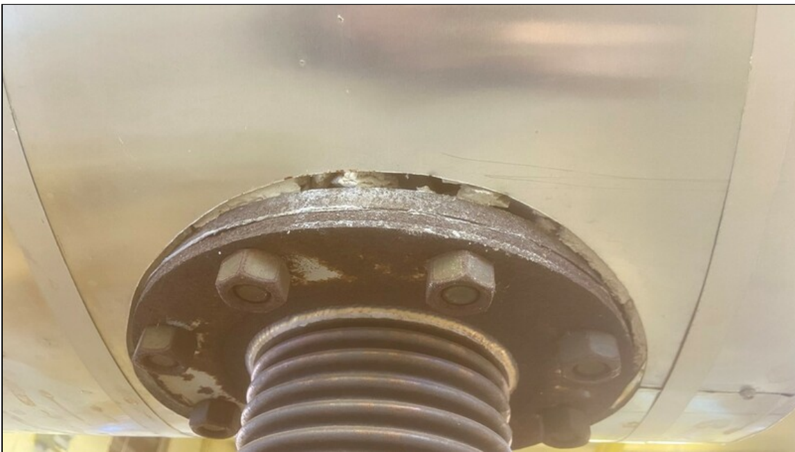
6 - View of the tank insulation
