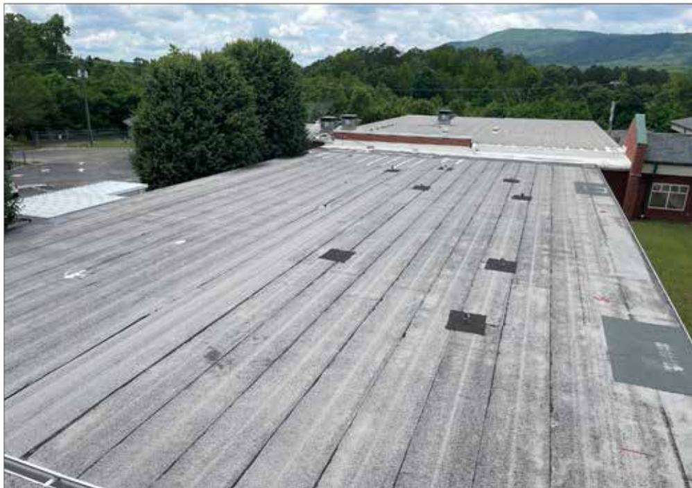
This is an overview of the Modified Roof System that was scanned.
