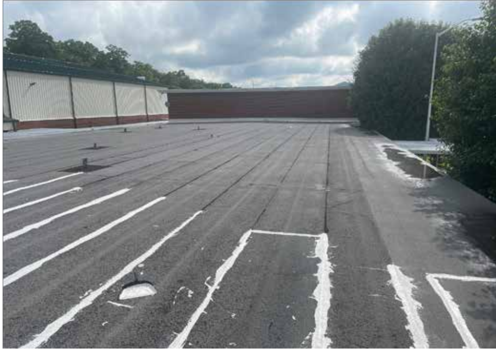
This is an overview of the Modified Roof System that was scanned.
