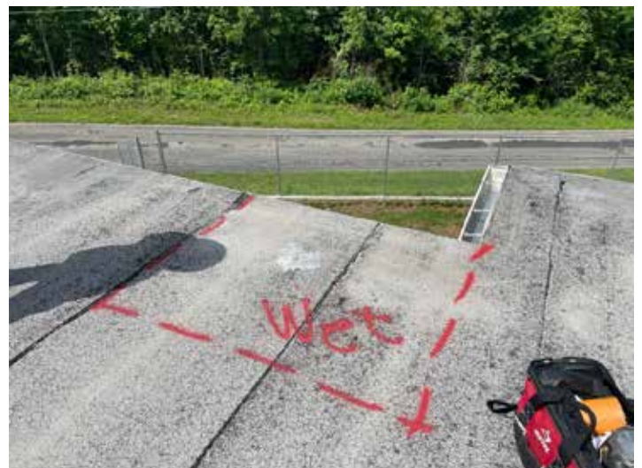
Wet areas were marked on the roof and represented on the roof plan in this report.
