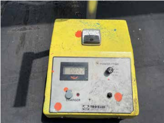
Elevated reading on the EPDM section.
