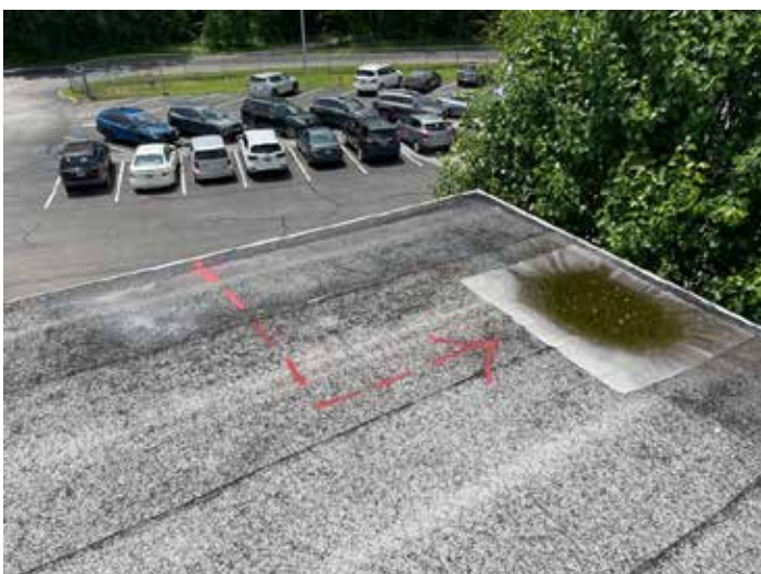
Wet area discovered. Potential damaged decking.
