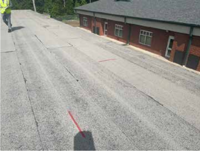
A 10'x10' grid was painted on the roof to properly record the readings on the nuclear gauge.
