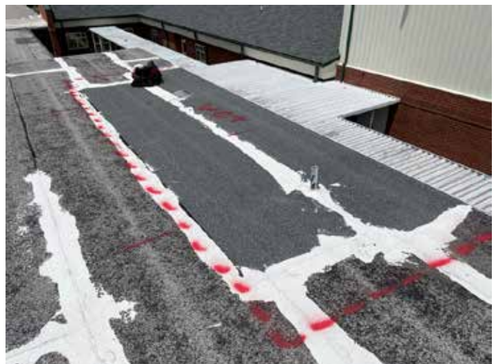
Wet areas were marked on the roof and represented on the roof plan in this report.
