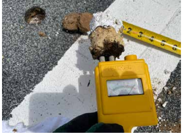
Delmhorst reading at the nuclear reading of 13. This core was taken on the cafeteria, upper roof section.
