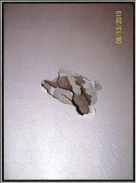
Photo #17 No Asbestos Detected in Cementitious Board and Sheetrock Combination Wall System
