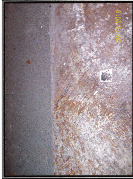
Photo #3 Asbestos Detected at >1% in Tan Floor Tiles under Parquet Sheet Flooring at Counter Area
