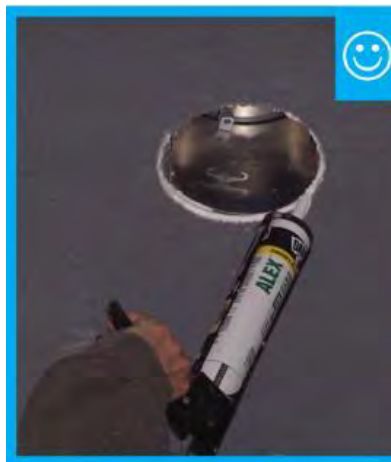
Caulk around all penetrations in drywall at attic, including lighting and ductwork
