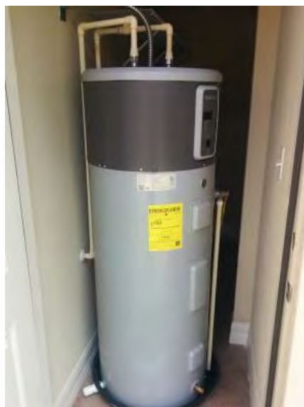
Electric Storage Tank
