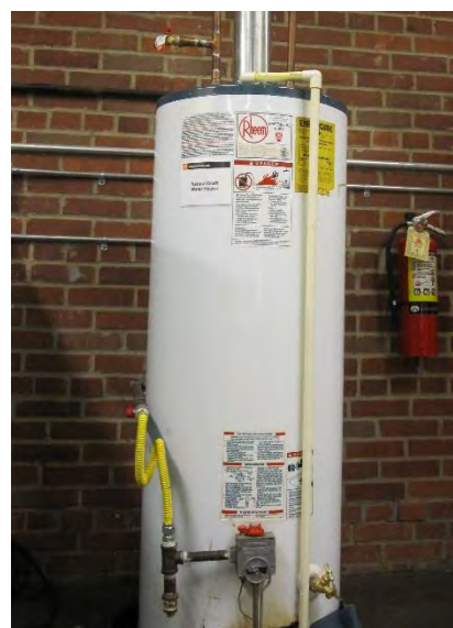
Gas Storage Tank
