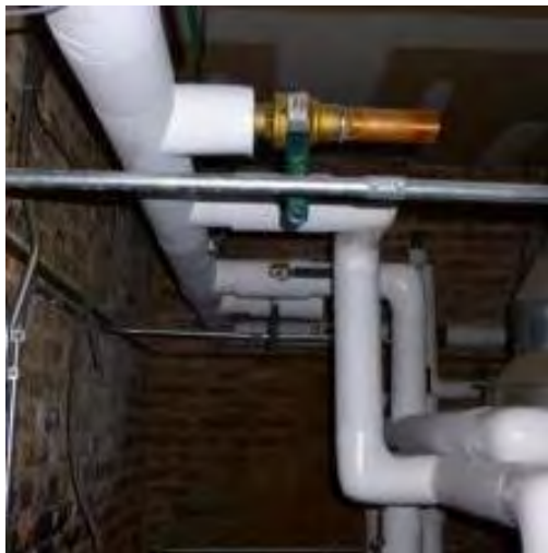
Insulate 100% of hot water pipe
