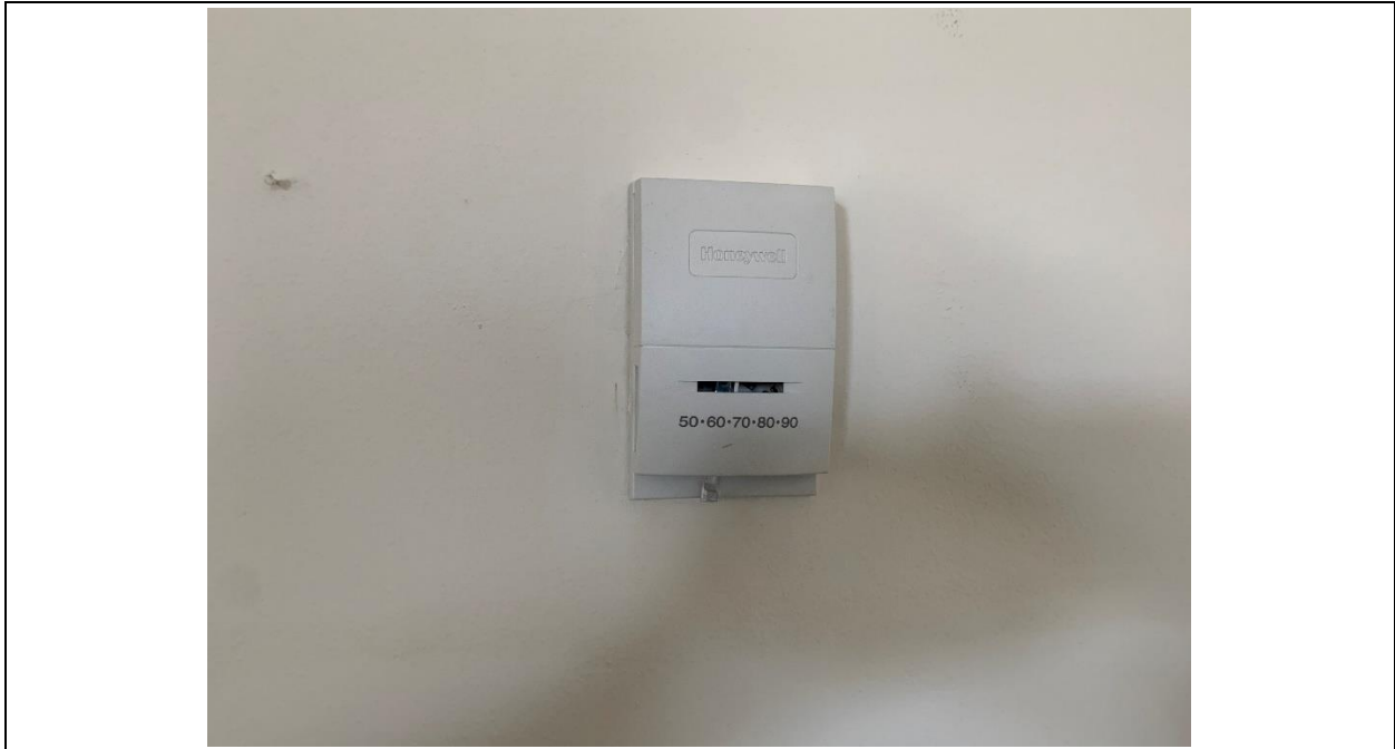
Mercury Thermostat in Living Room
