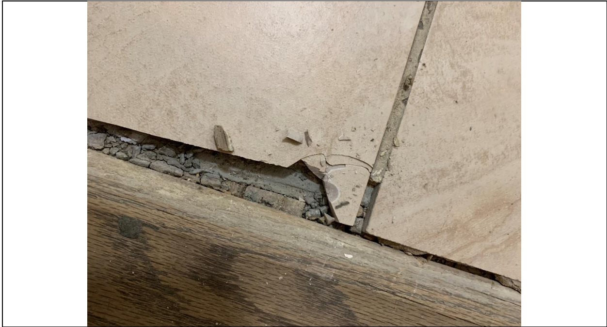
Homogeneous Material No. 11 – Non-ACM Pinkish Gray CT with Gray Grout and Gray Setting Base located in the Shower Room on the 1 st Floor
