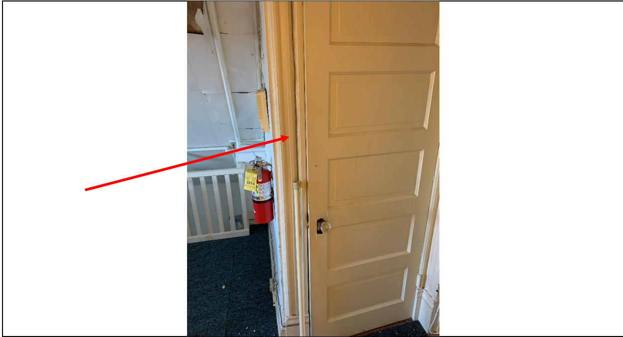
LBP-11: Lead-Based Paint on Closet Door Casing, Landing on 3 rd Floor
