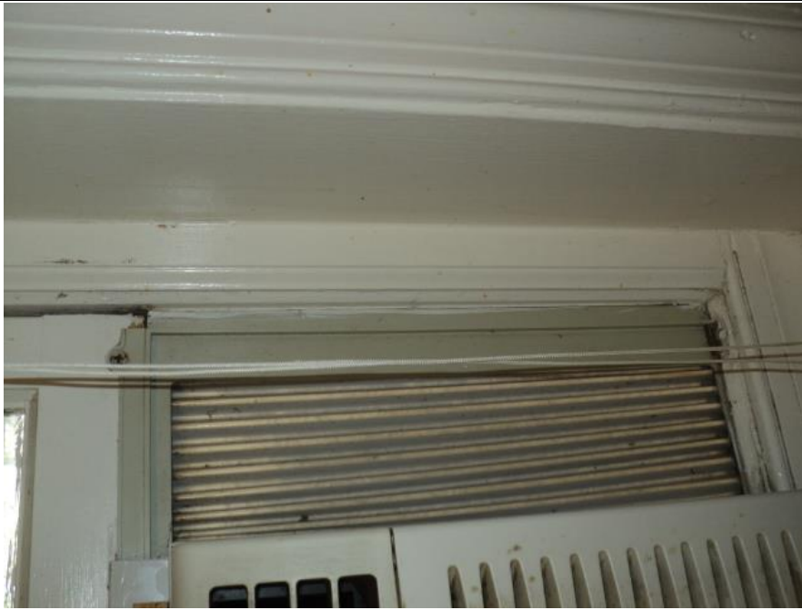
Homogeneous Material No. 5 – Non-ACM White Interior Window Caulk located in the Kitchen and Bedroom 1-3
