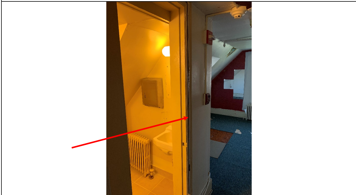
LBP-10: Lead-Based Paint on Door Casing in Bathroom on 3 rd Floor
