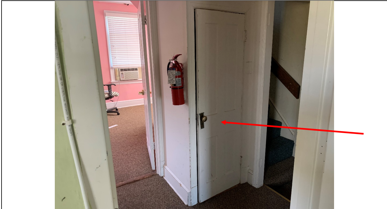
LBP-7: Lead-Based Paint on Closet Door in Landing Area (2 nd Floor)
