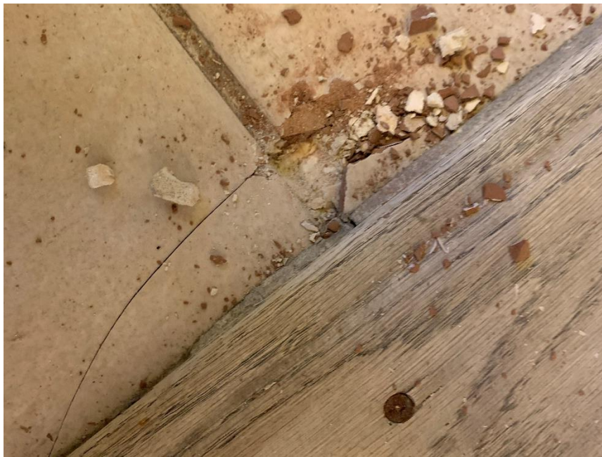
Homogeneous Material No. 10 – Non-ACM Mottled Pink CT with Light Gray Grout and White Setting Base located in the Bathroom on the 1 st Floor
