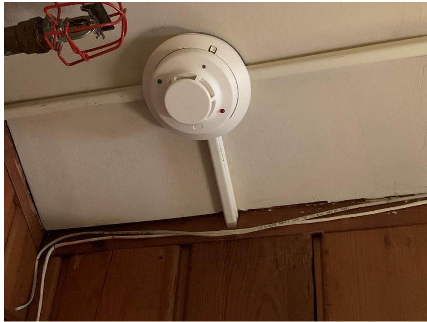
Typical Smoke Detector Throughout the Subject Property
