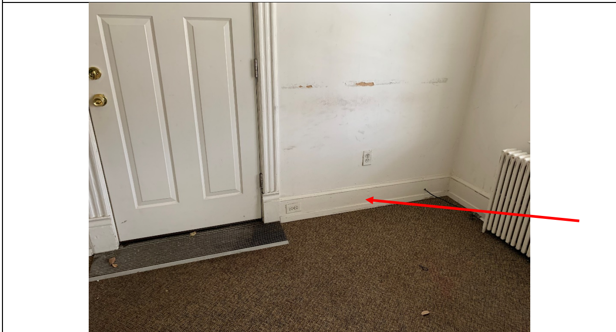
LBP-6: Lead-Based Paint on Baseboard in Living Room
