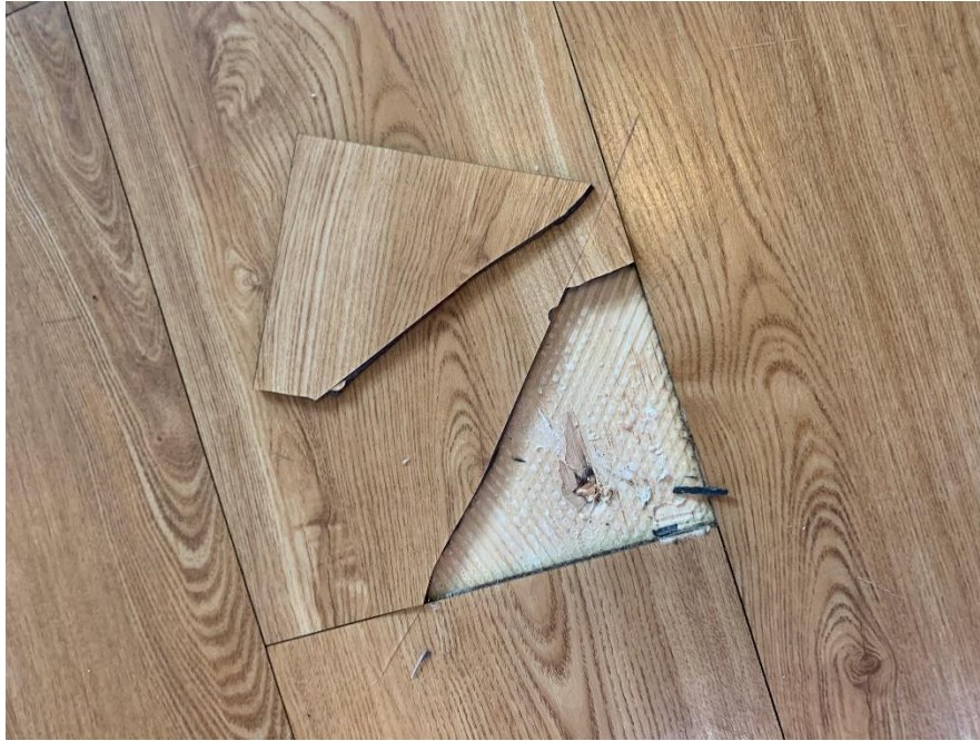
Homogeneous Material No. 9 – Non-ACM Tan Faux Wood Pattern Vinyl Plank Flooring with Cream Mastic located in Bedroom 1-2 and Bedroom 1-3
