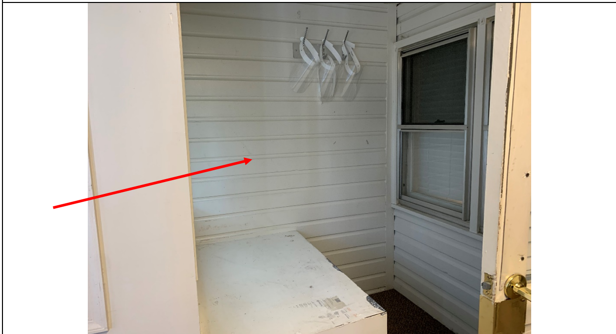
LBP-4: Lead-Based Paint on Siding/Paneling in the Office Area
