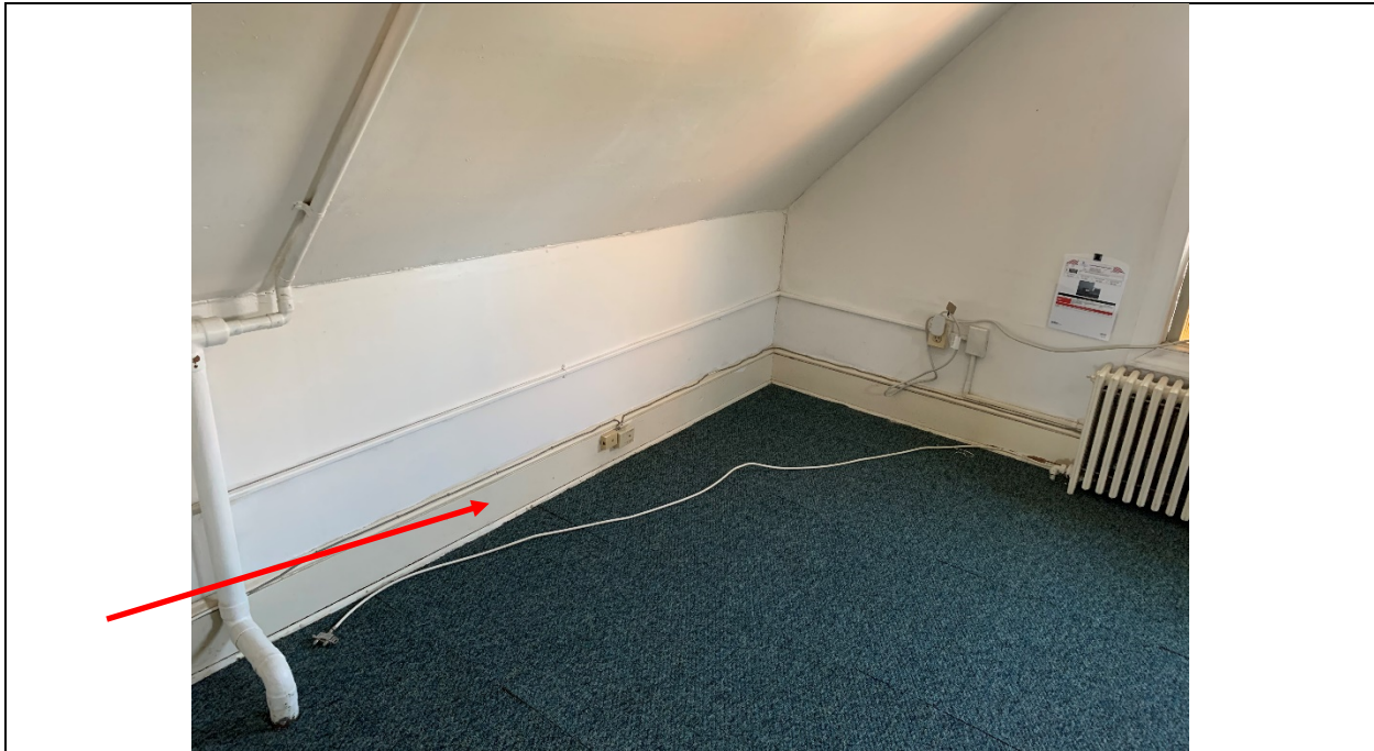
LBP-13: Lead-Based Paint on Baseboard in Bedroom 3-1 on 3 rd Floor
