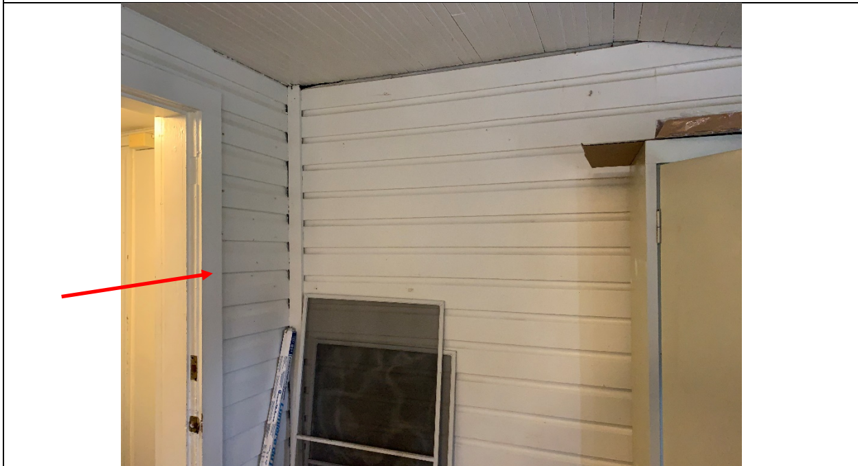
LBP-2: Lead-Based Paint on Casing on Door Leading to Office from Living Room/Dining Room
