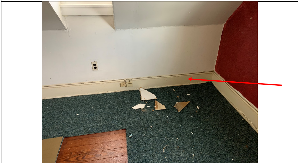
LBP-8: Lead-Based Paint on Baseboard in Bedroom 3-2 (3 rd Floor)
