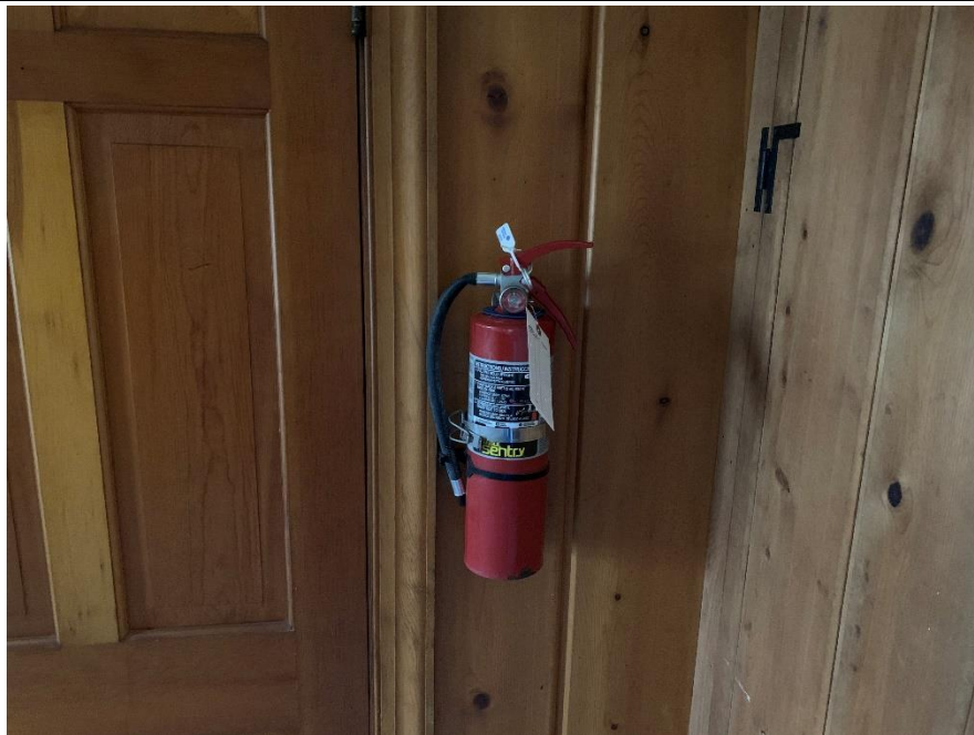
Typical Fire Extinguisher Throughout the Subject Property
