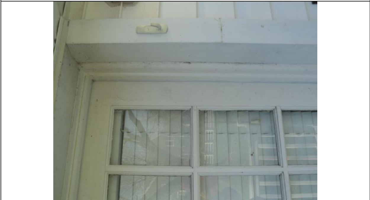
Homogeneous Material No. 16 – Non-ACM White Exterior Door Caulk located on the Exterior Door
