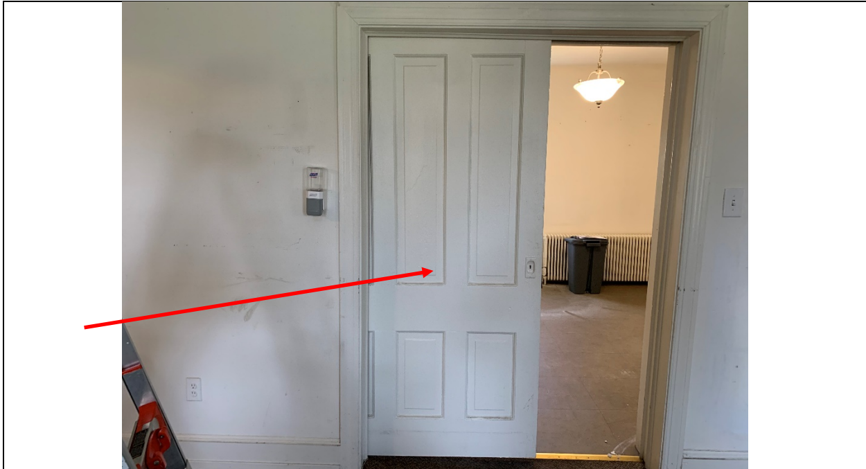
LBP-5: Lead-Based Paint on Pocket Door Separating Living Room and Dining Room
