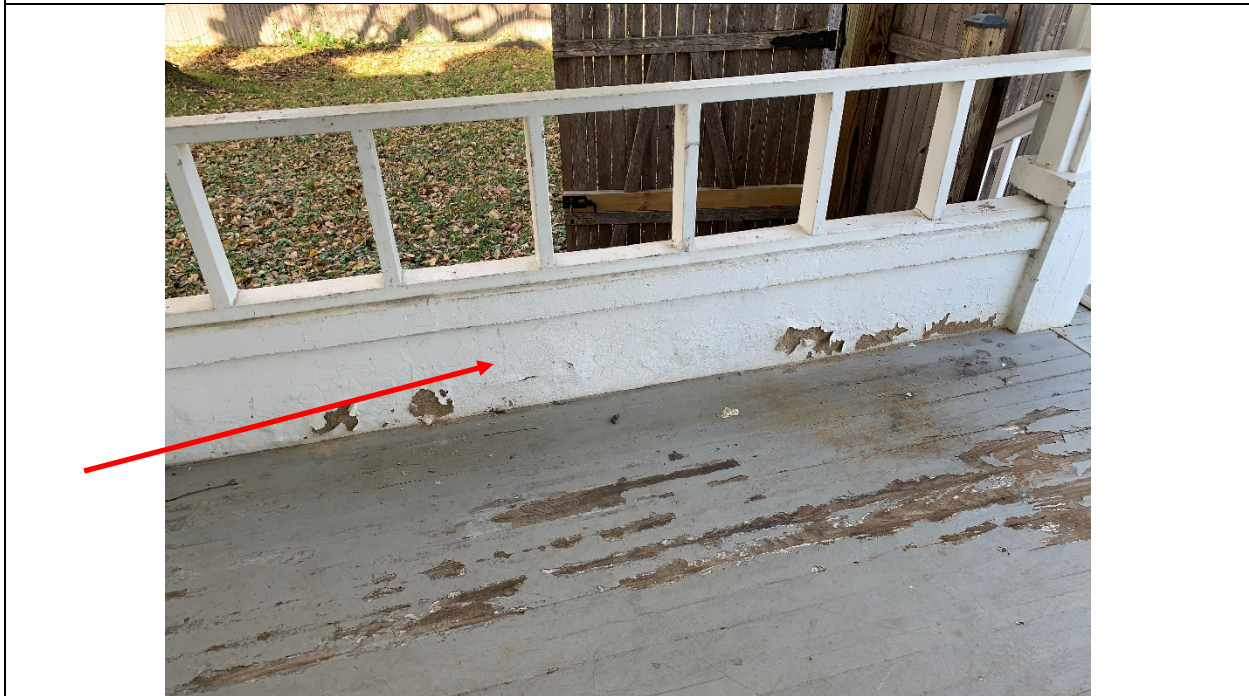
LBP-14: Lead-Based Paint on Concrete Knee Wall in Landing Area of Entrance to Property
