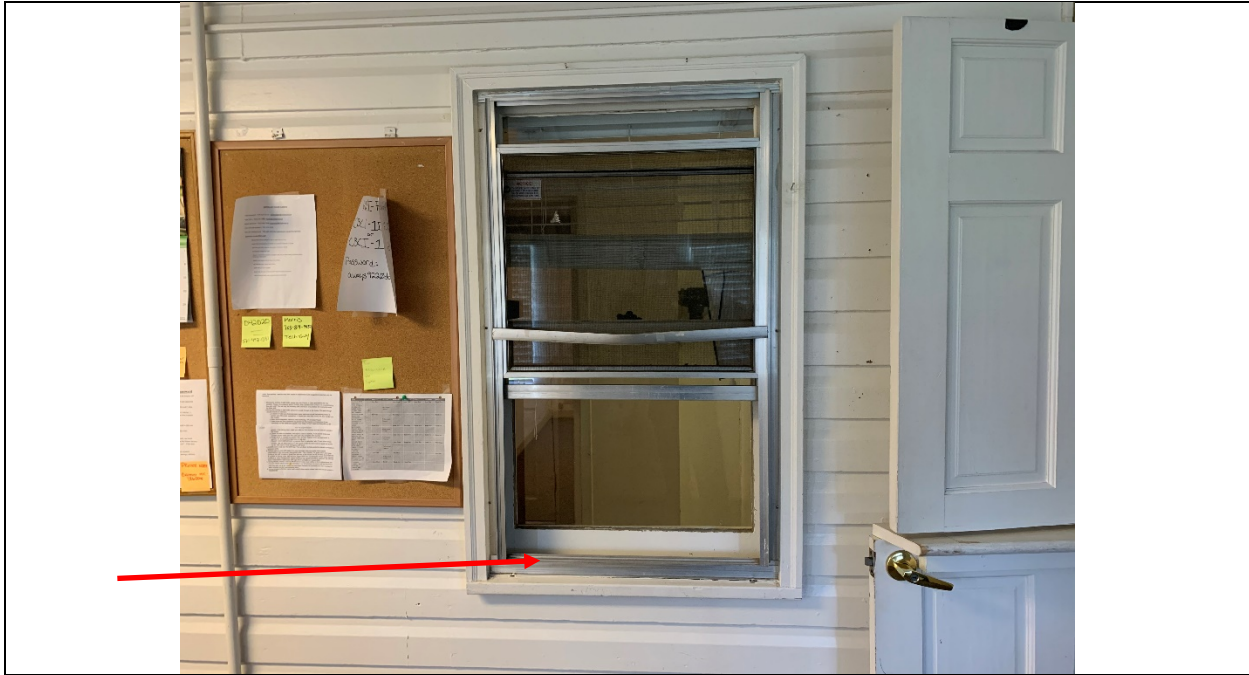
LBP-3: Lead-Based Paint on Window Sash, Window Casing, Windowsill & Window Trough in the Office
