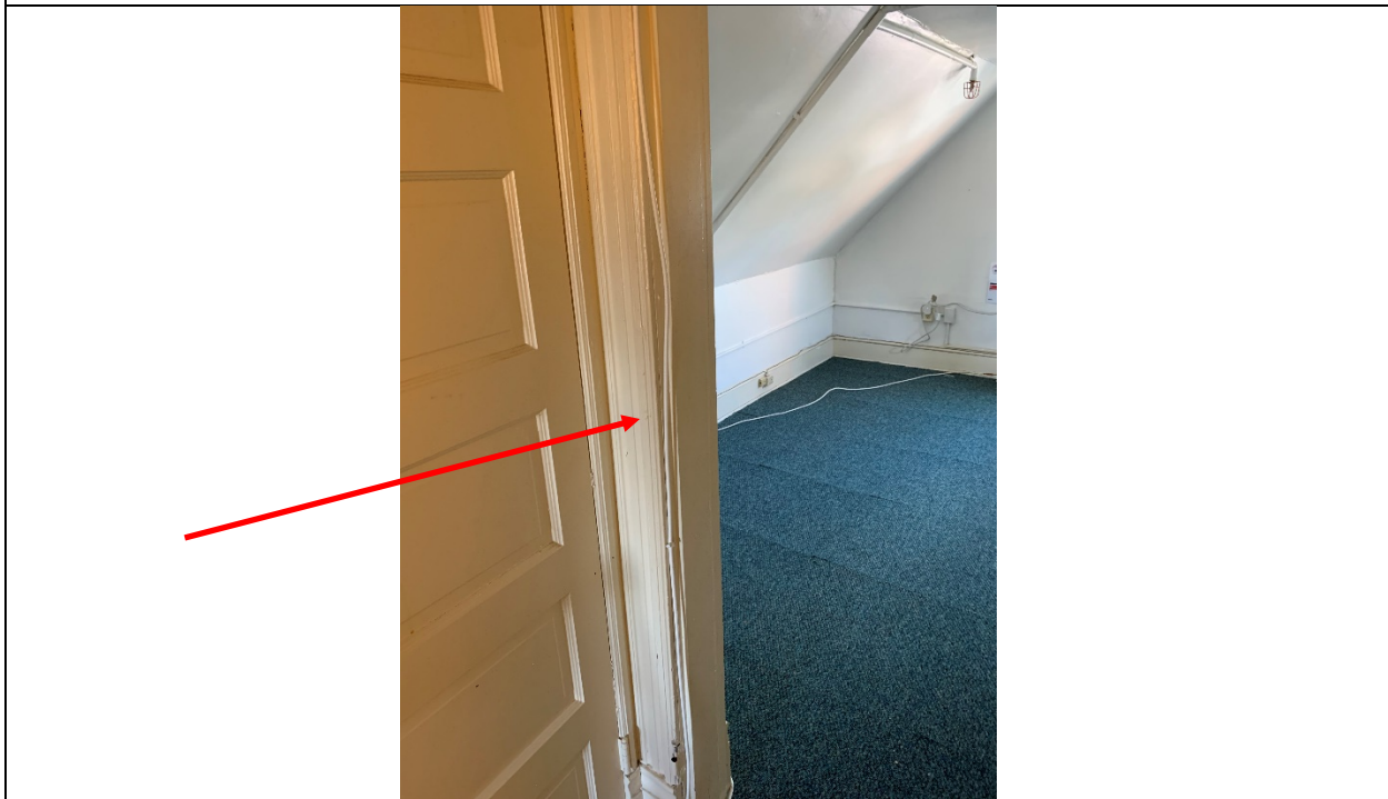
LBP-12: Lead-Based Paint on Door Casing Leading to Bedroom 3-1 on 3 rd Floor
