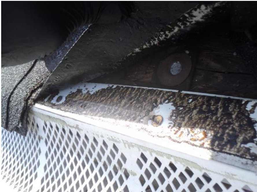
Homogeneous Material No. 18 – Non-ACM Black asphalt roof shingle with Black Asphalt Ice Shield and Black Felt Paper located on the Roof
