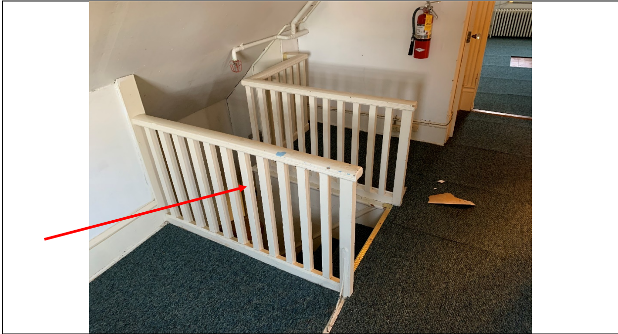
LBP-9: Lead-Based Paint on Handrail and Rail Spindle, Stairway to 3 rd Floor Area
