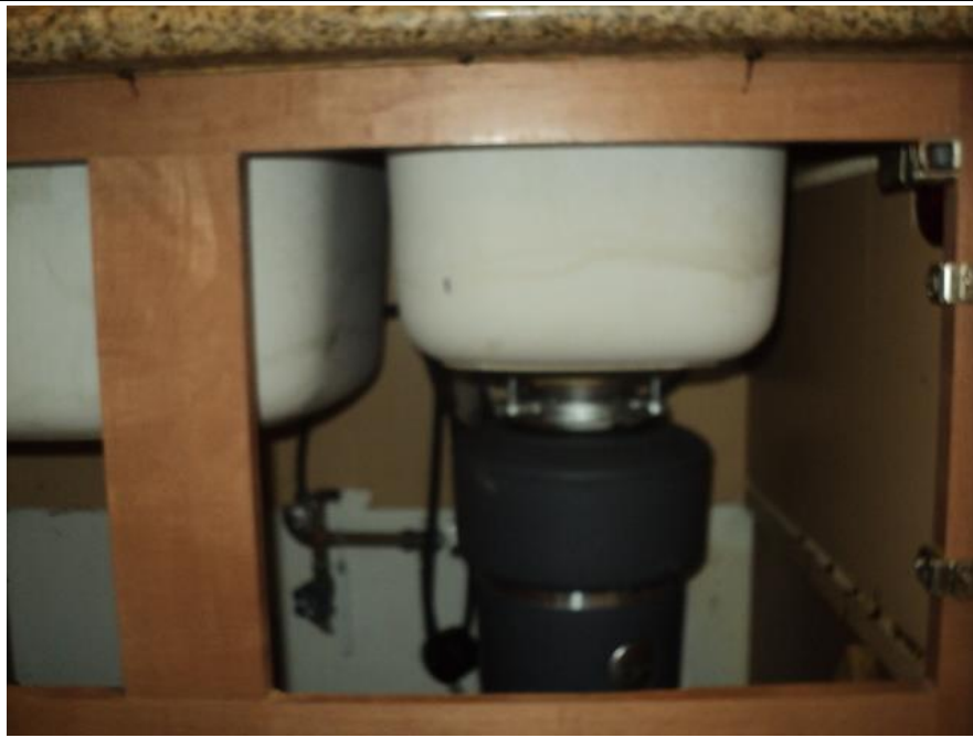
Homogeneous Material No. 7 – Non-ACM Light Gray Under Sink Bowl Coating located in the Kitchen
