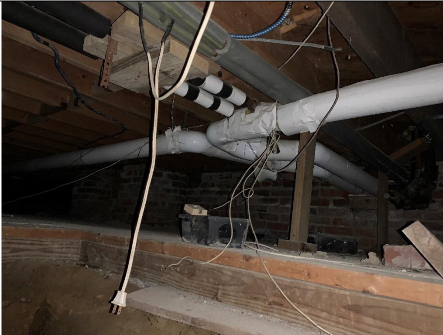
Another View of Non-ACM Fiberglass Insulation on Piping in Basement
