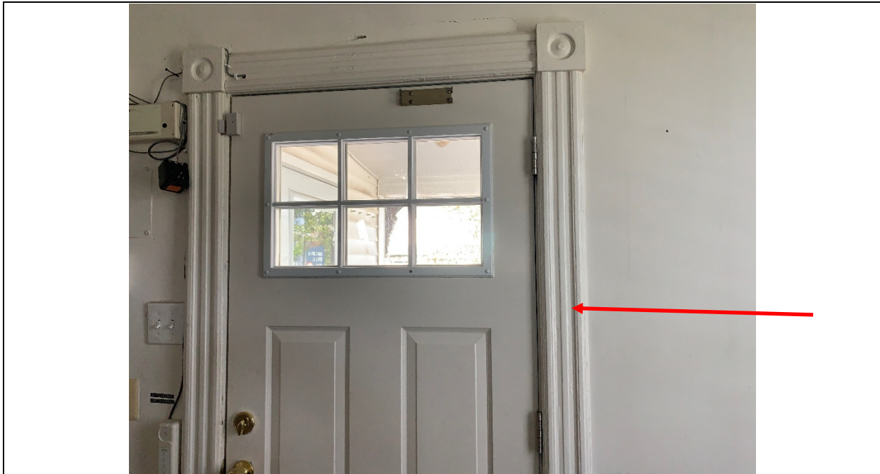
LBP-1: Lead-Based Paint on Living Room Door Casing
