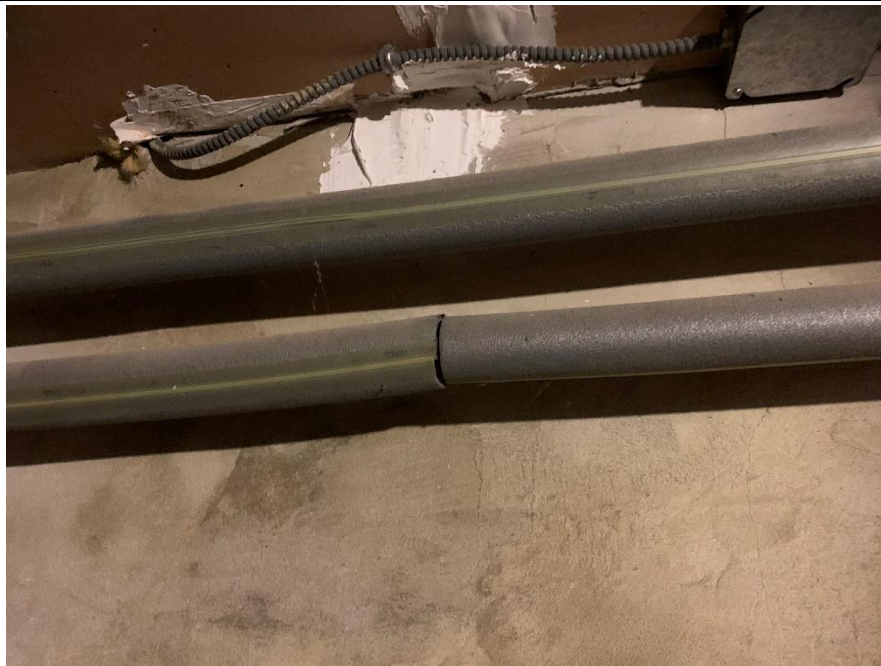
Non-ACM Foam Insulation on Piping in Basement
