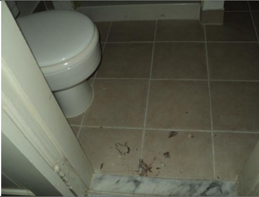
Homogeneous Material No. 13 – Non-ACM Creamish White CT with Cream Grout and White Setting Base located in the Bathroom on the 3 rd Floor
