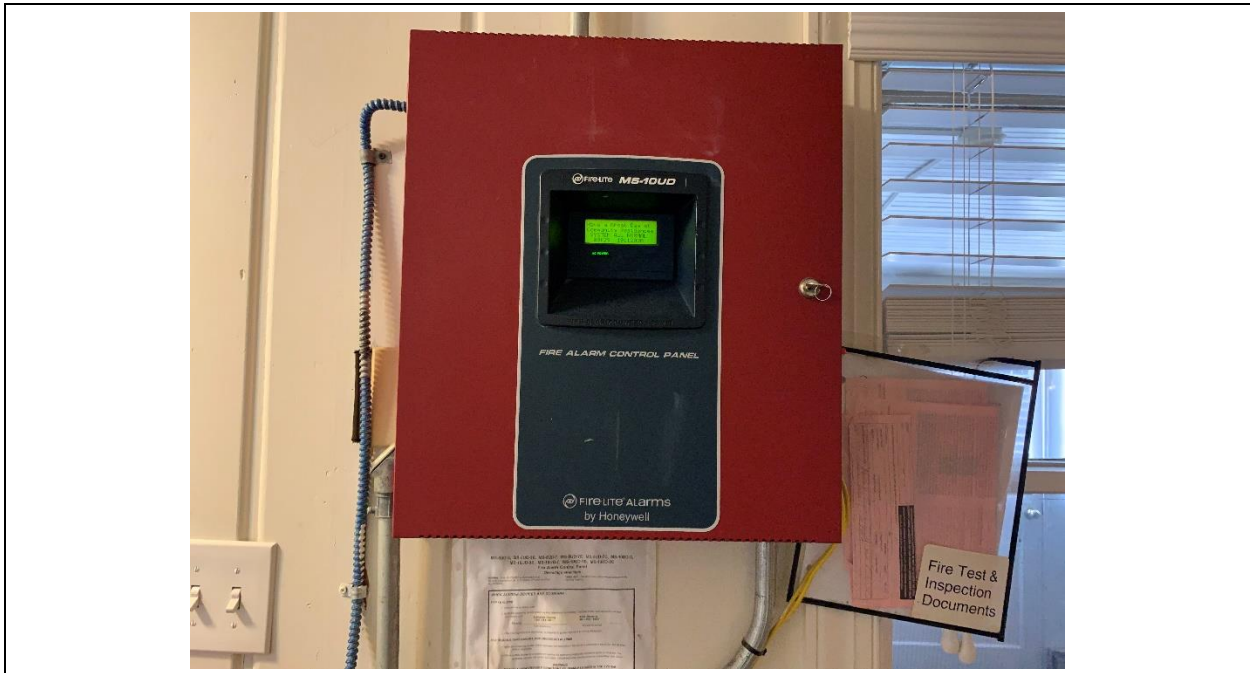
Fire Alarm System in the Office Area of the Subject Property
