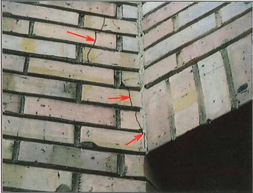
23 - Brick veneer stress cracking
