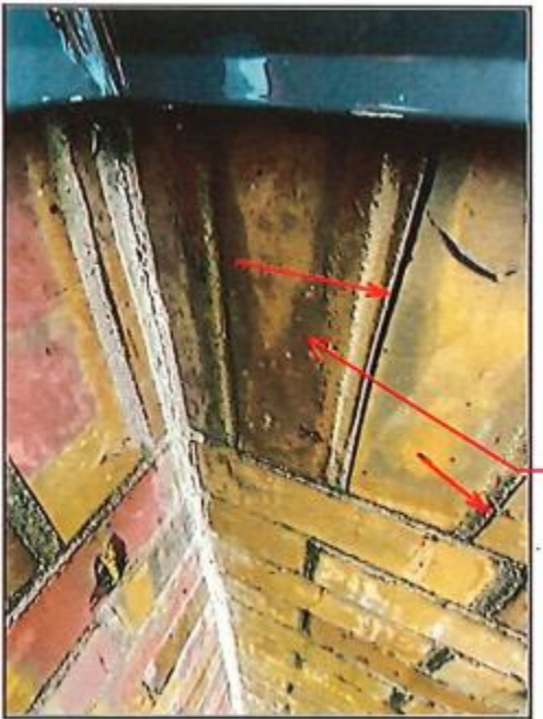
24 - Typical brick joint mortar separation
