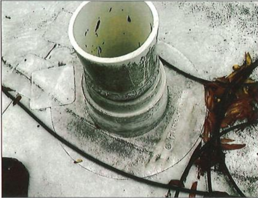
41 - Typical roof penetration boot without clamp
