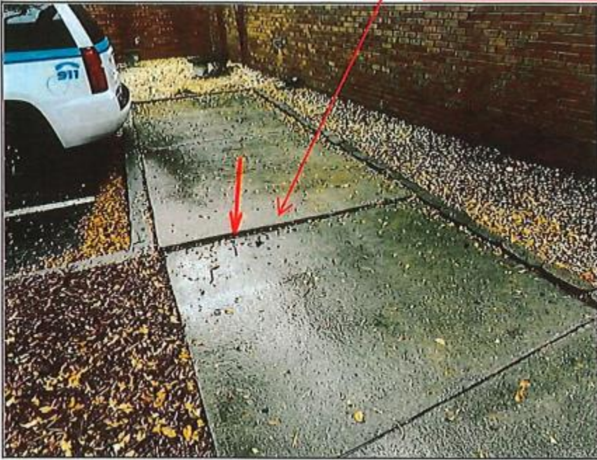
15 - Concrete sidewalk displacement
