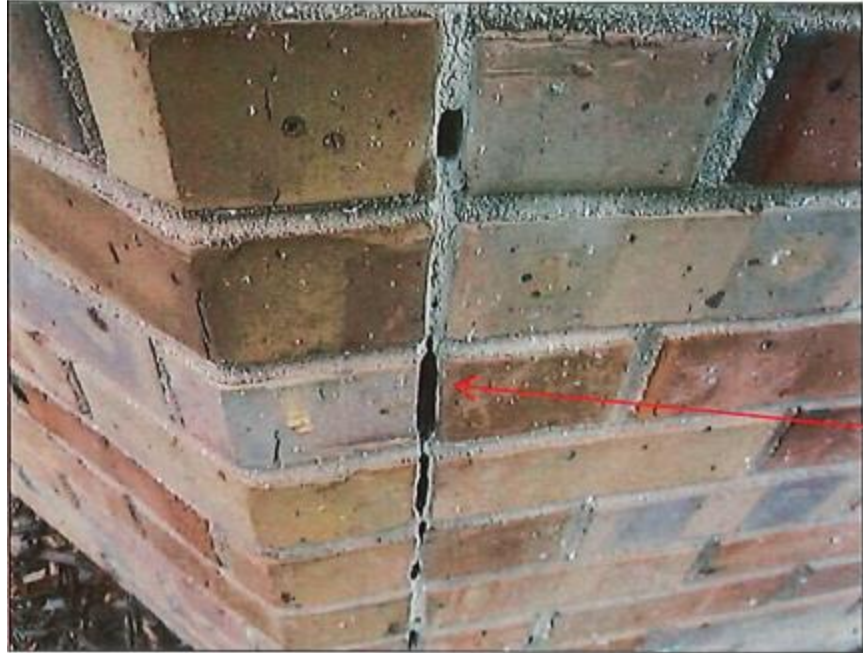
19 - Typical control joint cohesive failure
