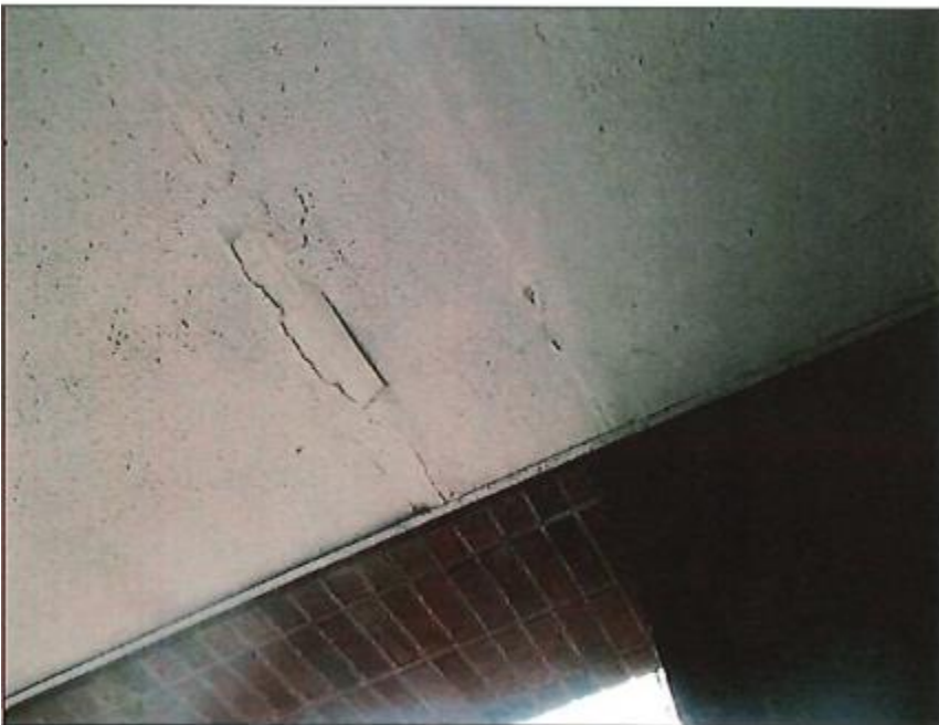
34 - Entry area soffit finish delamination
