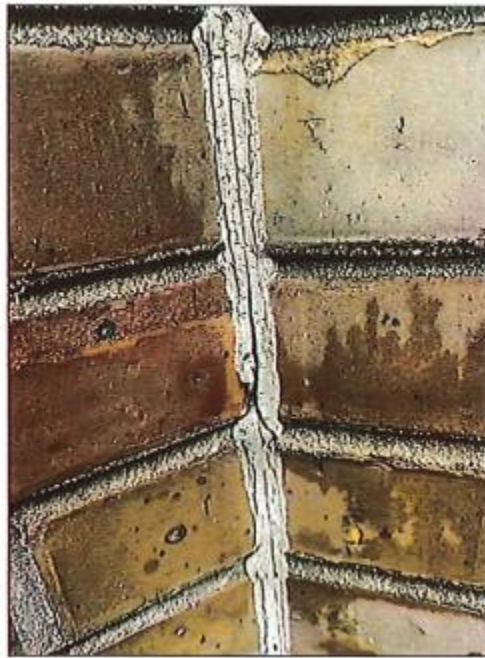
20 - Typical cohesive failure in brick veneer joint
