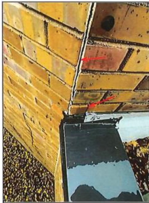
44 - Roof Level; brick corner joint failures
