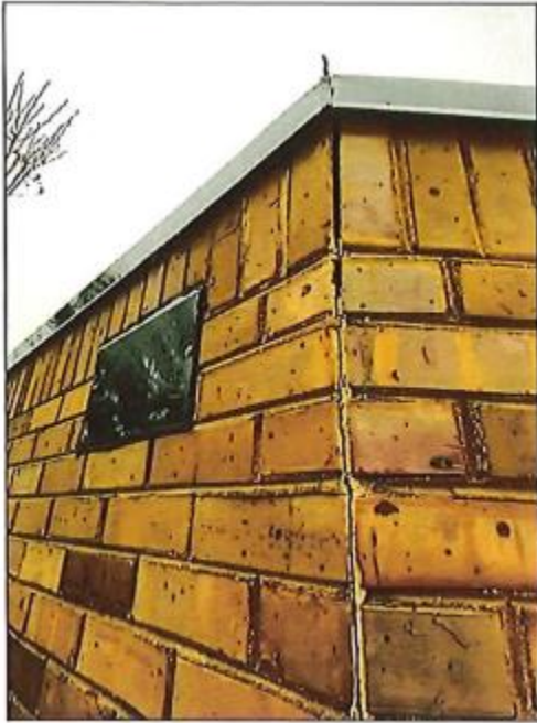
45 - Roof Level; brick corner joint failure
