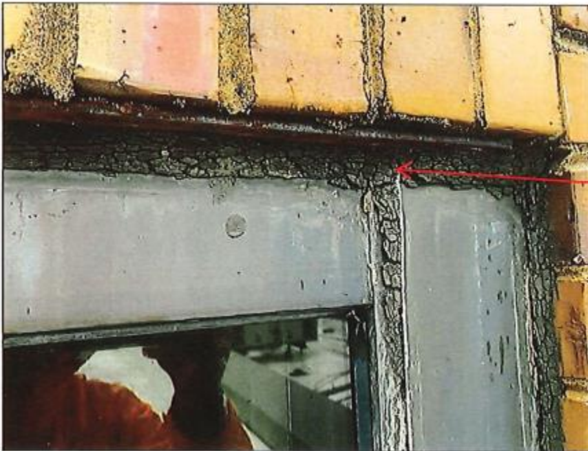
50 - Roof Level; clerestory window sealant cracking
