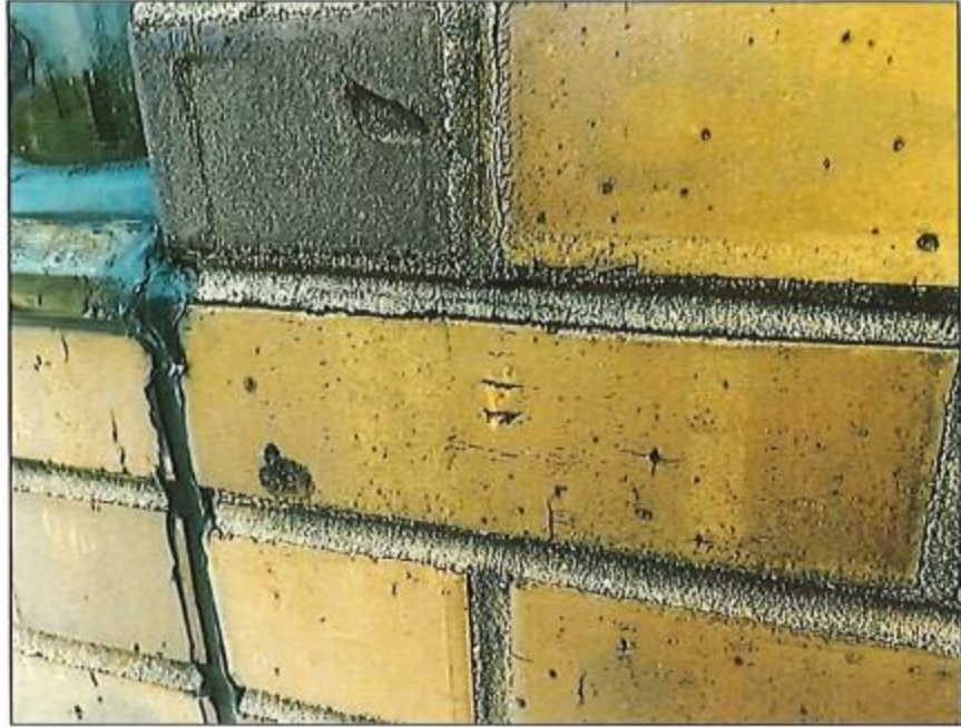
47 - Roof Level; mortar joint separation
