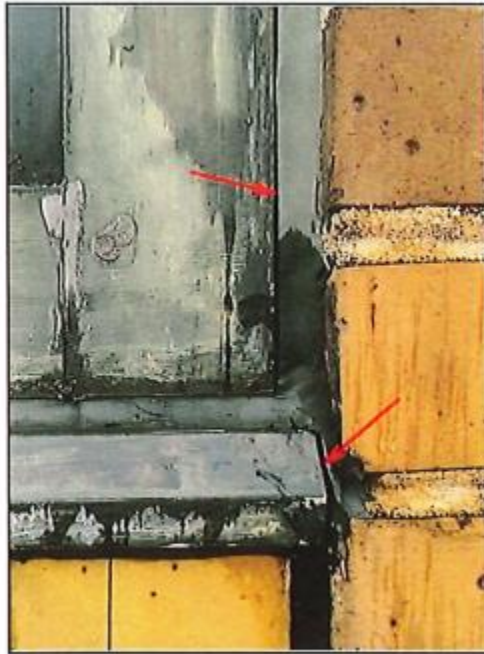
48 - Roof Level; clerestory window sealant adhesive failure
