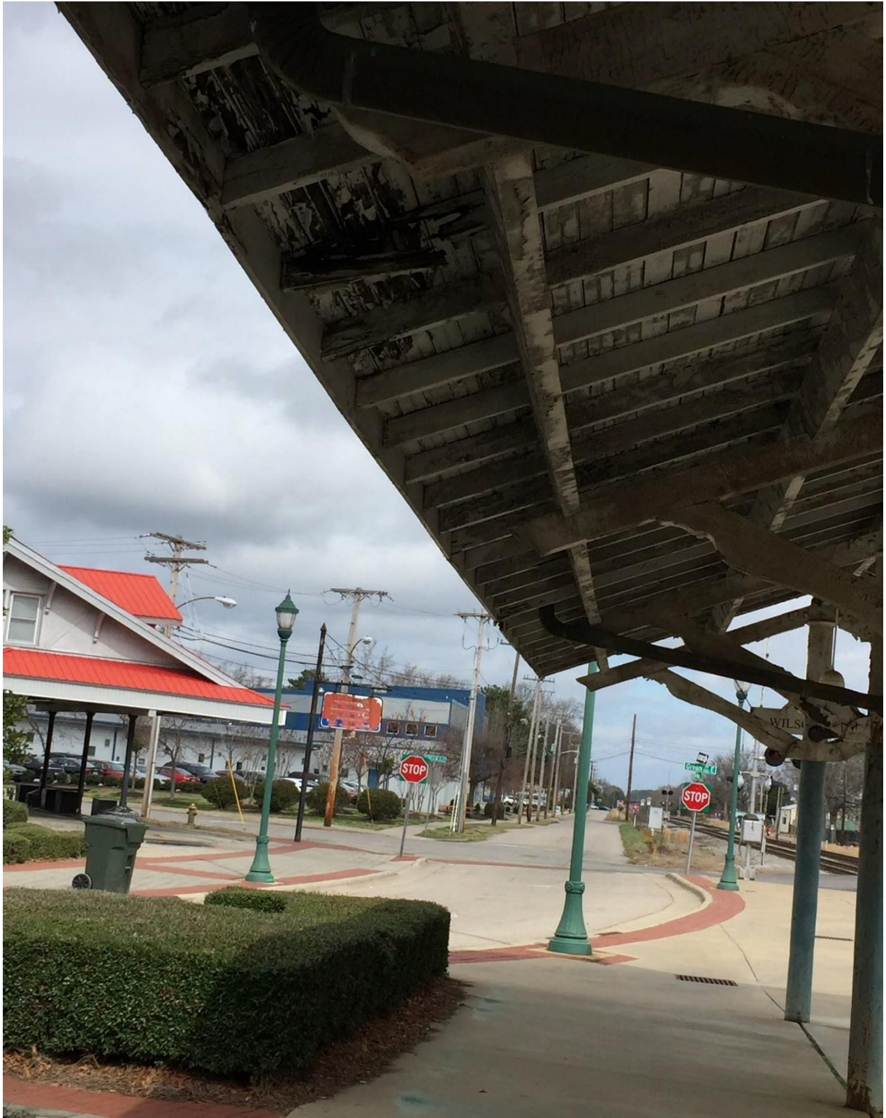
Peeling Paint and Roof Damage
