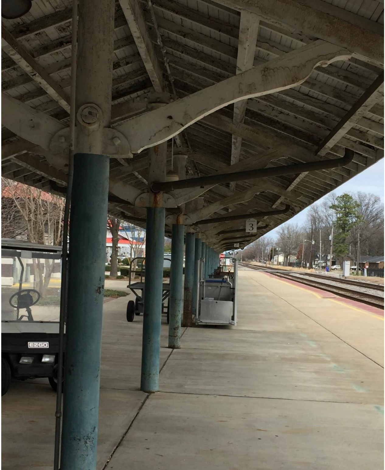
Peeling Paint and Worn Conditions
