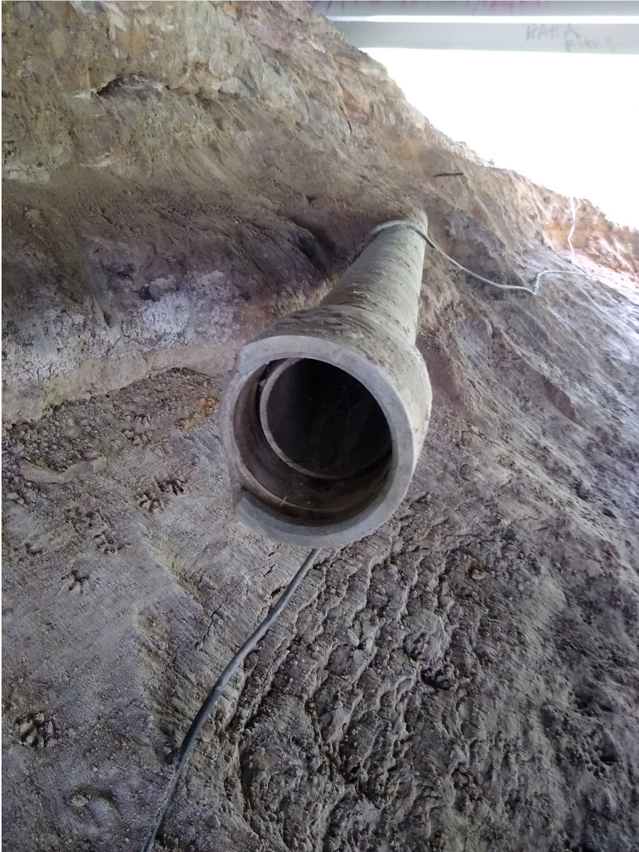
Figure 6 Close-up of broken asbestos concrete pipe at south side of bridge
