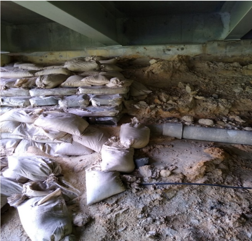
Figure 2 Existing broken pipe under bridge and temp. sandbags to be removed
