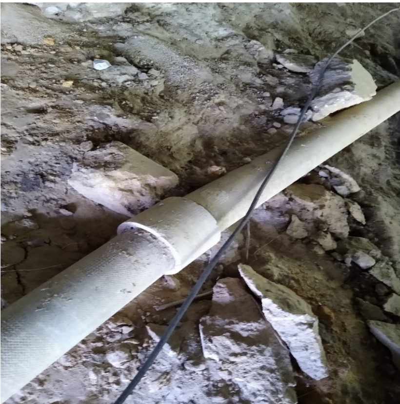
Figure 3 Contractor to be aware of wiring running alongside Asbestos Concrete waterline and refrain from damaging.
