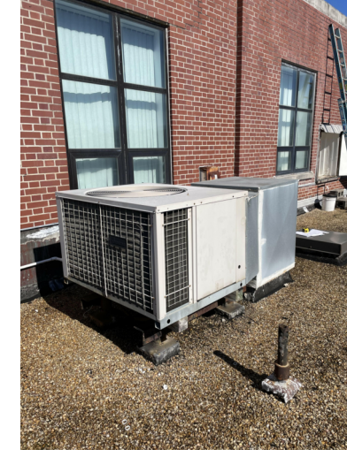
EXISTING HVAC UNIT 11
