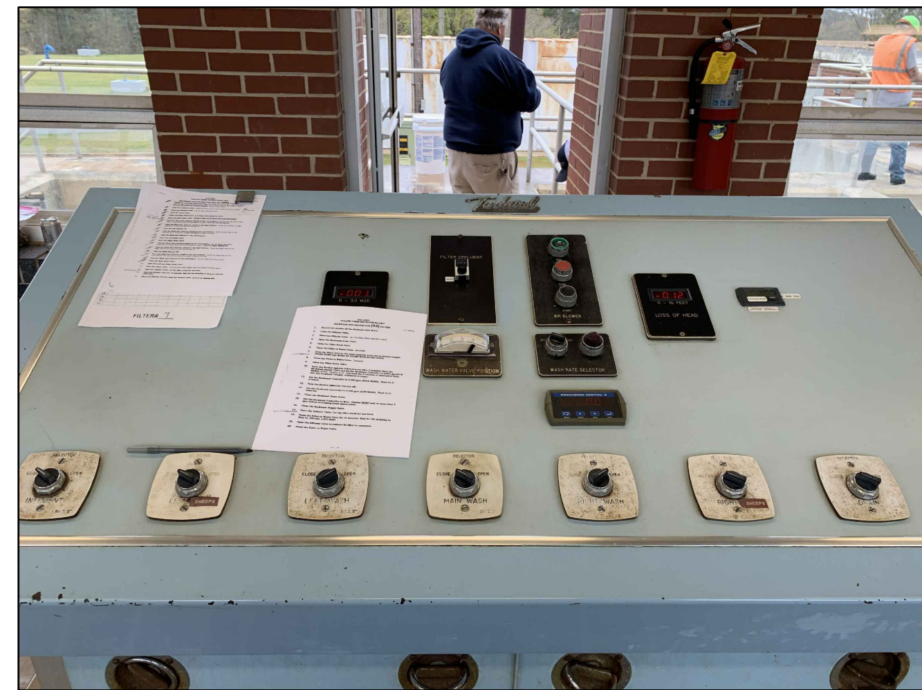
FILTER OPERATING CONSOLE DIGITAL DISPLAY
