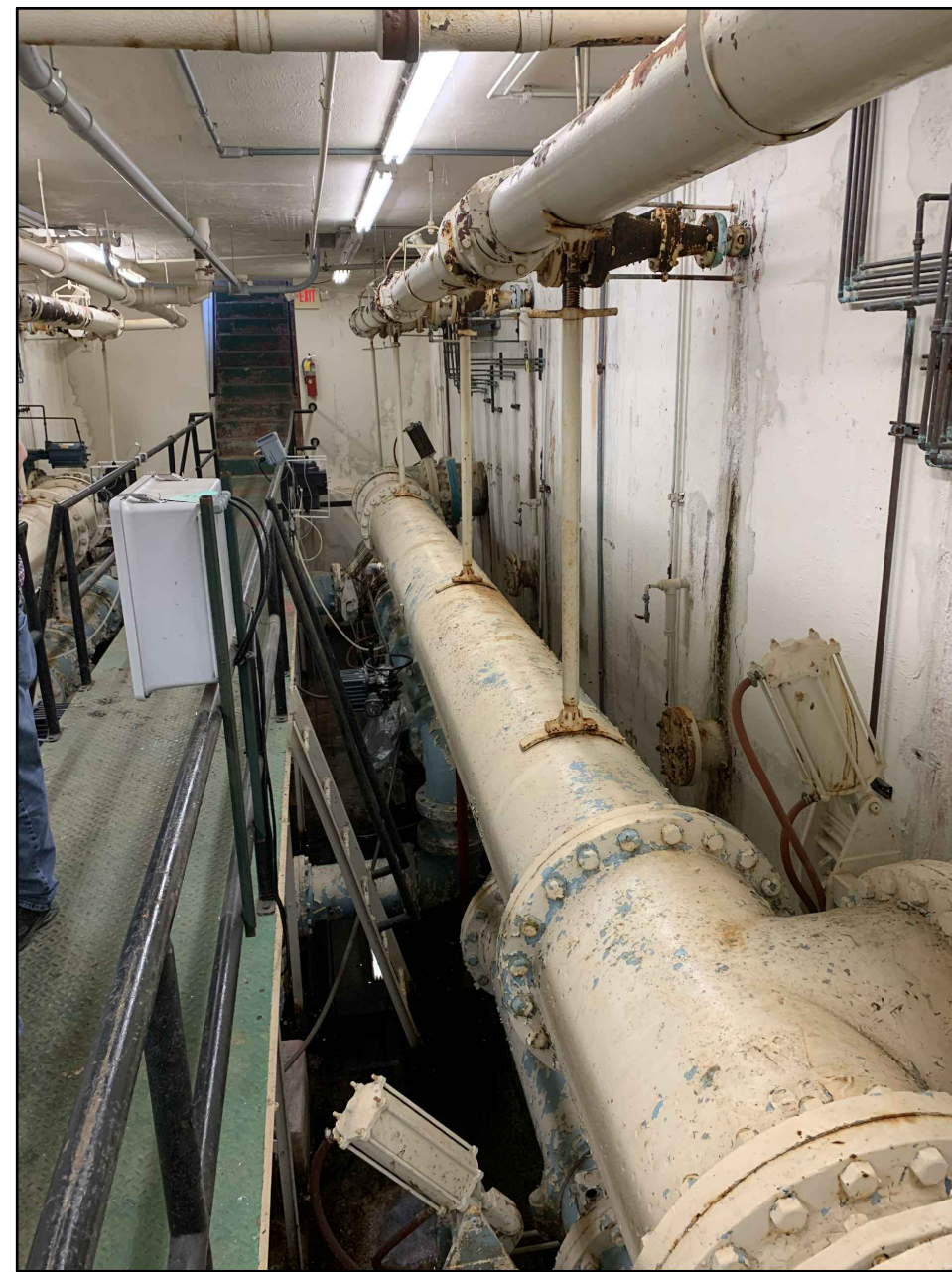
SURFACE SWEEP PIPING AND SUPPORTS
