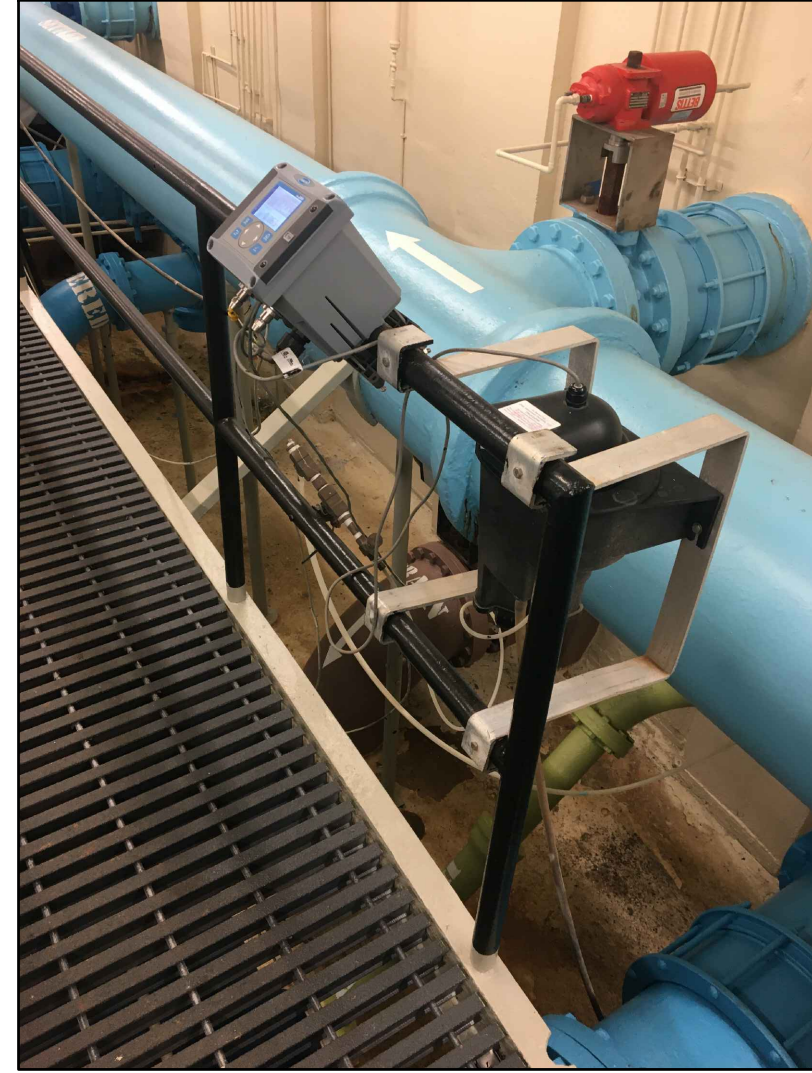
TURBIDITY METER & CONTROLLER
