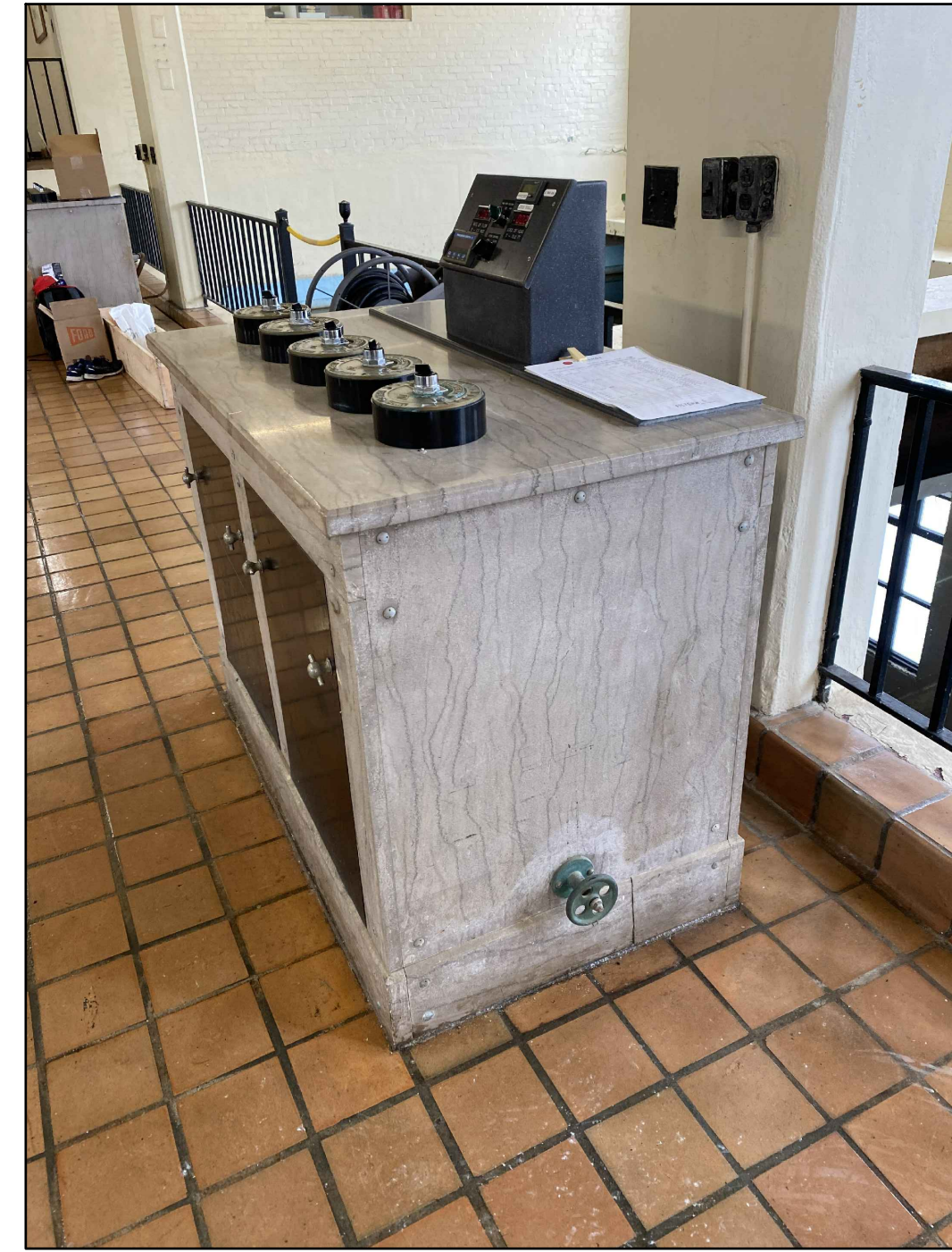
FILTER OPERATING CONSOLE
