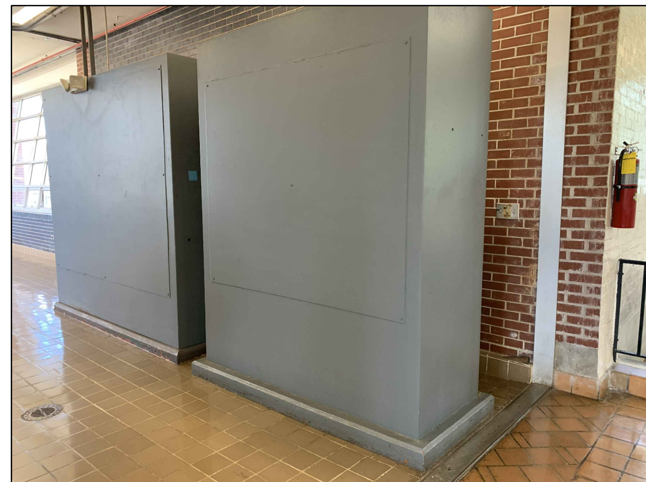
EMPTY ELECTRICAL CABINETS AND CONCRETE PADS
