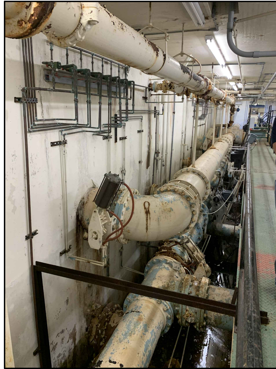
PIPE GALLERY & HYDRAULIC ACTUATOR PIPING
