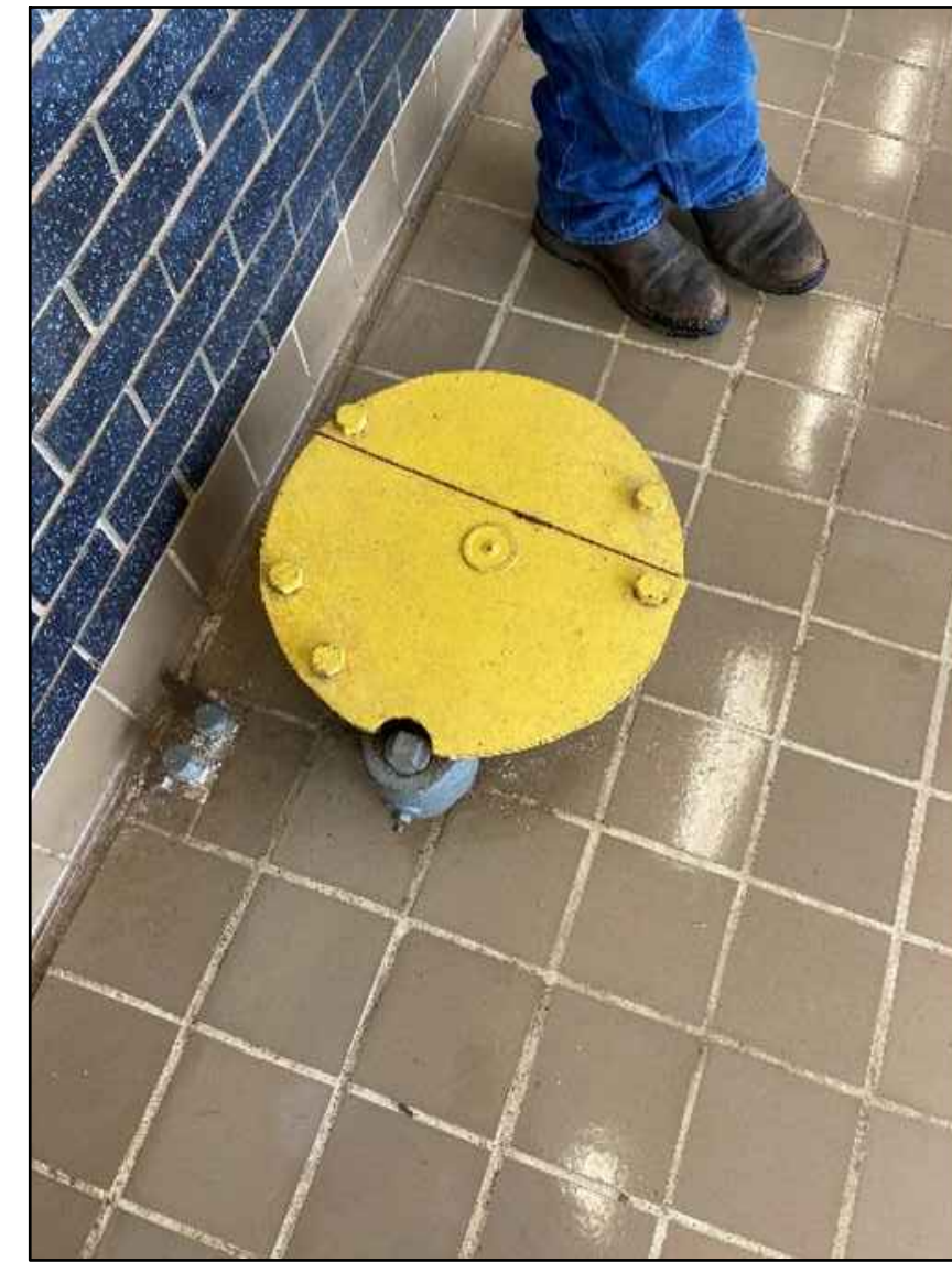
FLOAT WELL IN FILTER GALLERY
