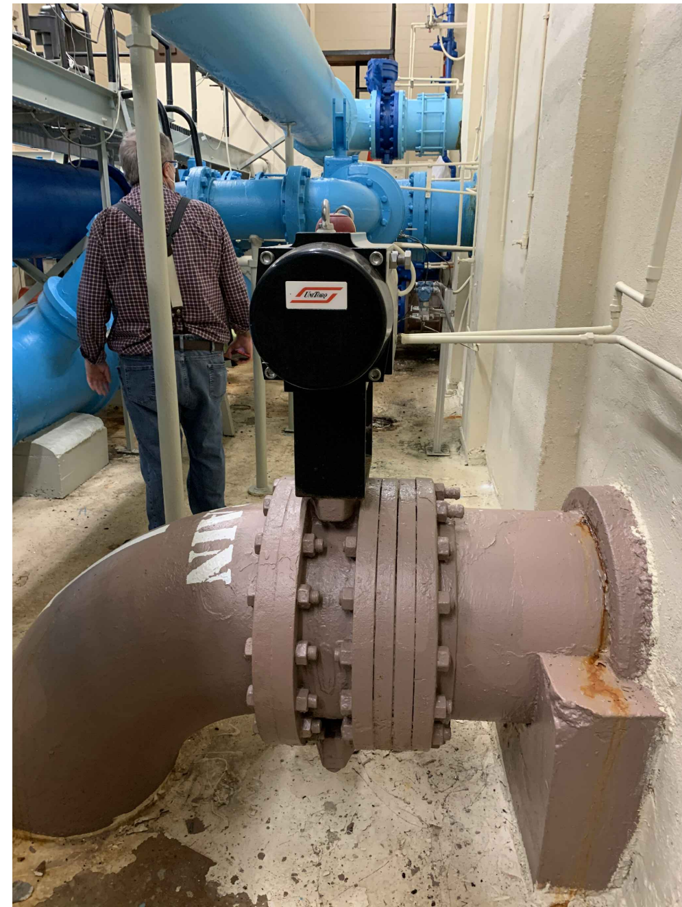
18" WASTE DRAIN VALVE
