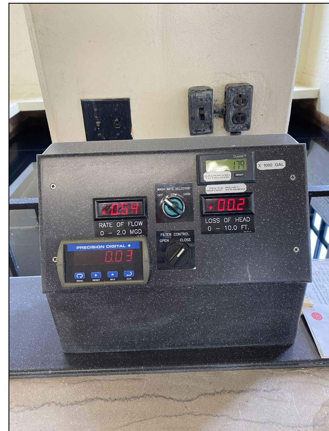
EXISTING OPERATING CONSOLE DIGITAL DISPLAY
