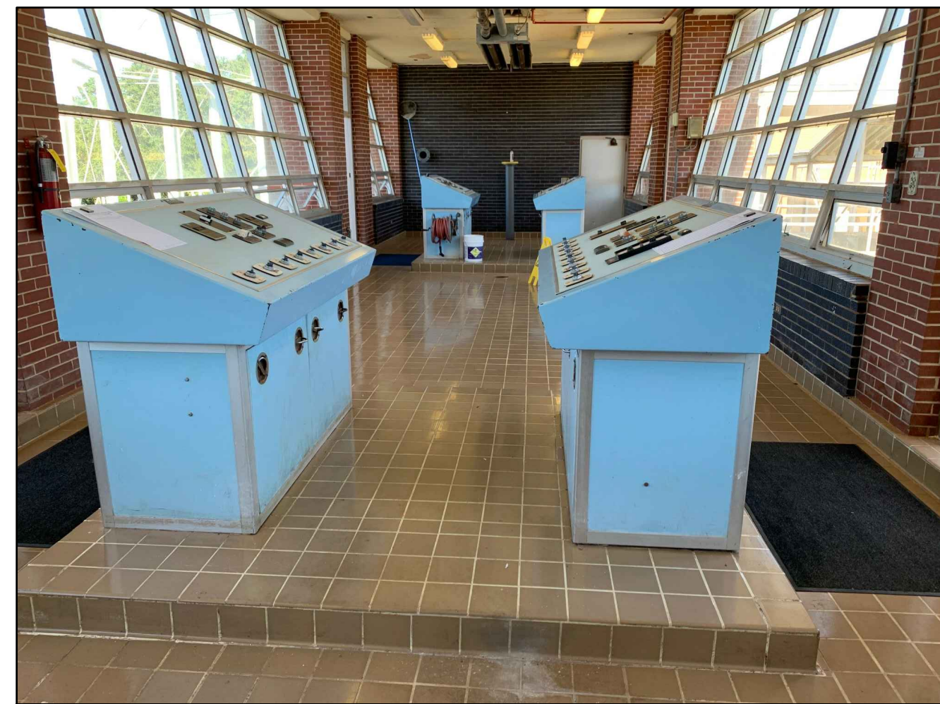
FILTER OPERATING CONSOLES
