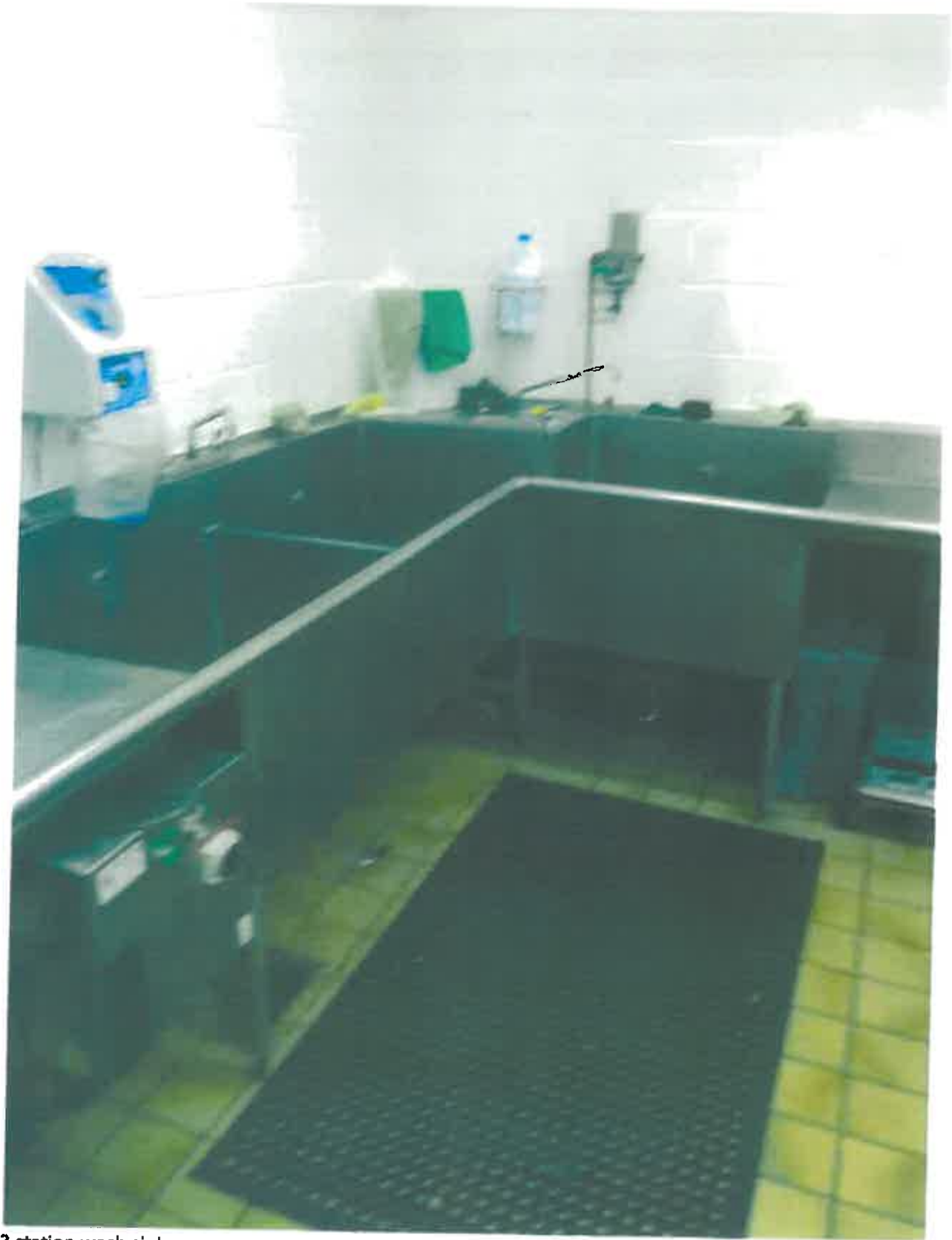
3 station wash sinks
