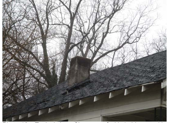
Photo 16 – Typical view of house roof with 1 chimney with tar that are presumed positive for asbestos
