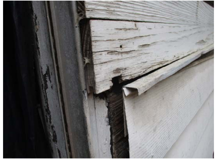
Photo 14 – White filler material in wooden siding in the back door area
