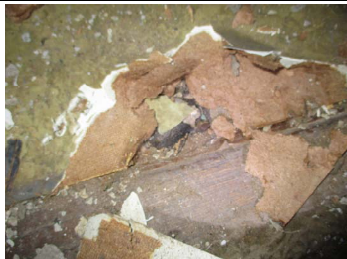
Photo 5 – Tan rock fissure pattern roll vinyl floor over 4 layers of vinyl floors & adhesives in the dining room
