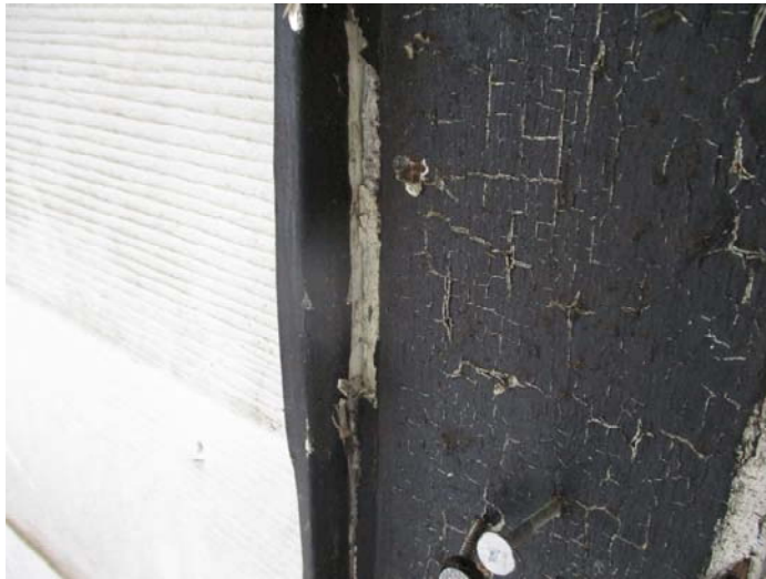
Photo 13 – Hard white caulk on wooden window & door casings
