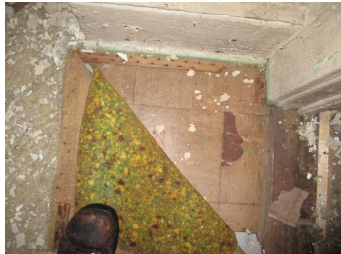
Photo 3 – 9"x9" brown streaked floor tile & mastic under carpet in the living room & hallway
