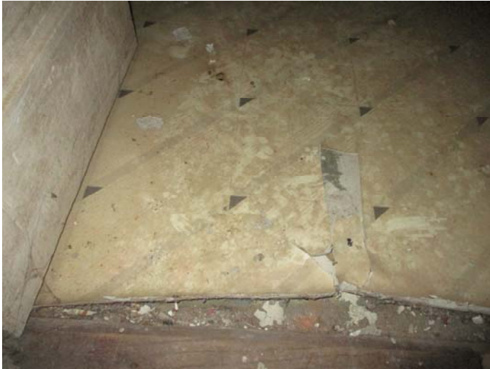
Photo 7 – Tan with gray stripes roll vinyl floor with backing & adhesive in the bathroom
