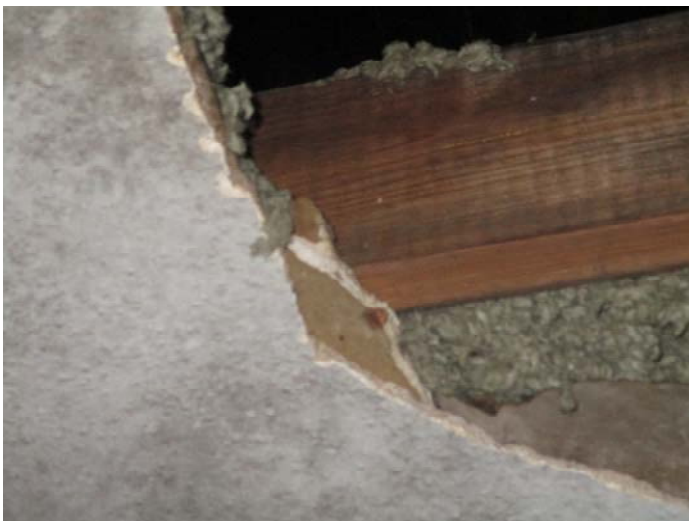
Photo 11 – Unfinished drywall beneath plaster scattered throughout the residence
