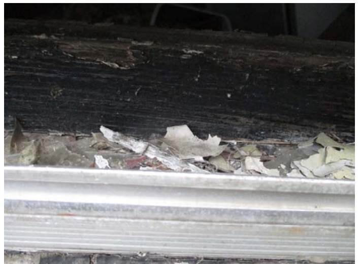
Photo 12 – Wooden window glazing
