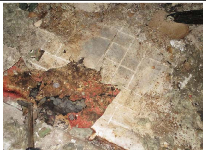
Photo 6 – Tan & gray pattern roll vinyl floor over 5 layers of vinyl floors & adhesives in the kitchen
