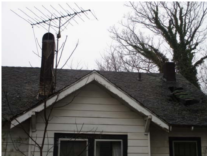
Photo 15 – Typical view of house roof with 2 chimneys with tar that are presumed positive for asbestos
