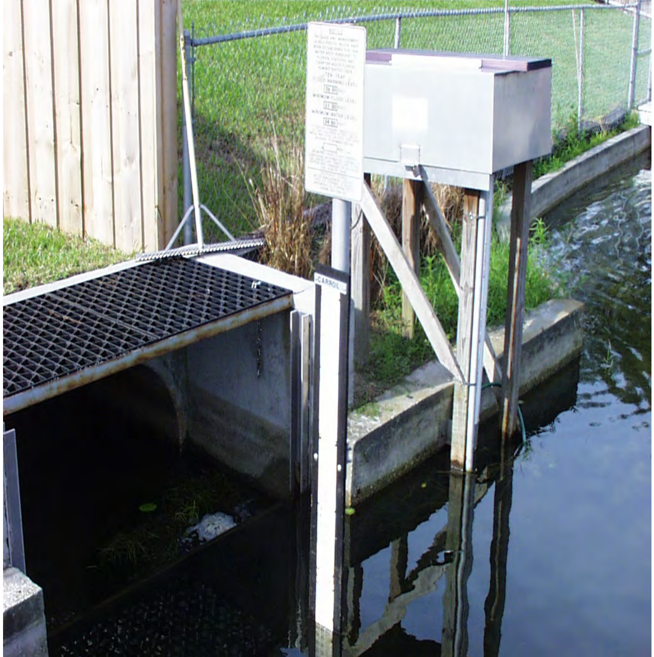
Figure 2: Staff gauge located adjacent to a stilling well and recorder shelter
