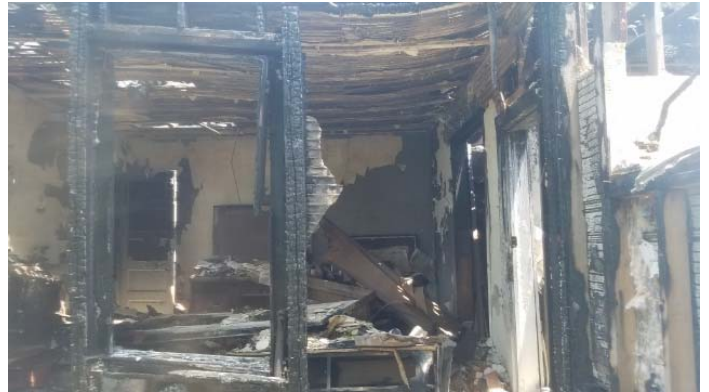
Photo 10 – Exterior view through burnt wall.
