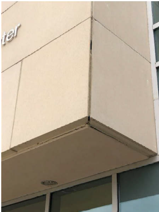
Image 1476: Soffit movement at outside corner, likely evidence of water intrusion.
