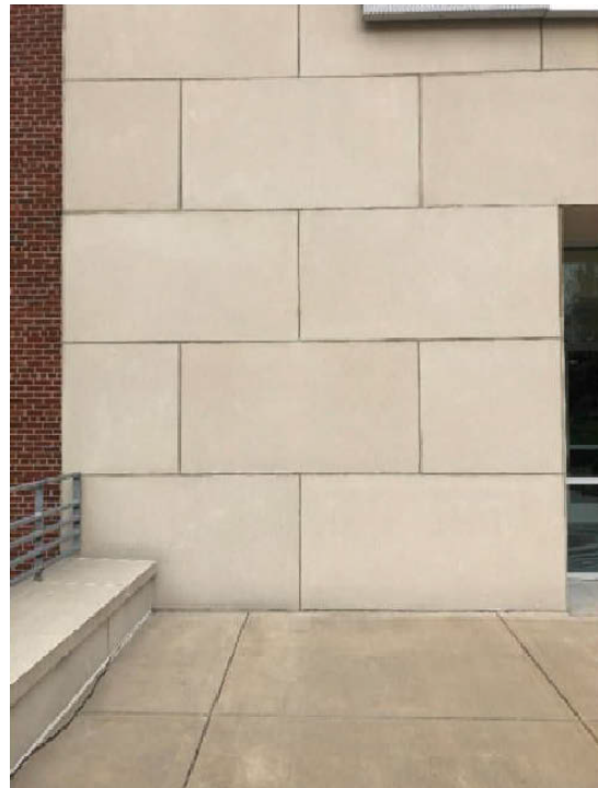
Image 1513: Weeps missing at pavement.
