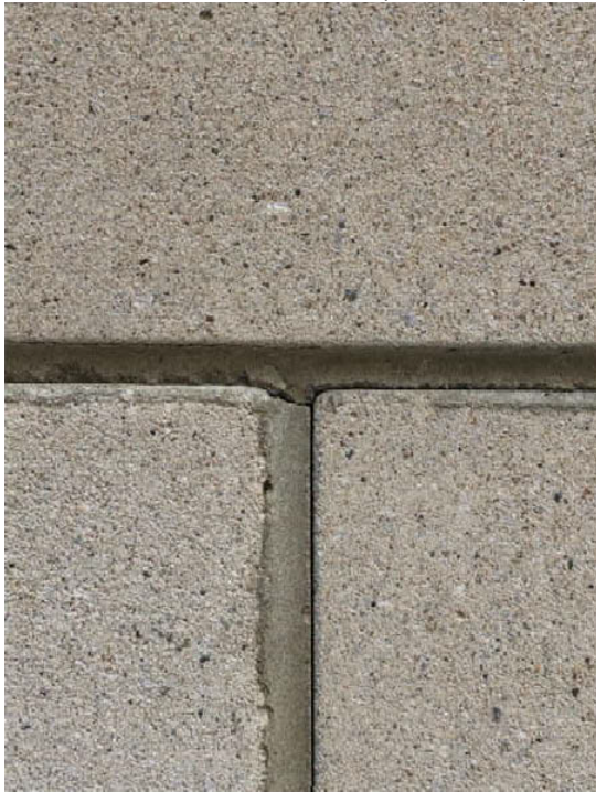
Image 1486: Bond line failure - may be caused by panel movement or shrinkage.
