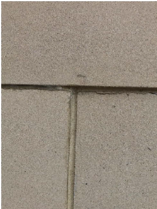
Image 1490: Panels out of plane.
