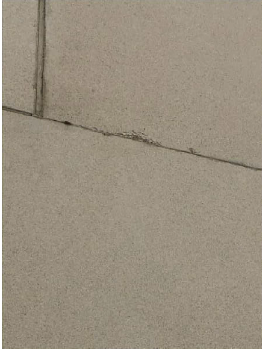
Image 1503: Bed joint too small; spalling.
