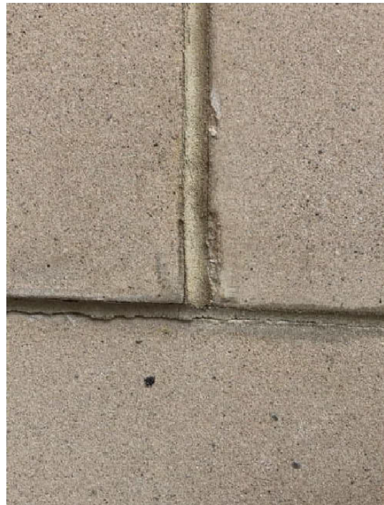
Image 1522: Panels out of plane
