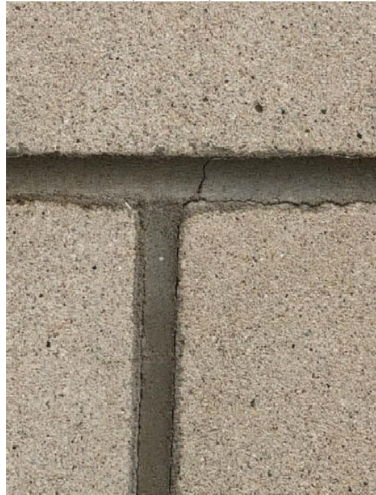
Image 1494: Bond line failure - may be caused by panel movement or shrinkage.
