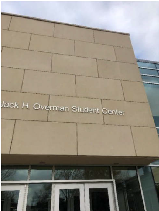
Image 1511: Weeps missing at shelf angles.
