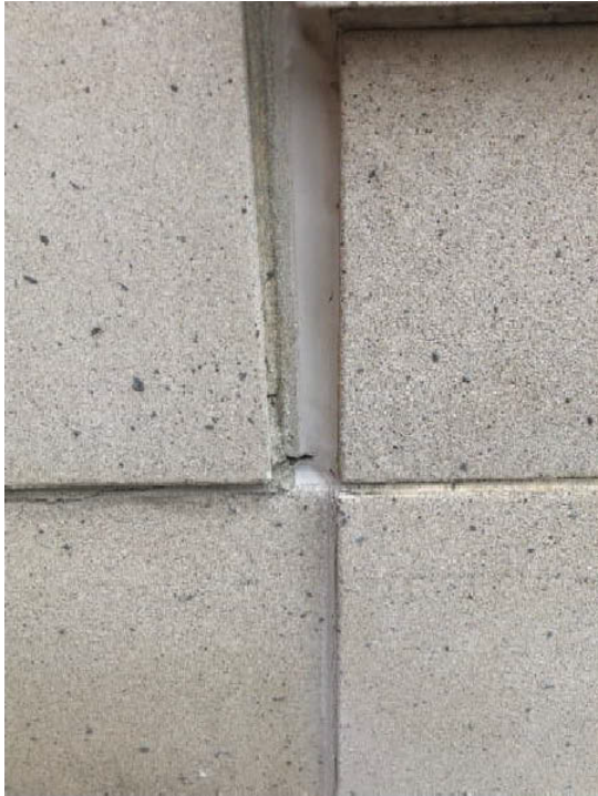
Image 1489: Adhesive and cohesive failure of sealant. (See sealant recommendations below).
